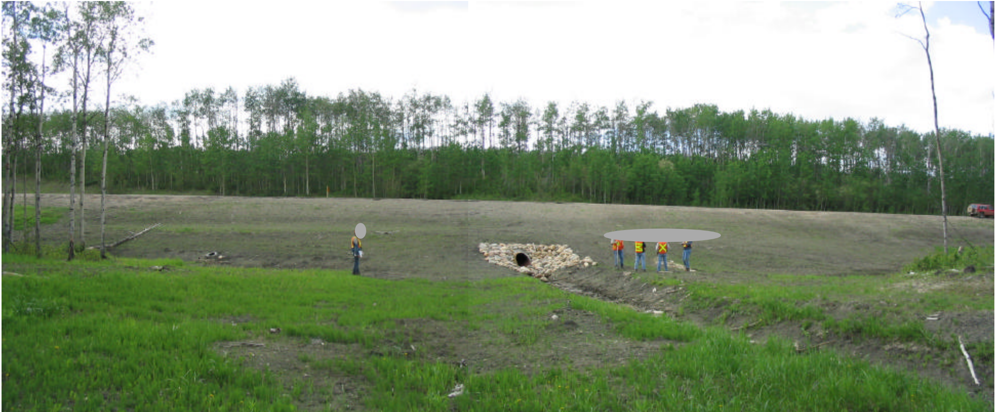
PHOTO 2 LOOKING WEST AT CULVERT OUTLET AND RECENT REPAIR
