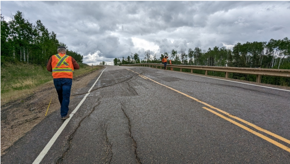
Photo 4: Looking northeast where south scarp crack crosses the highway at the central portion of Site 11.
