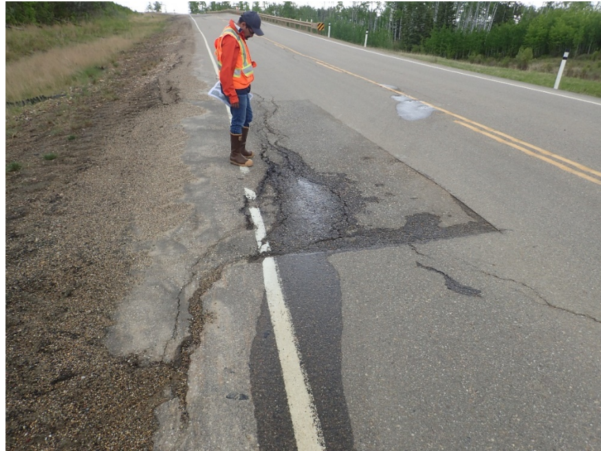
Photo 7: Scarp crack and rutting in a patch located in the SBL.
