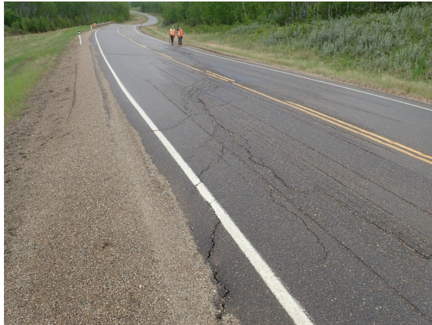
Photo 6 – Looking southwest at north scarp crack.
