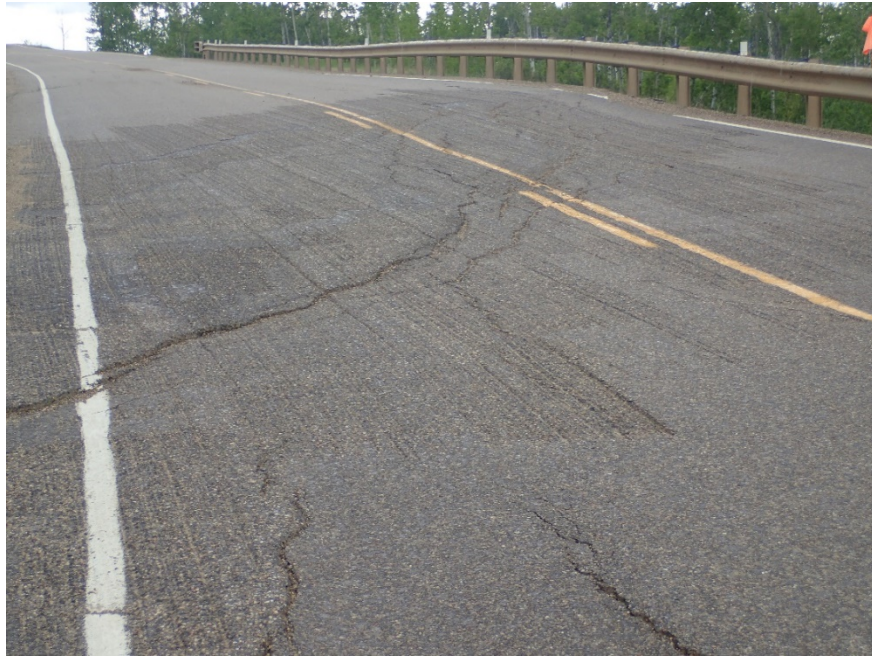
Photo 3 – Looking east at south scarp crack crossing highway (see Photo #4).
