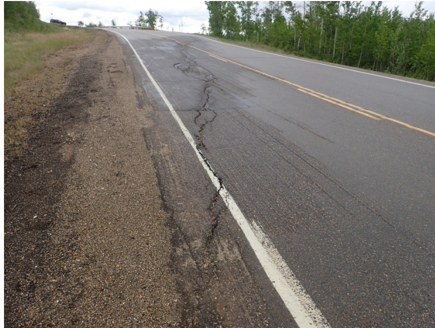
Photo 5 – Looking northeast at north scarp crack.
