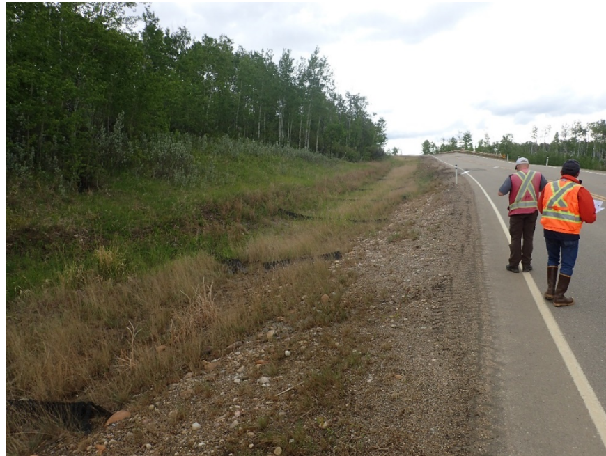
Photo 2 – Looking east at south end of site at installed erosion control measures where previously observed significant gully was regraded.
