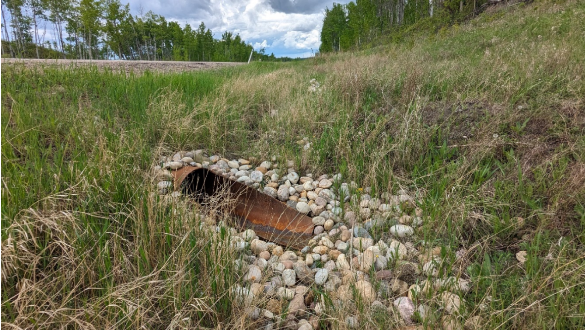
Photo 5: Erosion adjacent to km 20.22 culvert inlet (right side of Photo 5).
