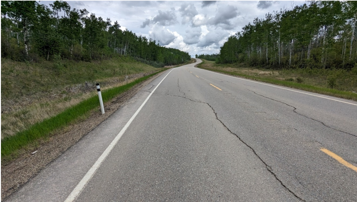
Photo 3 – Looking northeast at potential scarp crack northeast of Photo 3.
