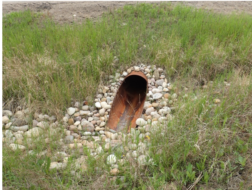
Photo 4 – Looking at inlet of culvert at km 20.22. Note minor rill on the right-hand side of the photo.
