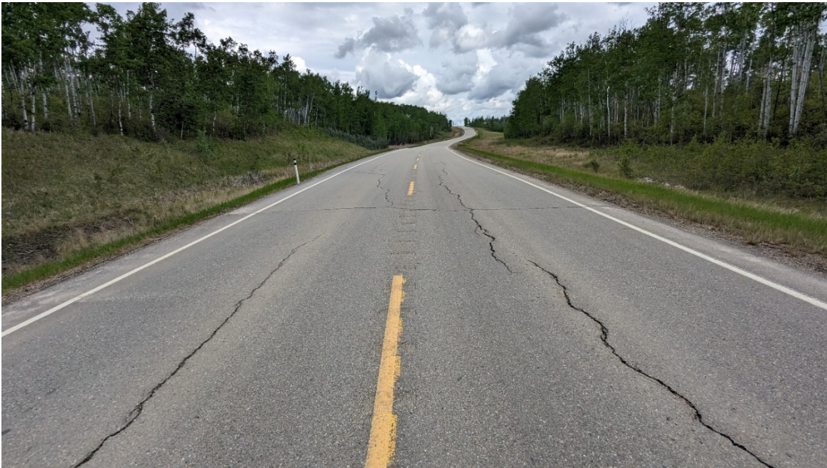
Photo 2 – Looking northeast at cracking that is continuing to surface around km 20.26 (just northeast of the culvert).
