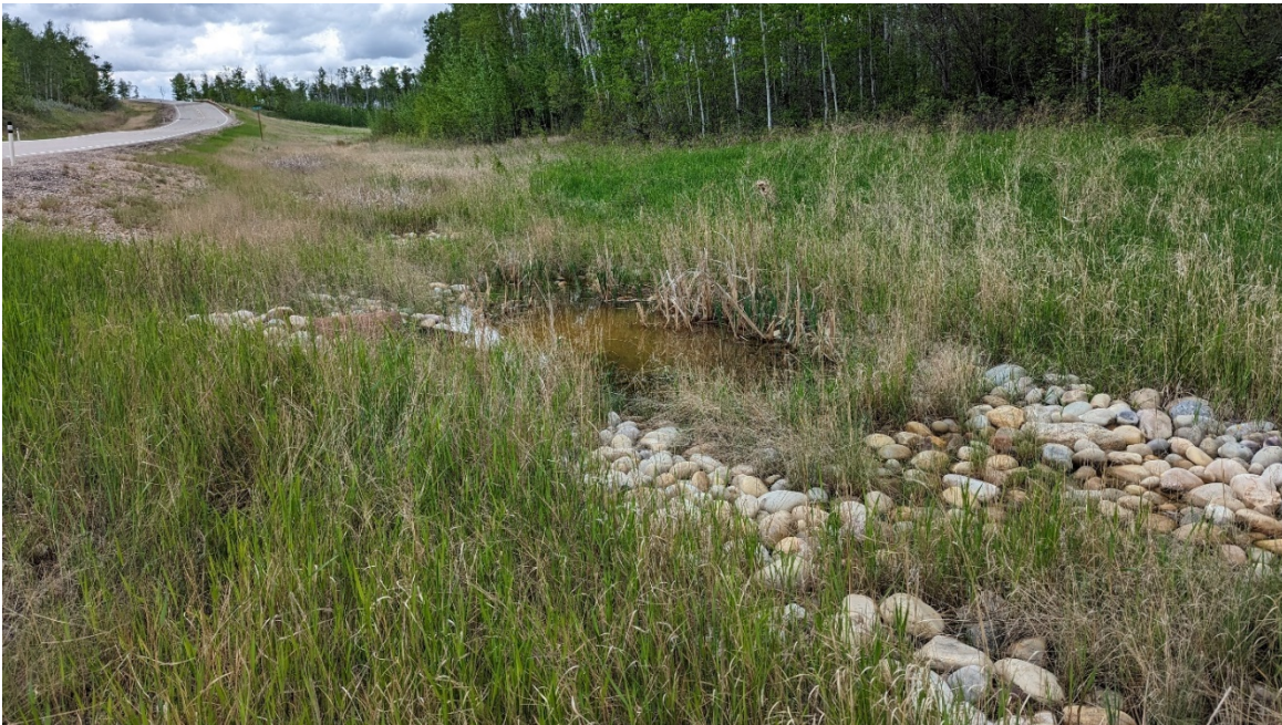
Photo 6: Ponding water in reggraded downslope ditch at the km 20.38 culvert outlet.
