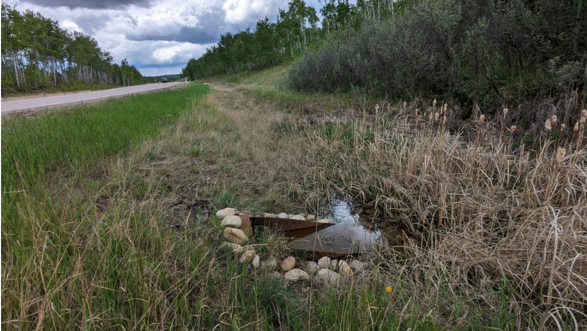
Photo 7: Poor drainage and ponding water at the km 20.38 culvert inlet.
