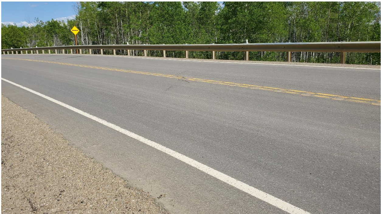
Photo 2 – Looking up-chainage at cracks starting to resurface where main scarp crosses highway.
