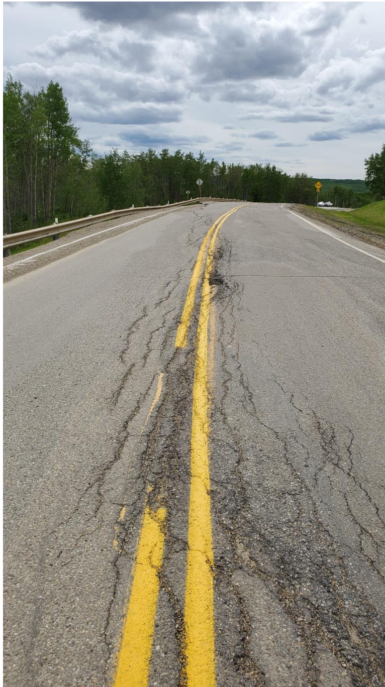
Photo 5 – Looking down-chainage at patch near east end of Site #7 (back towards Photo #6). Note growing width of crack pattern.
