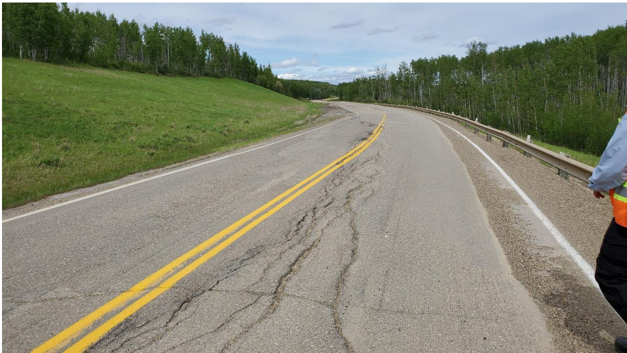
Photo 4 – Looking up-chainage at milling over main scarp crack.
