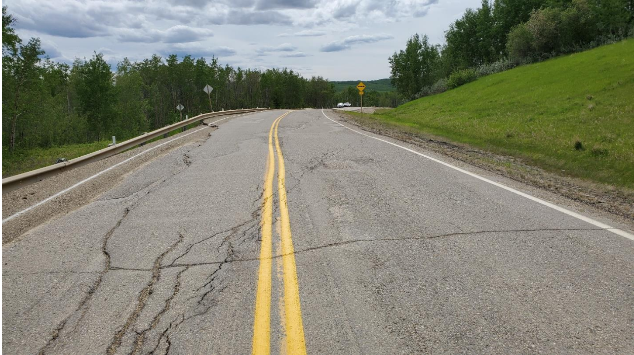
Photo 3 – Looking down chainage at main scarp crack along highway surface.
