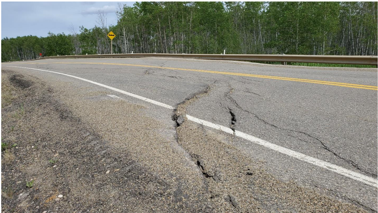
Photo 2 – Looking up-chainage at cracks and milling where main scarp crosses highway.
