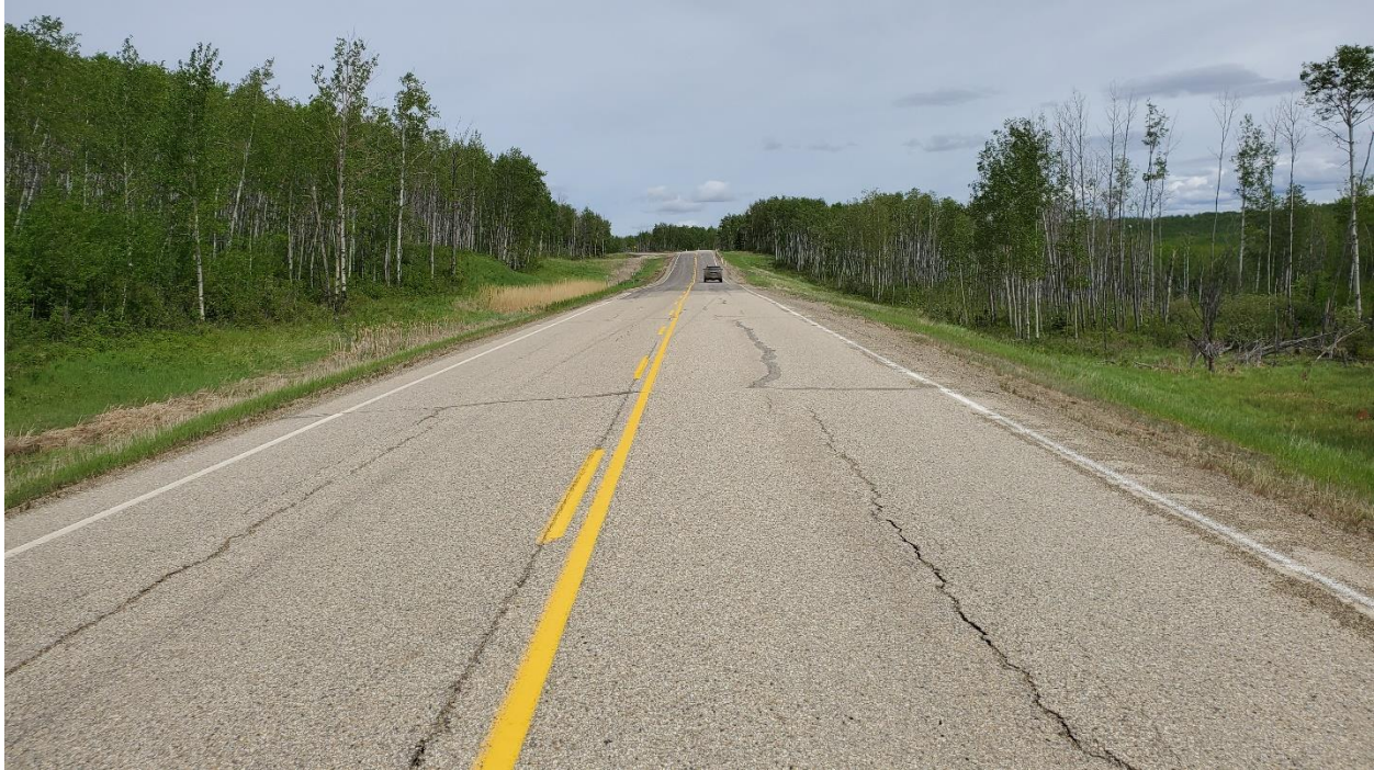
Photo 7, Site 6 – Looking northeast at 2019 patch at km 19.3. There is a noticeable dip about 20 m to 30 m east of the start of the patch.
