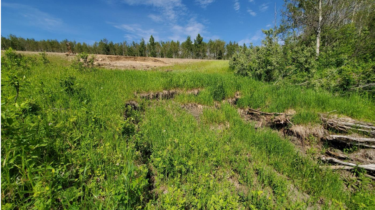
Photo 1, Site 5 (June 24, 2020) – Looking north at slump that has formed at the north edge of the deep landslide depression adjacent to the highway at about km 19.06.
