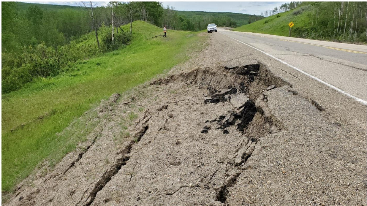
Photo 4, Site 5: Looking west at new slide over the culvert outlet at km 19.07.
