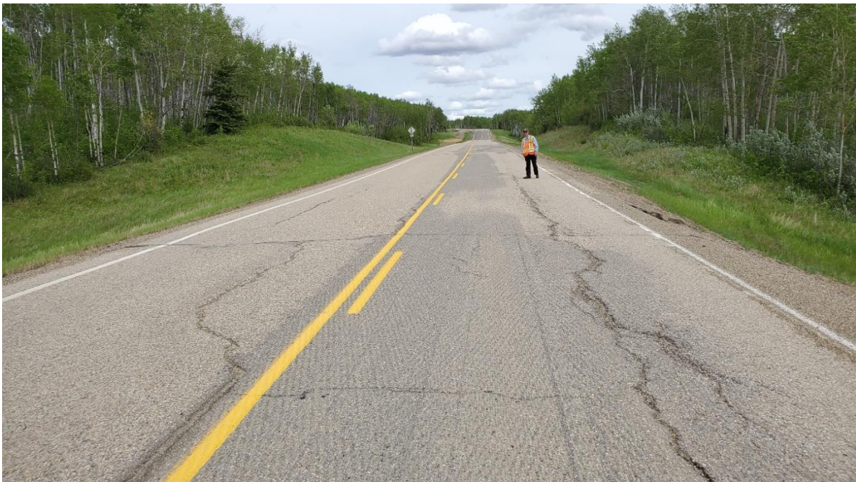
Photo 2, Site 5 – Looking east at crack pattern over culvert outlet at km 19.07 and new slide at edge of right shoulder.
