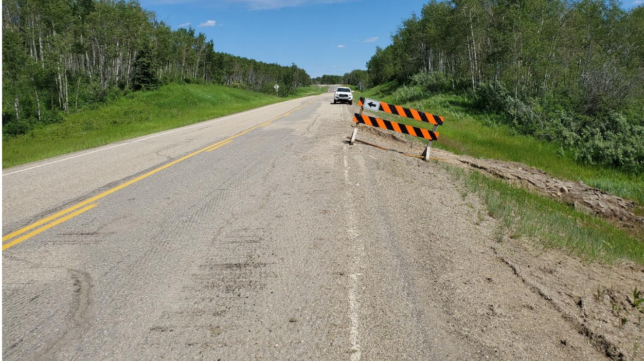
Photo 2, Site 5 (June 24, 2020): Looking east at partially-repaired slide on right shoulder.
