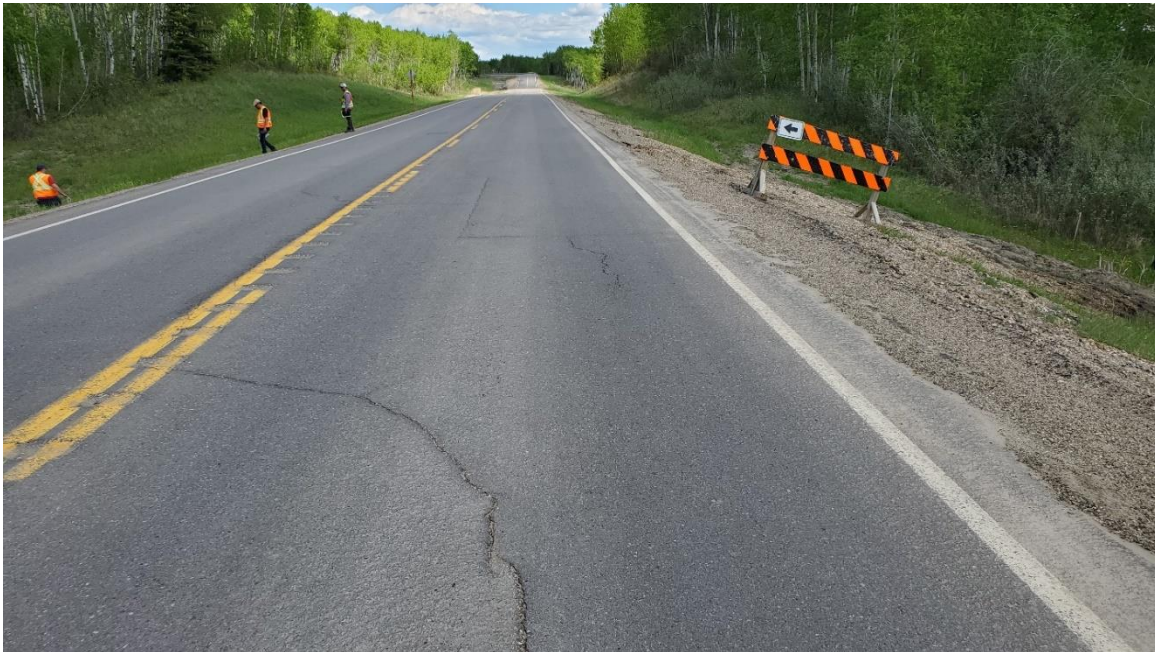
Photo 2, Site 5 – Looking east at crack pattern and slide at edge of right shoulder.
