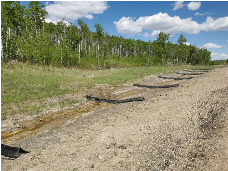
Photo 10, Site 6 – Looking northeast at matting and Georidges installed in the upslope ditch.
