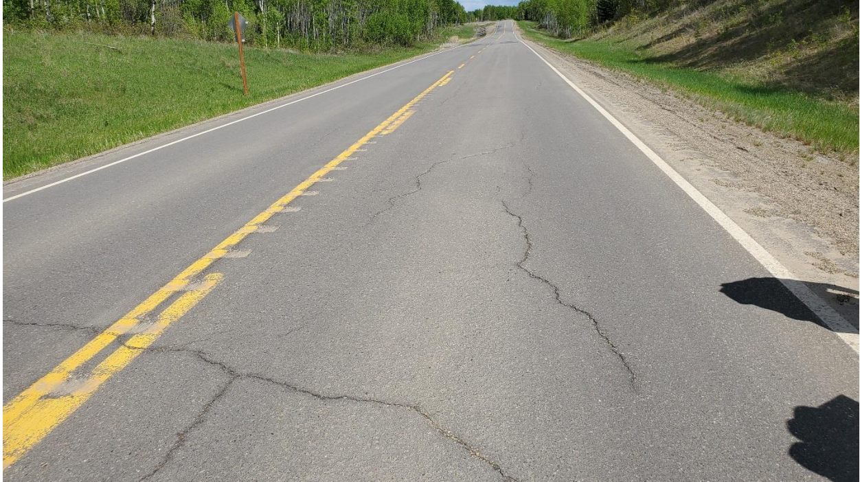
Photo 5, Site 5 – Looking northeast at intermittent cracking between km 19.10 to km 19.13.
