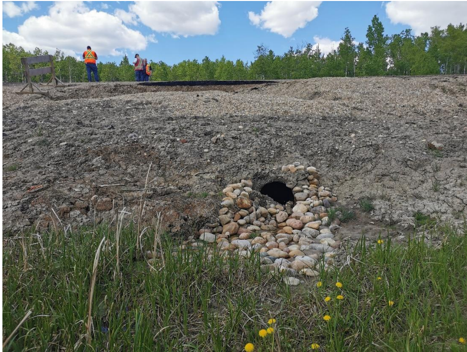
Photo 1, Site 5 – Looking north at slump that has formed at the north edge of the deep landslide depression adjacent to the highway at about km 19.06. Culvert outlet partially blocked with debris.
