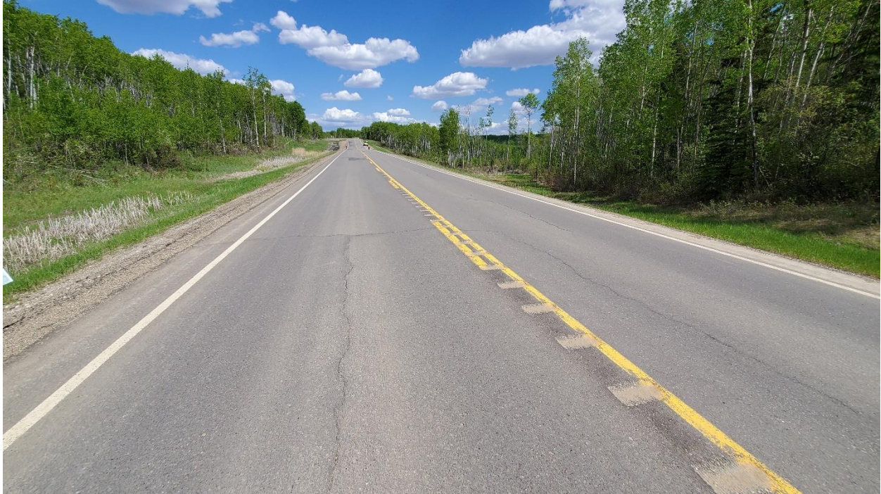
Photo 7, Site 6 – Looking northeast at cracks on the road south of the culvert.
