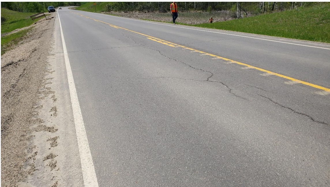
Photo 6, Site 5 – Looking southwest at intermittent cracking between km 19.10 to km 19.13.
