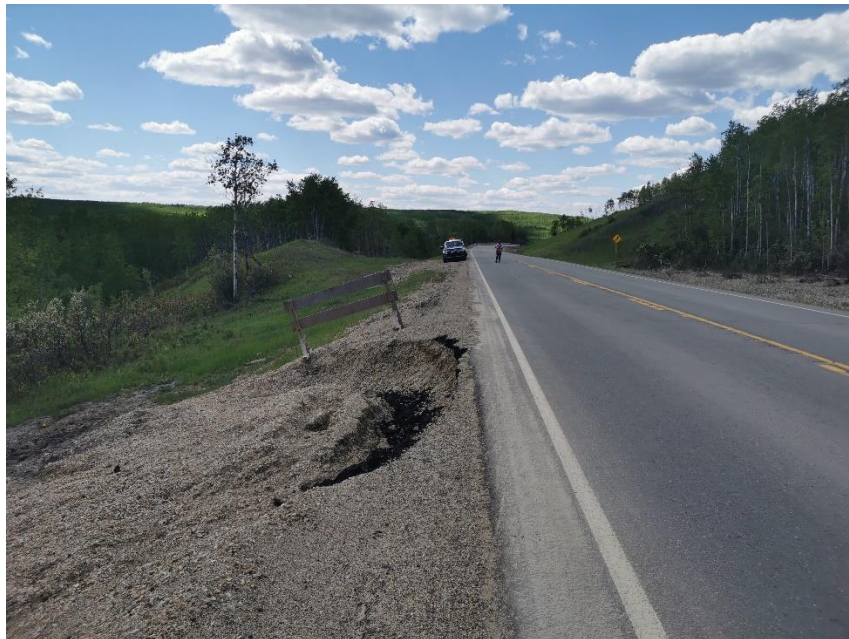
Photo 4, Site 5: Looking west at slide over the culvert outlet at km 19.07.
