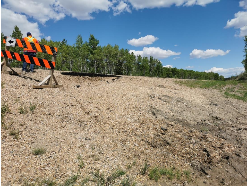
Photo 3: Looking east at the fill placed over the 2020 slump during the highway overlay in 2021.
