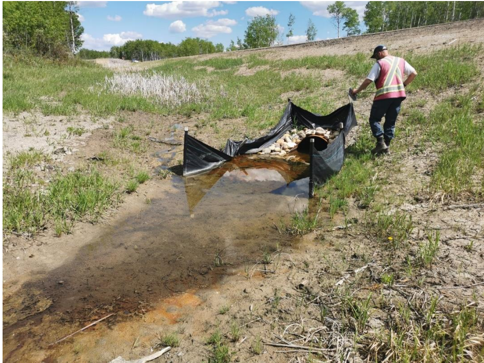
Photo 11, Site 6 – Looking southeast at inlet of new culvert that has pooled water because it is not draining.
