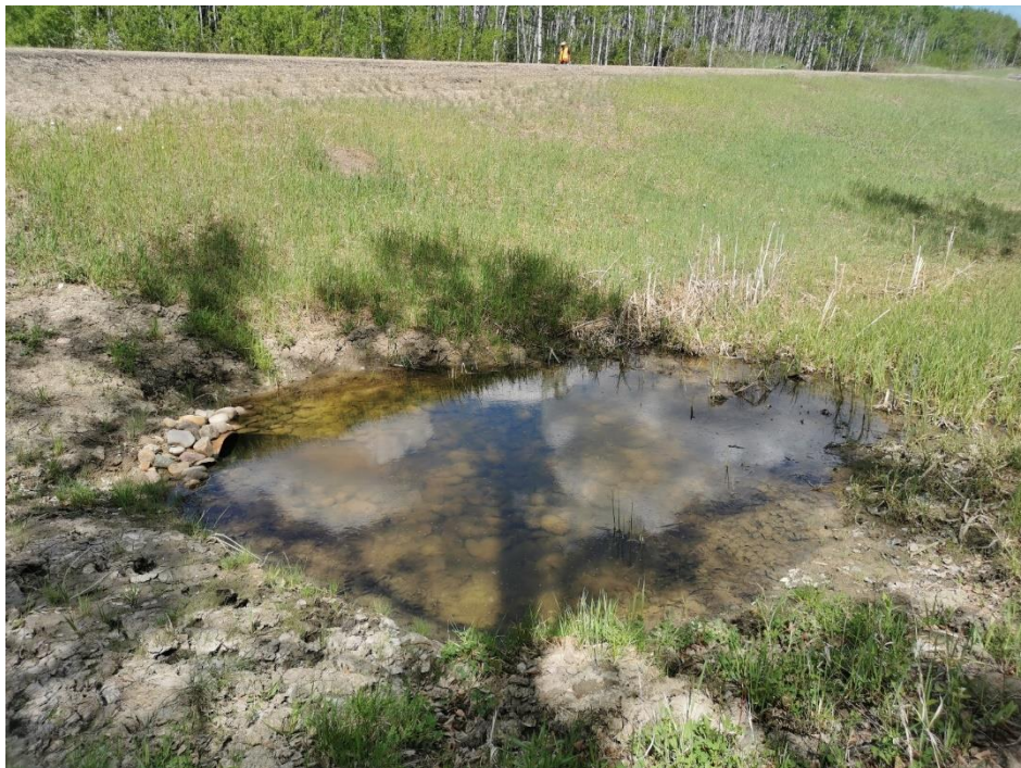
Photo 12, Site 6 – Looking northeast at new culvert outlet that has pooled water because it is not draining.
