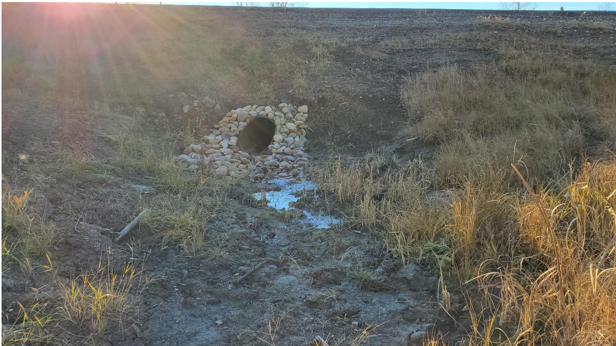
Photo 12 (Oct. 28) – New culvert inlet. Note that inlet seems a bit high.
