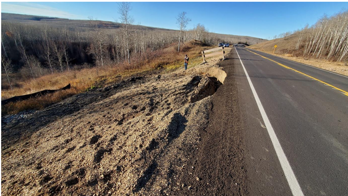
Photo 4 (Oct. 28) – Looking east at slump.
