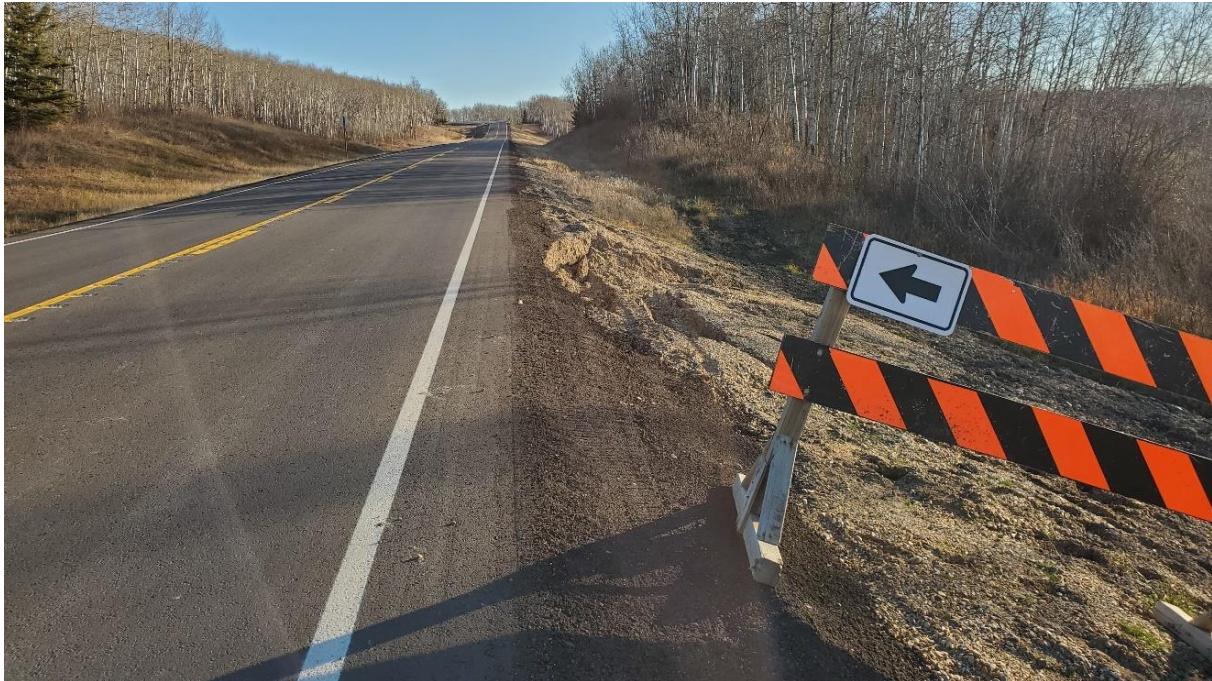
Photo 3 (Oct. 28) – Looking west at crest of slump
