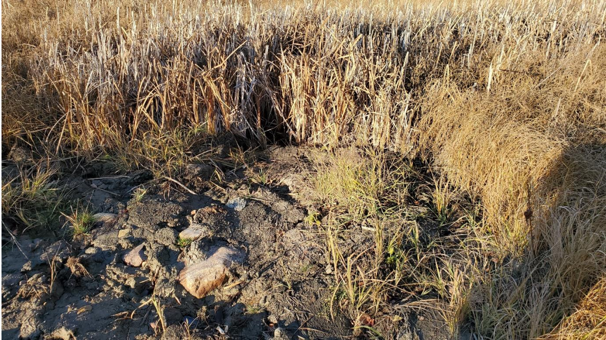
Photo 13 (Oct. 28) – Mound of material upstream/upslope of the culvert inlet blocking drainage from the slough.
