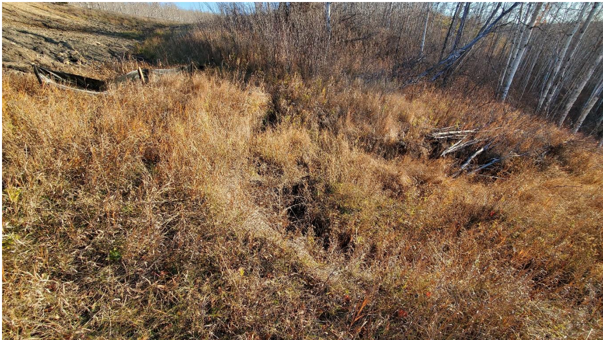
Photo 10 (Oct. 28) – Crest of the slump at the top of the gully.
