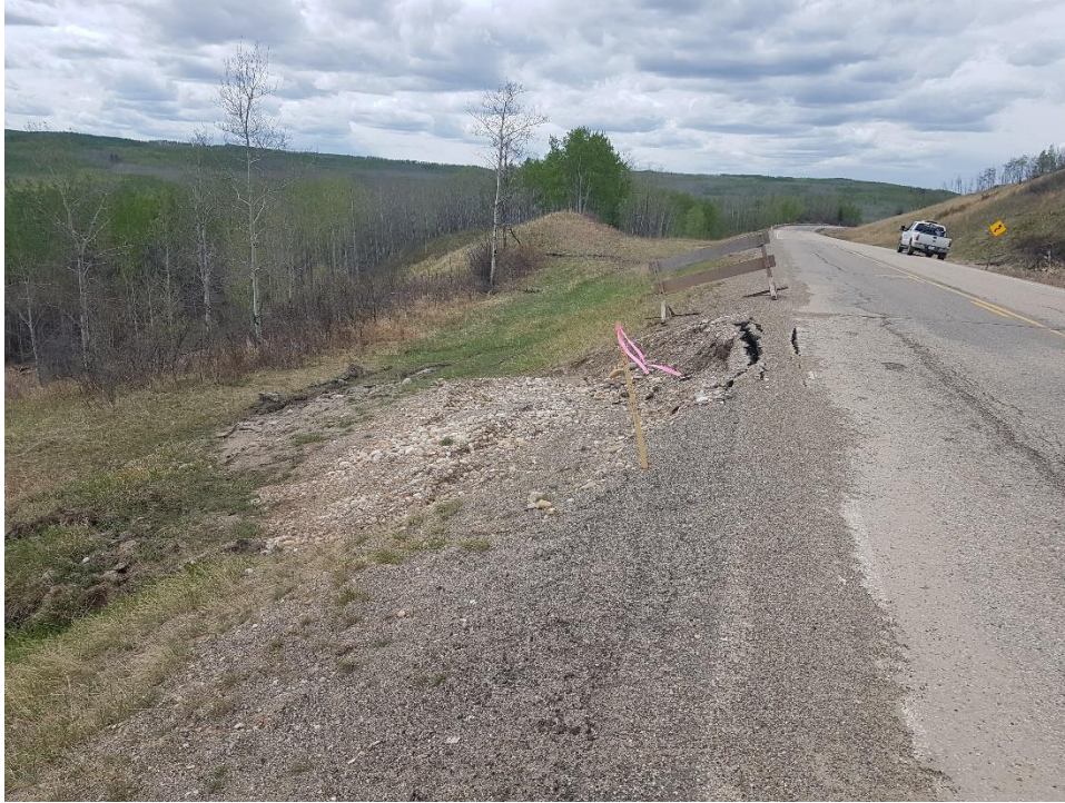
Photo 1 (McIntosh Perry, May 16, 2021) - Looking east at slump with stake at new culvert outlet.
