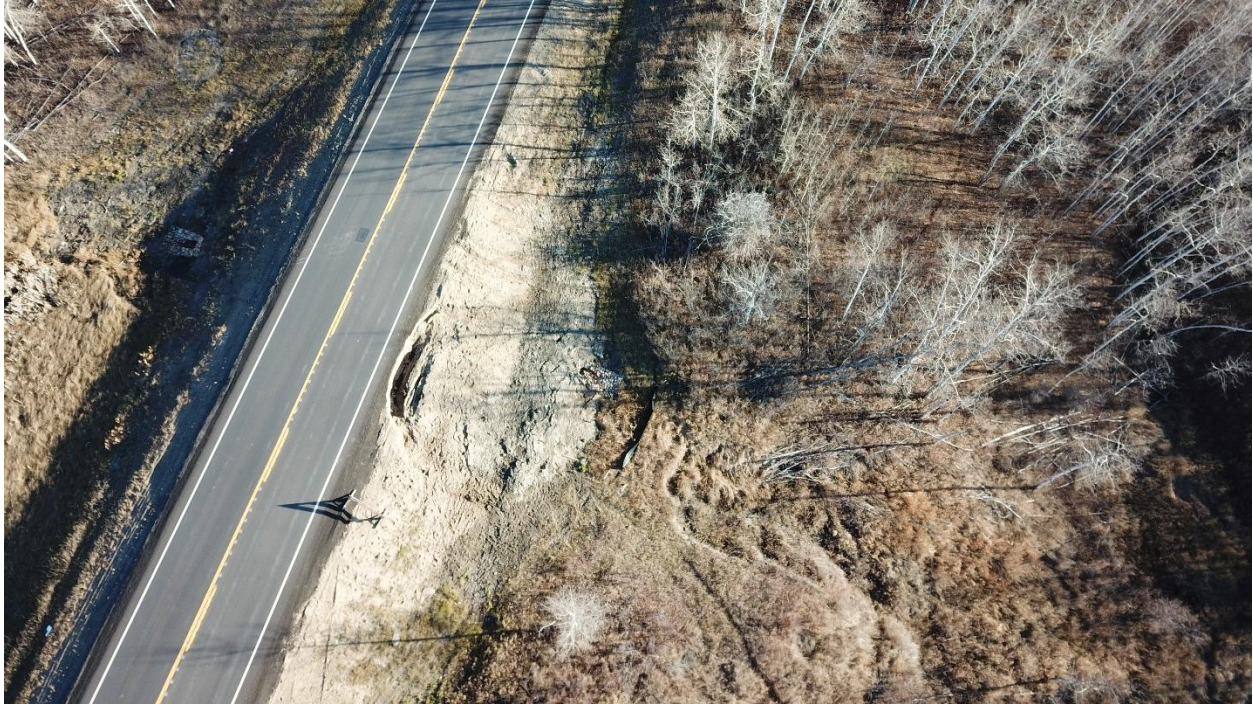
October 28, 2021 - UAV Photo of slide and new culvert. Sag pond is to the right.
