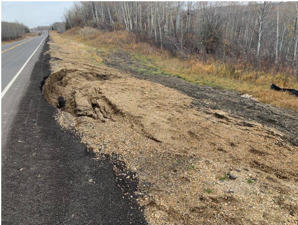
Photo 2 (MCI, Oct. 13) – Looking west at crest of slump
