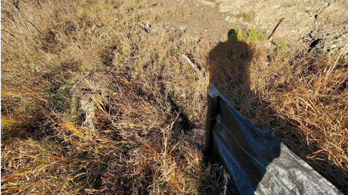
Photo 11 (Oct. 28) – Crack or trench on the west side of the silt fence. Also, note the soft, wet area toward the top of the photo.
