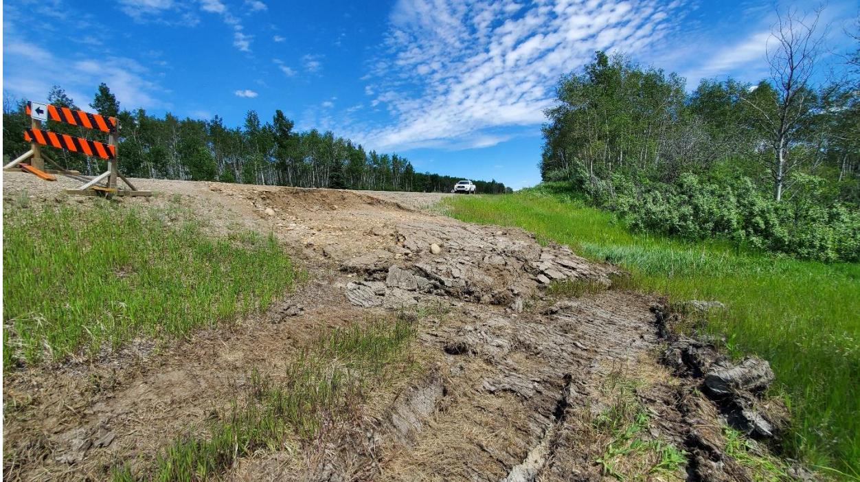
Photo 3, Site 5 (June 24, 2020): Emergency fill placed on the shoulder has also slumped.
