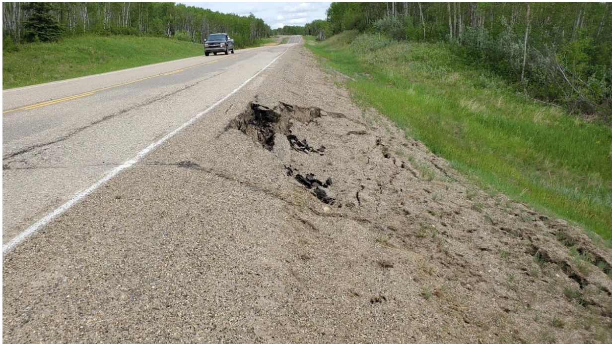
Photo 3: Looking east at new slump on shoulder that has blocked the culvert outlet (km 19.07).
