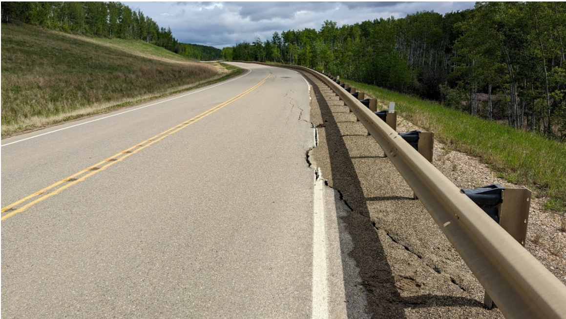
Photo 4– Looking east towards Site #8 where cracks were observed near the guardrail.
