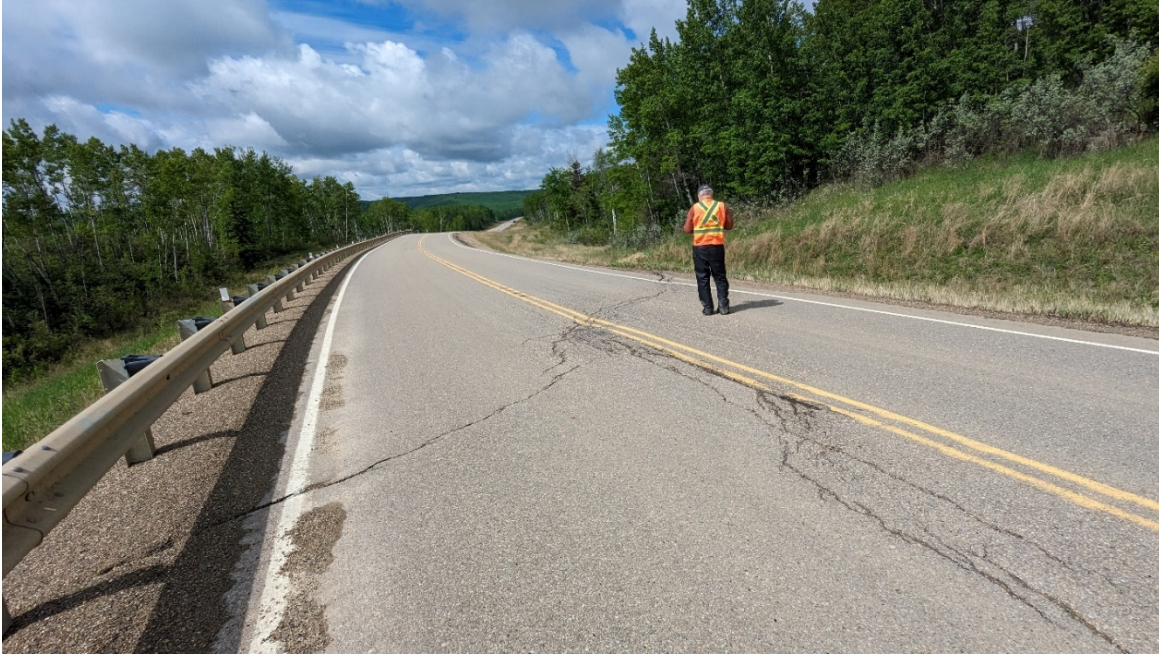
Photo 3 – Looking west at parallel cracks merging together at the centerline.
