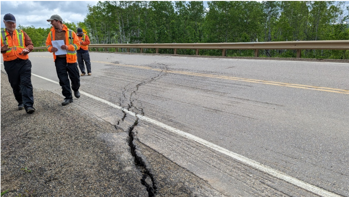
Photo 2 – Looking at cracks merging together and widening where main scarp crosses highway.
