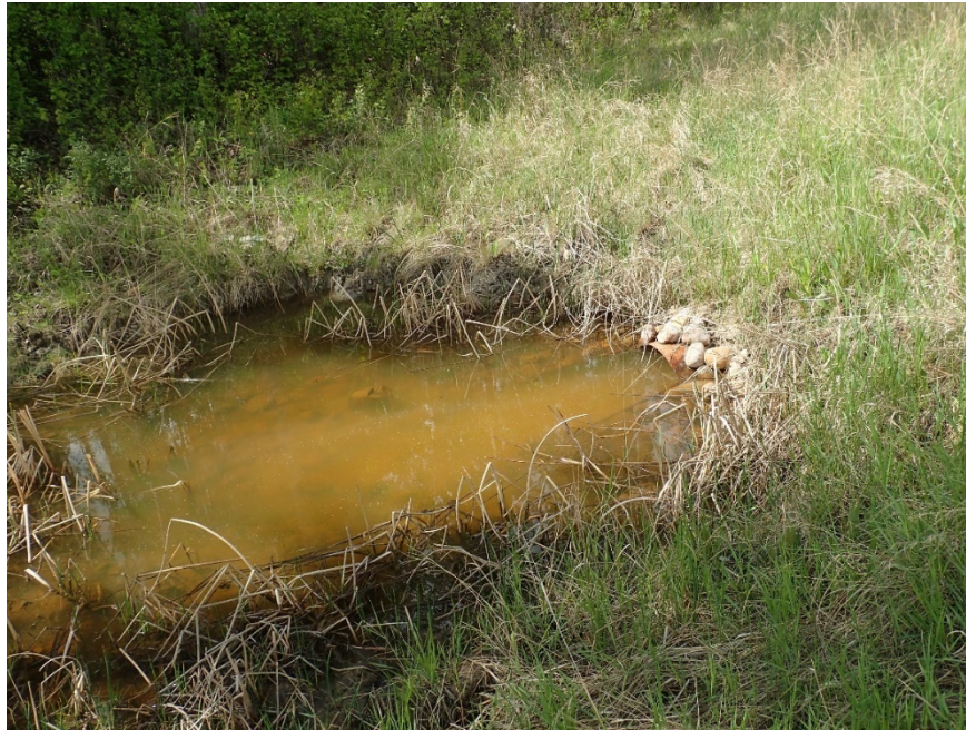
Photo 1, Site 5 – Looking northeast at ponded water at culvert inlet at km 19.07.
