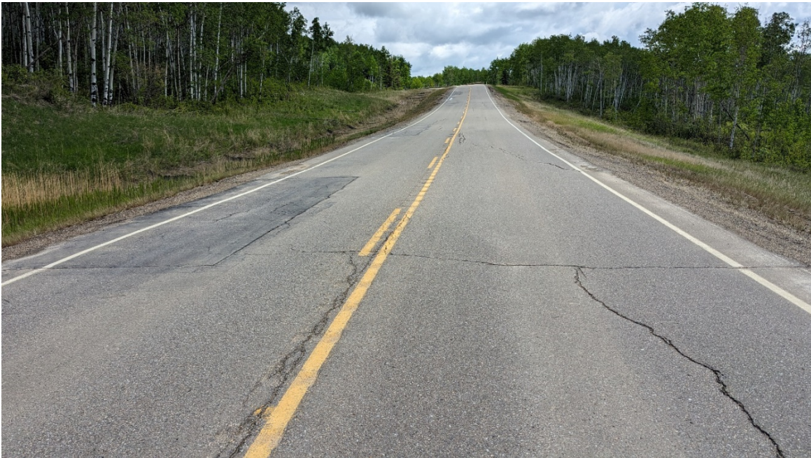
Photo 6, Site 6 – Looking northeast near km 19.3. Dip noted on eastbound lane and recent patches observed on westbound lane.
