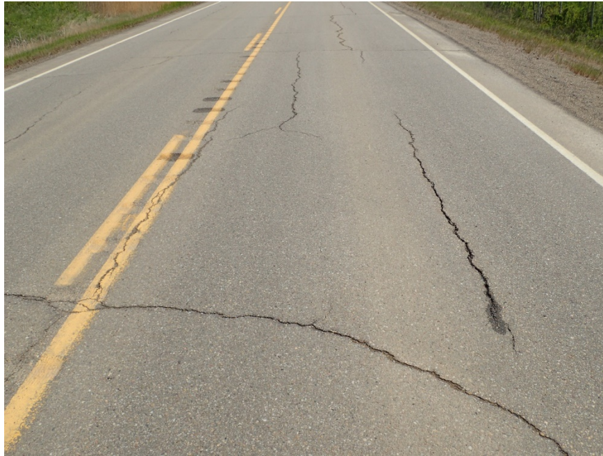
Photo 3, Site 5 – Looking northeast at intermittent cracking between km 19.10 to km 19.13.
