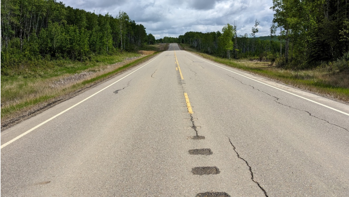
Photo 5, Site 6 – Looking northeast at cracks on the road south of the culvert.
