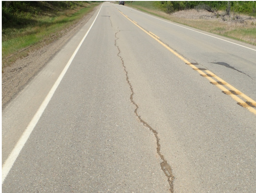
Photo 2, Site 5 – Looking west at crack pattern on the eastbound lane.
