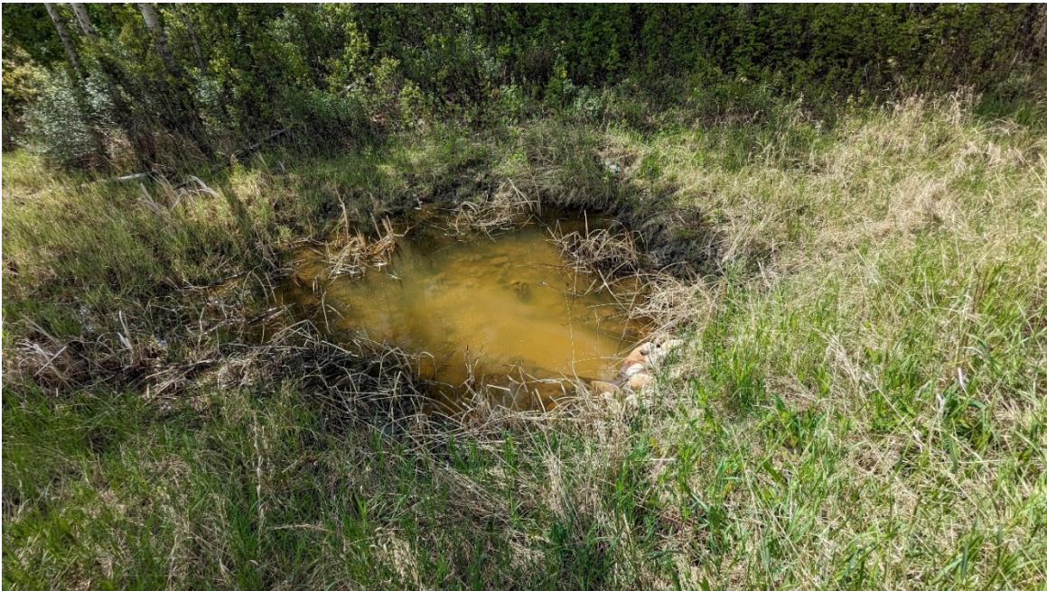
Photo 8, Site 6 – Looking southwest at culvert outlet that has pooled water because it is not draining.
