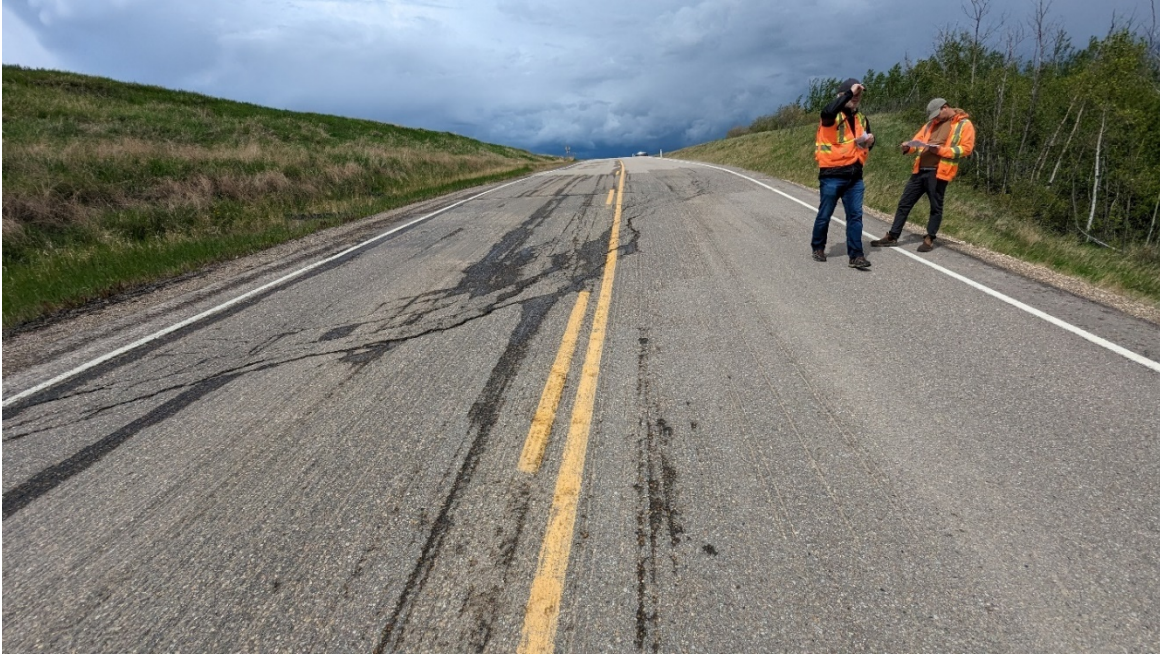
Photo 5, Site 15 – Looking north at diagonal crack intersecting the highway that was recently milled.
