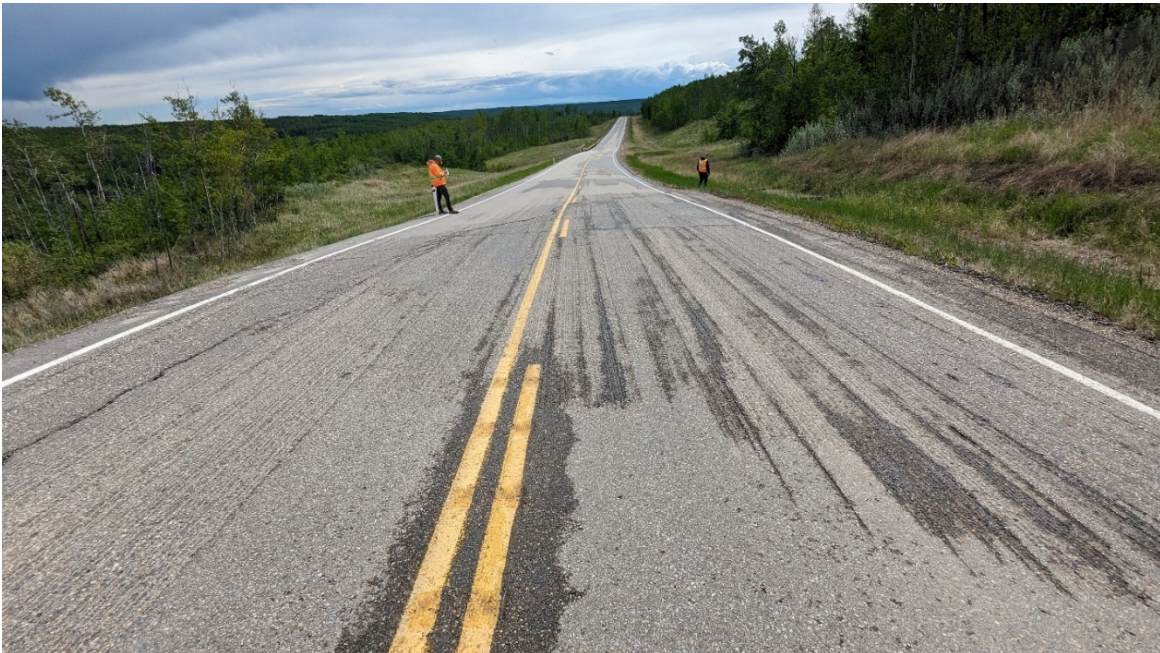
Photo 6, Site 15 – Looking south at the main crack and milled section of road.
