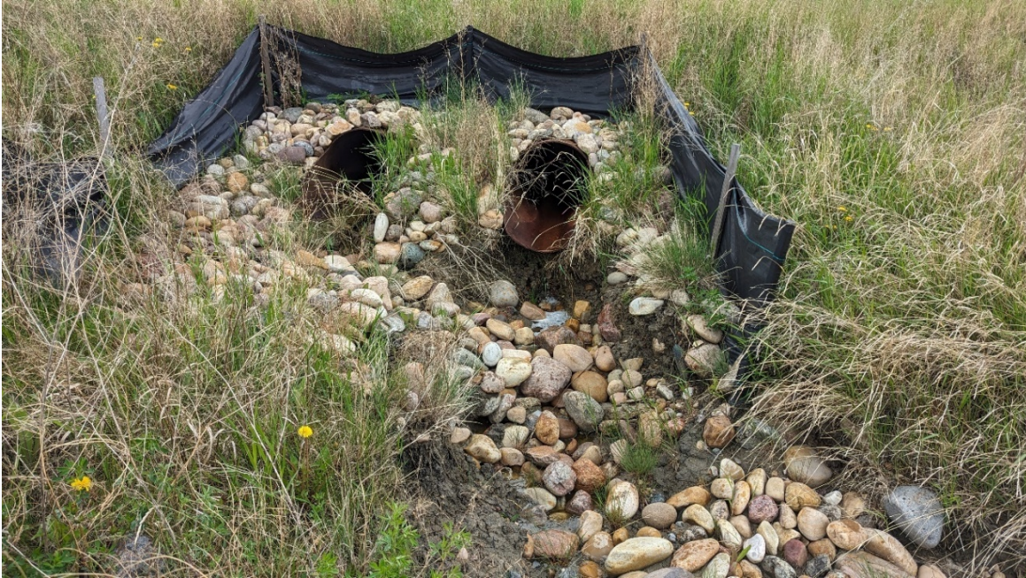
Photo 3, Site 14 – Looking at outlets of SWSP twin culverts outlets. The riprap apron at the north SWSP had collapsed.
