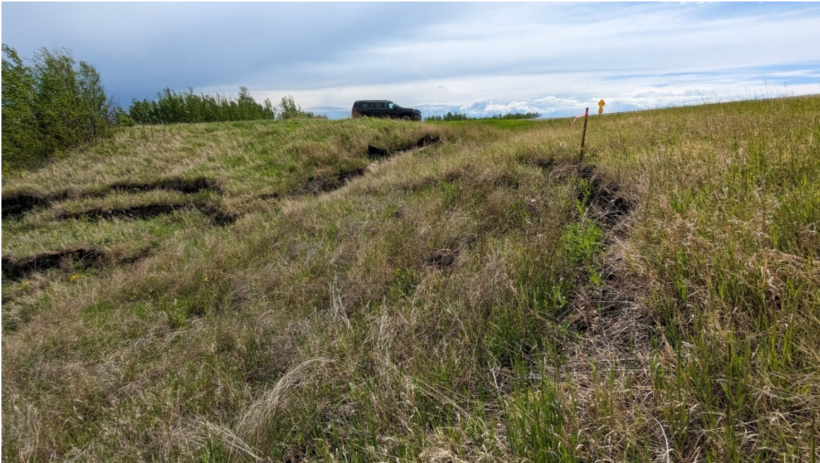
Photo 1, Site 14 – Looking southwest at slide scarp north of twin culverts that is retrogressing towards the highway.
