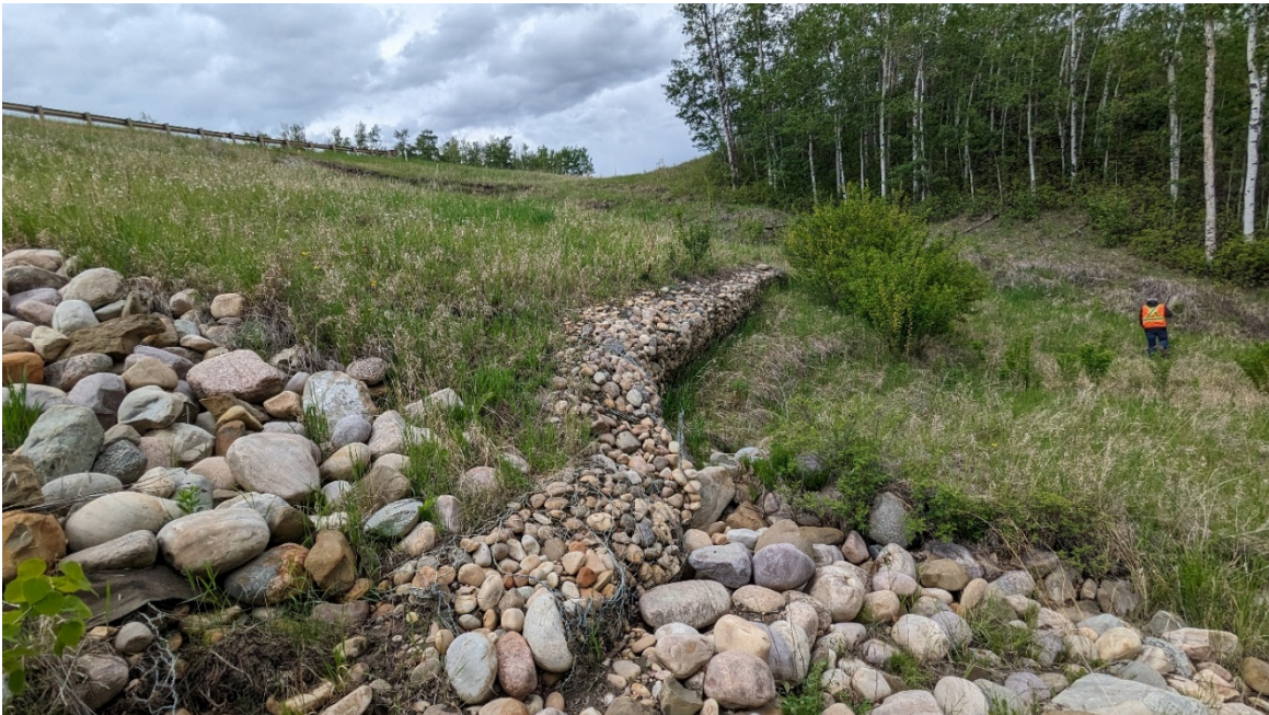
Photo 6 – Looking north at the distorted gabion wall and riprap apron as well as slumping below the wall.
