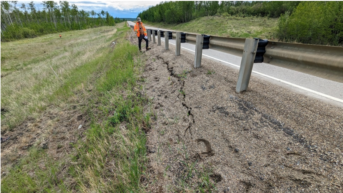
Photo 8 – Looking south at tension crack forming east and downslope of the guardrail.
