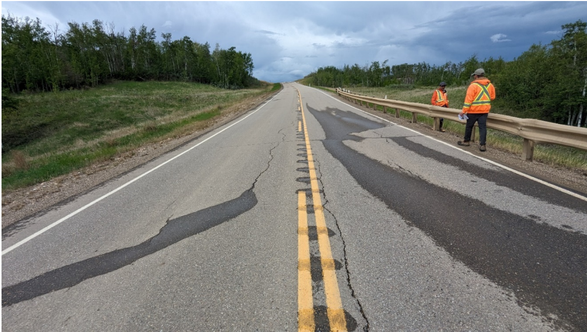
Photo 1 – Looking north where the crack pattern is starting to reflect through the 2021 overlay.
