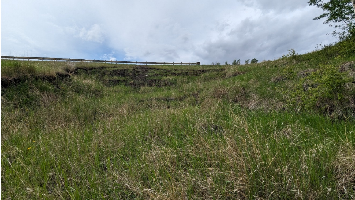
Photo 7 – Looking northwest at top of east embankment slide.
