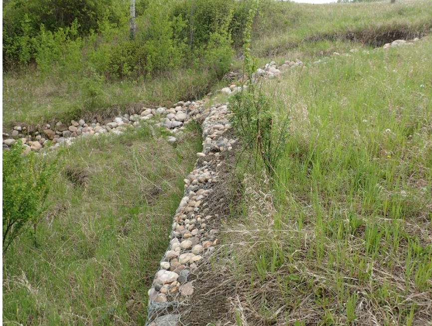
Photo 5 – Looking south at gabion wall on downslope side of embankment. Note eroded south face of riprap apron from culvert outlet.
