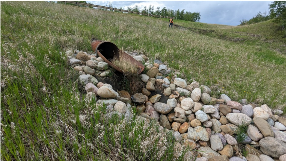
Photo 4: Looking northwest at hanging culvert outlet. Erosion on left-hand side (south) is worse and may be part of a retrogressive tension crack from the slide further down the slope.
