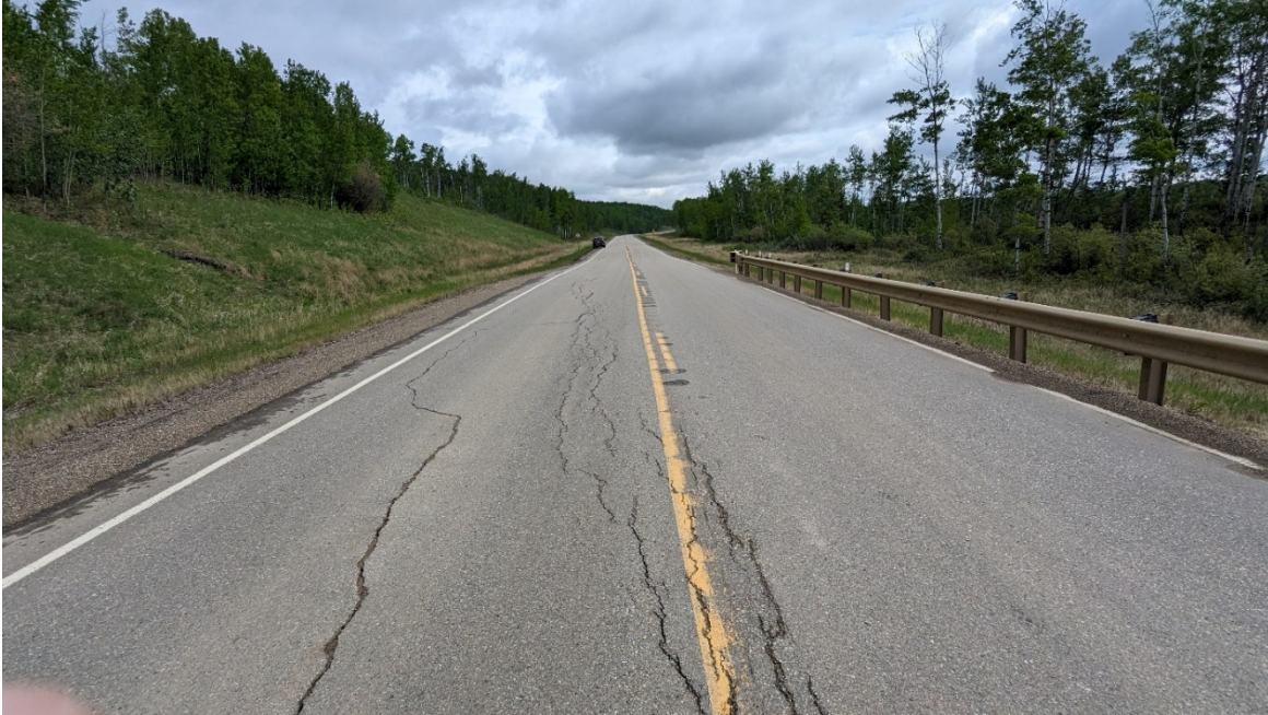
Photo 5, Site 9: Looking northeast at cracking near northeast end of site.
