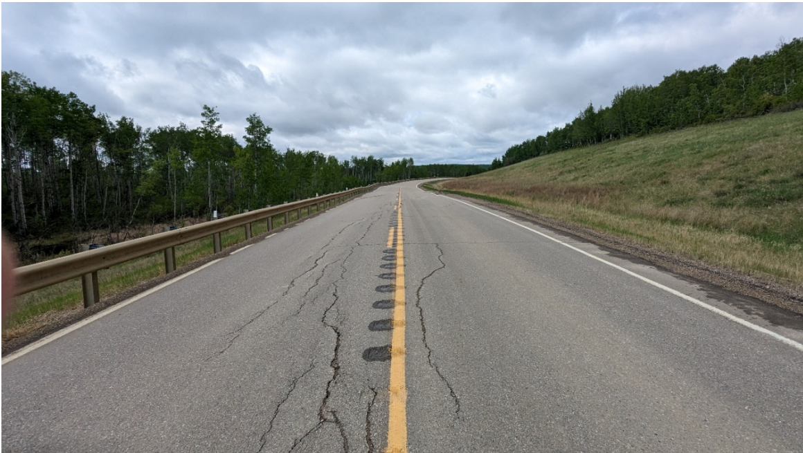
Photo 6, Site 9: Looking southwest at cracks along main slide scarp.
