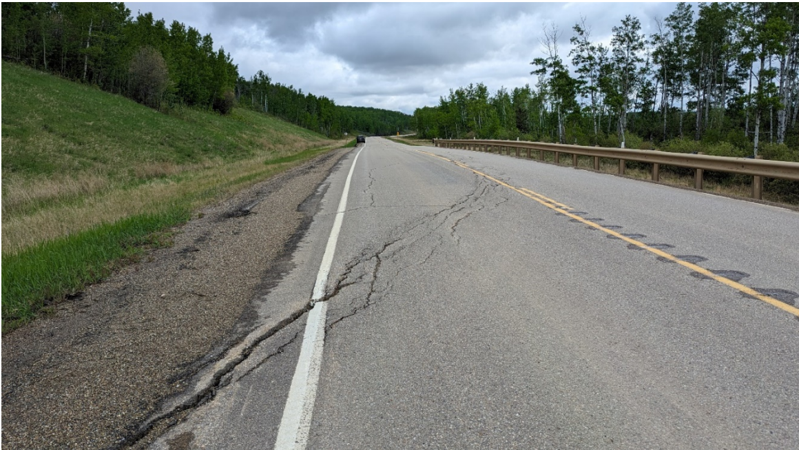
Photo 4, Site 9: Looking northeast at crack in highway surface over main slide scarp that has resurfaced.
