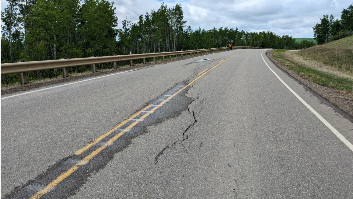
Photo 3, Site 8 – Looking southwest at crack crossing from the WBL towards the centerline and EBL.
