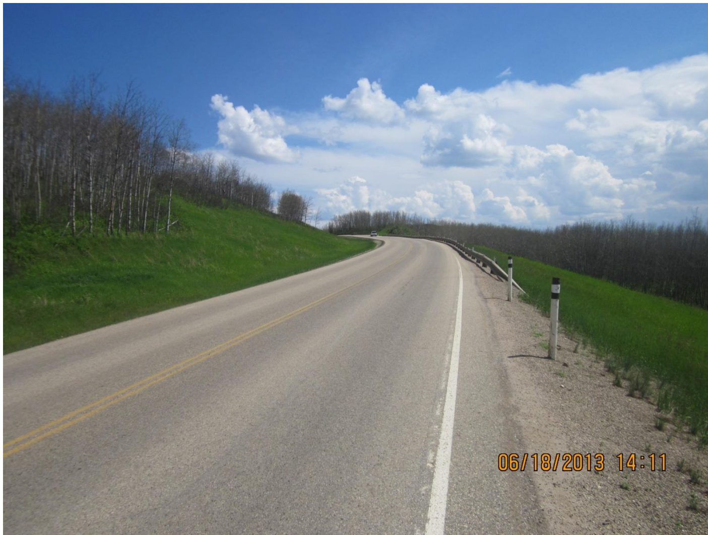
Photo 1: Looking upgrade to the east at the SH11-3 road surface
