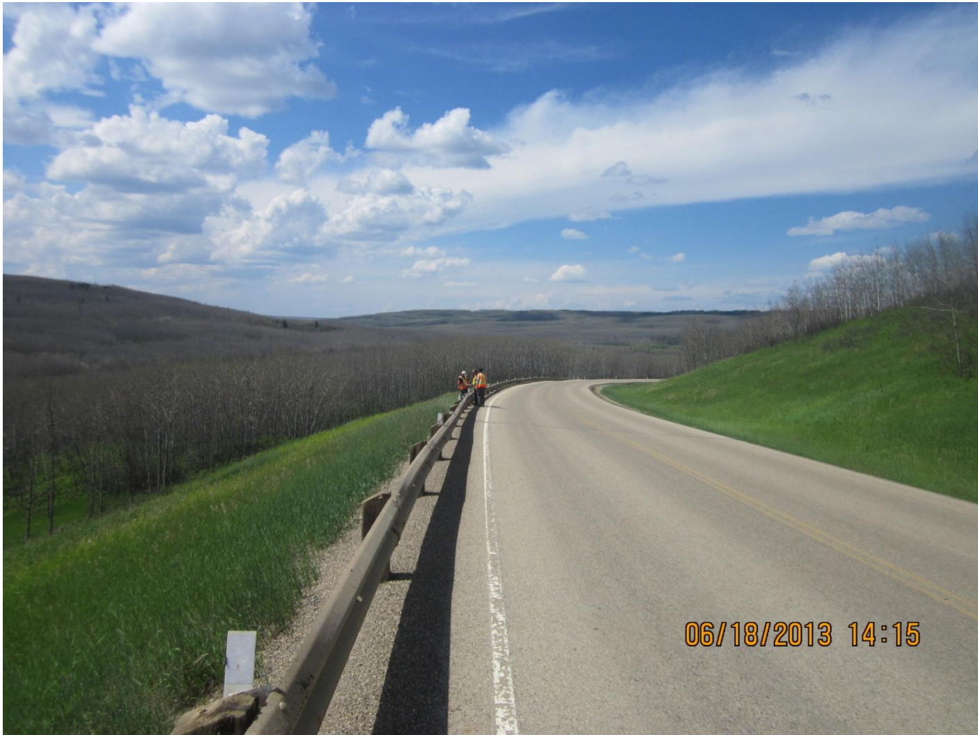
Photo 3: Looking downgrade to the west at the SH11-3 road surface. Note transverse cracking near centre of photo.
