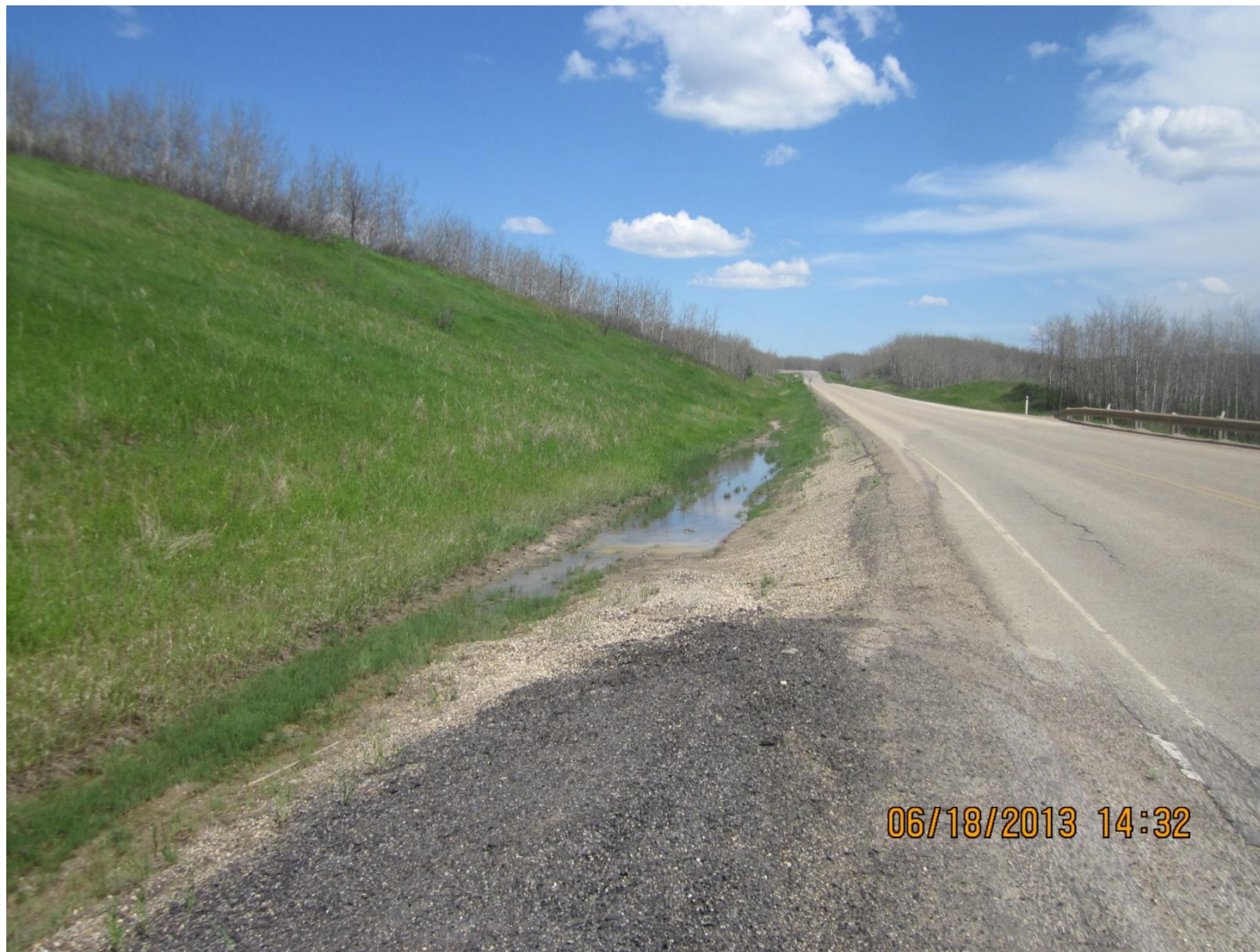
Photo 7: Wet backslope ditch at SH11-4.
