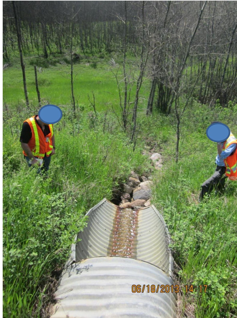
Photo 4: Looking south down the embankment at SH11-3 road surface. Note the sag pond at the bottom of the embankment.
