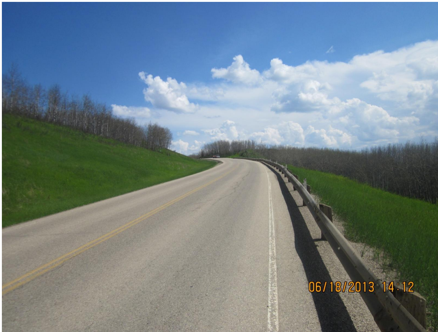
Photo 2: Looking upgrade to the east at the SH11-3 road surface. Note cracking (foreground) and distortion (background).
