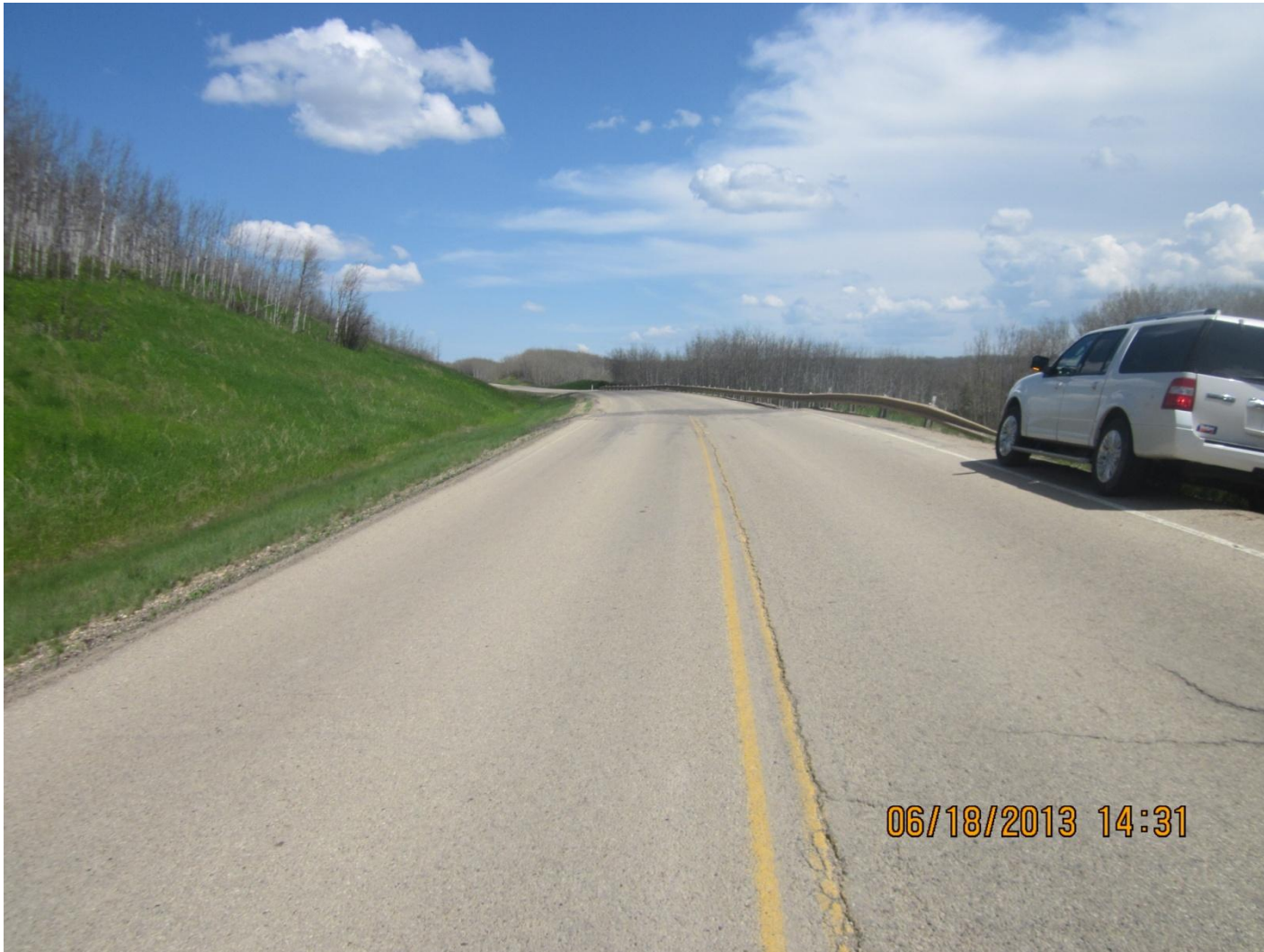
Photo 5: Looking upgrade to the west at the SH11-4 road surface. Note cracking and distortion of pavement.
