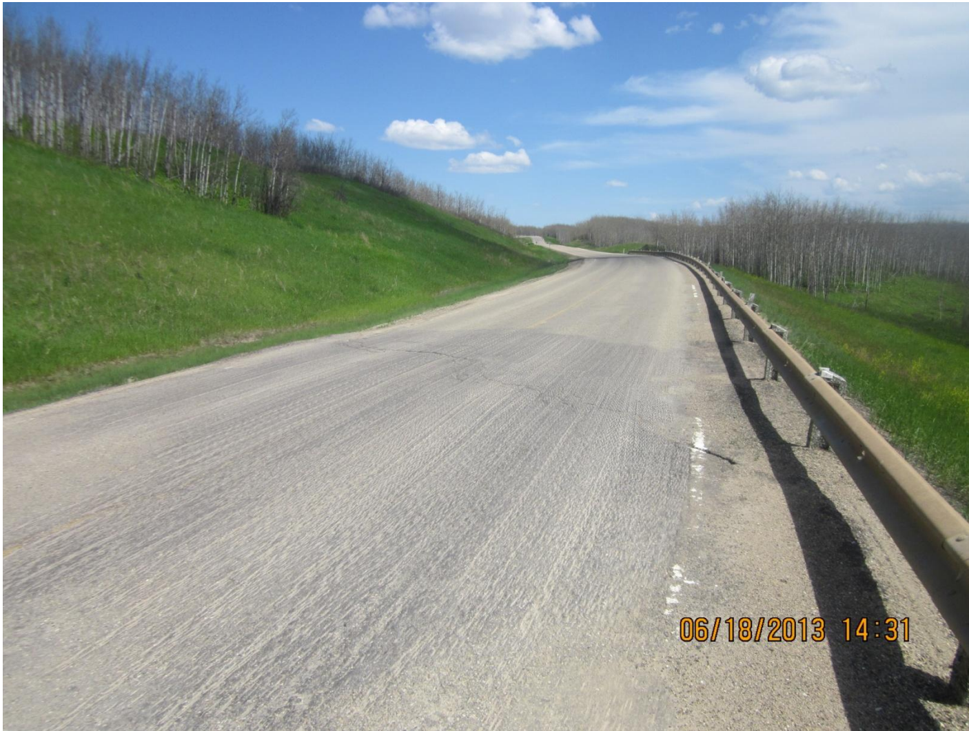
Photo 6: Looking upgrade to the west at the SH11-4 road surface. Note severe transverse crack and distortion of pavement in recently milled area.
