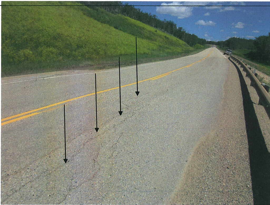
SH11-4 Photo 5. Looking upgrade at SH11-4. Note the undulations in the roadway and the cracking (July 2012).
