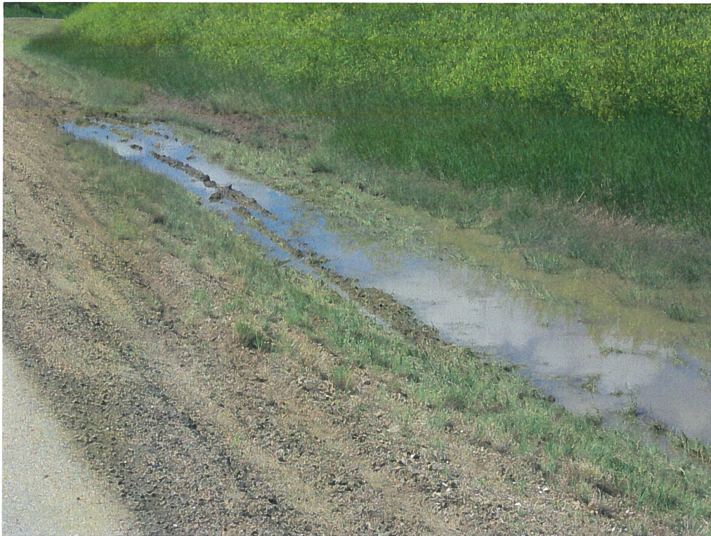
SH11-4 Photo 6. Looking at the wet backslope ditch at SH11-4 (July 2012).
