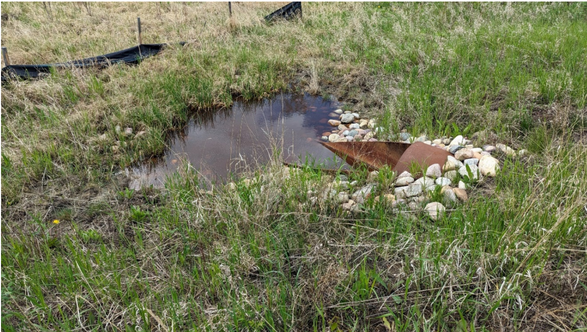
Photo 4, Site 3 –Ponded water observed at culvert outlet at km 18.28
