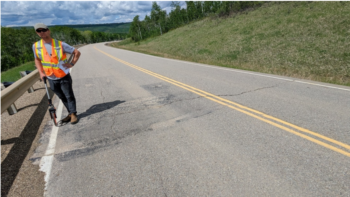
Photo 2, Site 4 – Looking northwest at cracking on patch along EBL.
