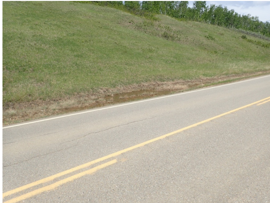
Photo 8, Site 4 – Looking northeast at ponded water in north ditch.
