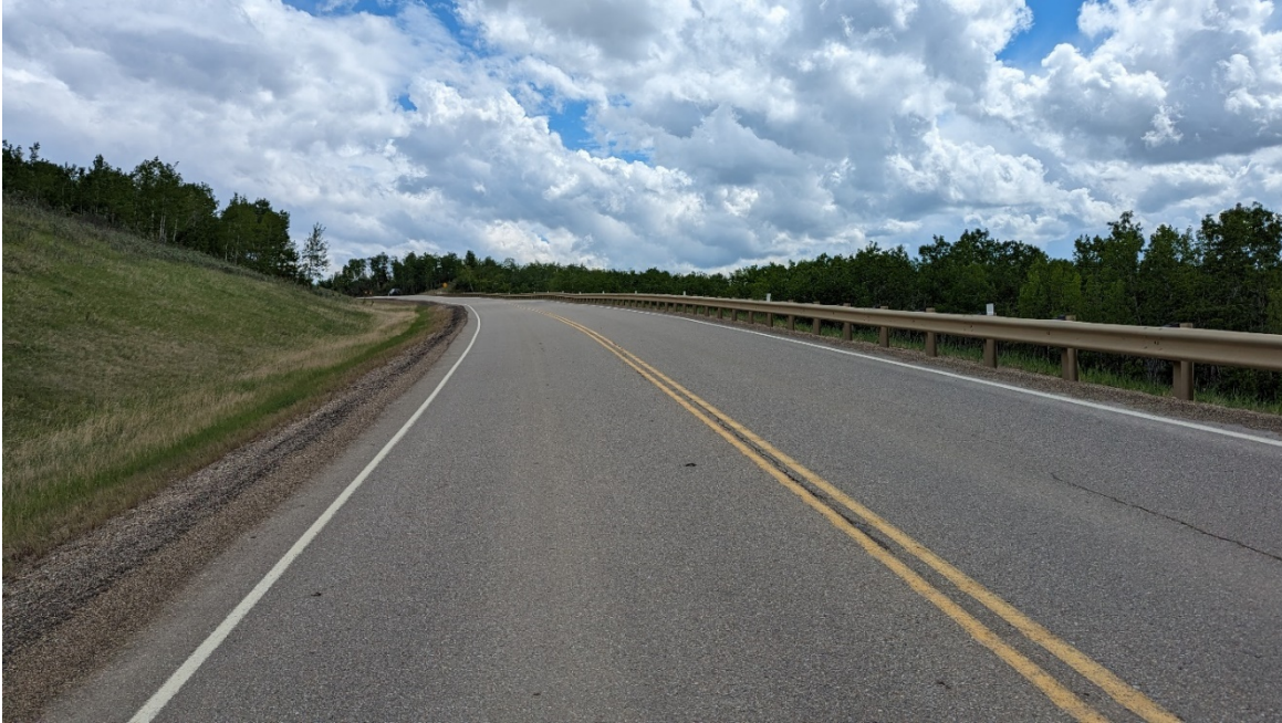
Photo 3, Site 4 – Looking southeast at cracking in highway surface at ~km 18.33.
