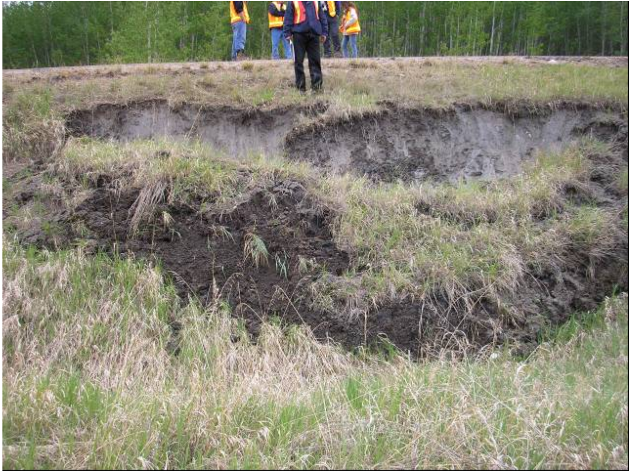
Photo 3 - Looking east (upslope) along slide from middle of slump, slickensides can be noticed, May 24, 2006.
