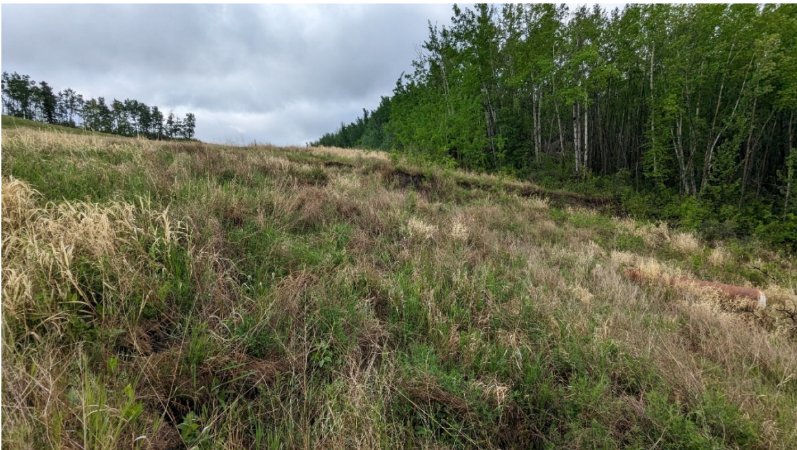
Photo 4 – Looking south at slide at km 14.45 located adjacent to south gabion basket swale. The culvert may be from the previous highway alignment.
