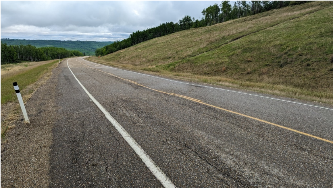
Photo 3 – Looking northeast at crack pattern reflecting through patch on highway above scarps shown in Photo 7.
