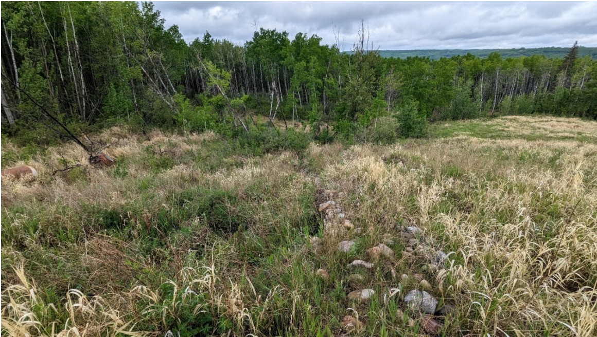
Photo 5 – Looking west where slide at km 14.45 cuts into the gabion basket swale. There has been a lot of vegetative growth in this area.
