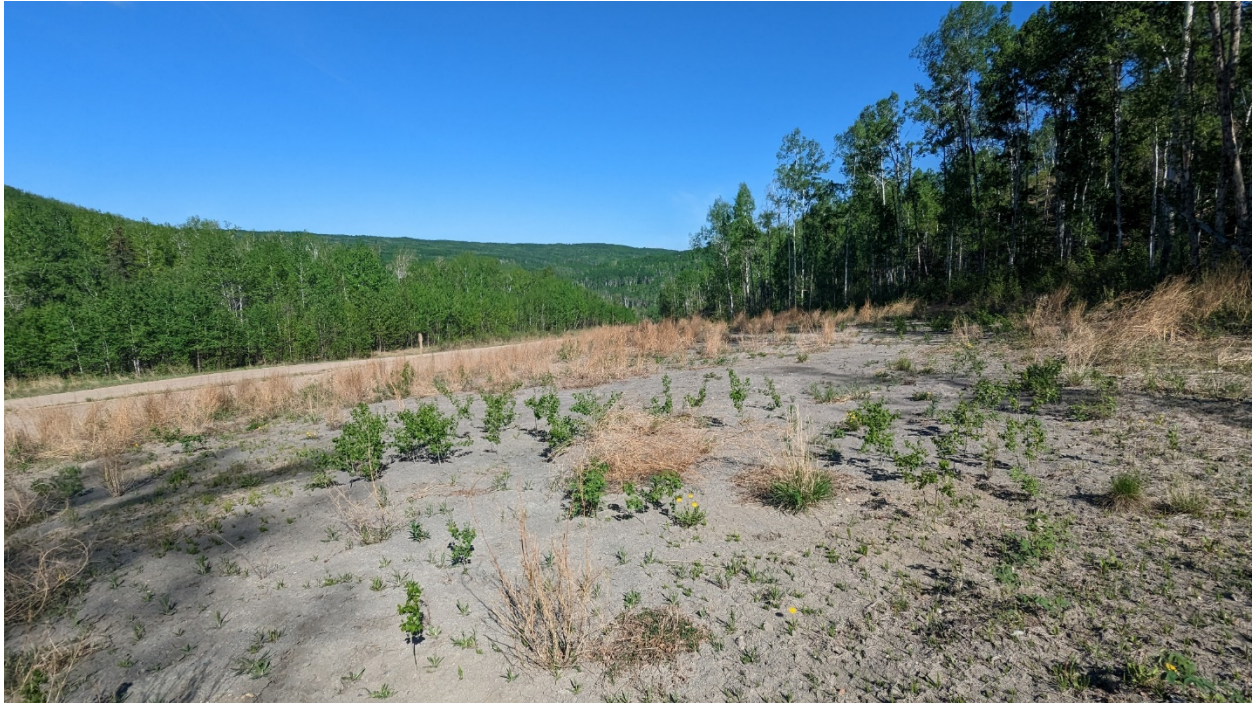
Photo 5 – Looking north at poor vegetation coverage at top of new backslope.
