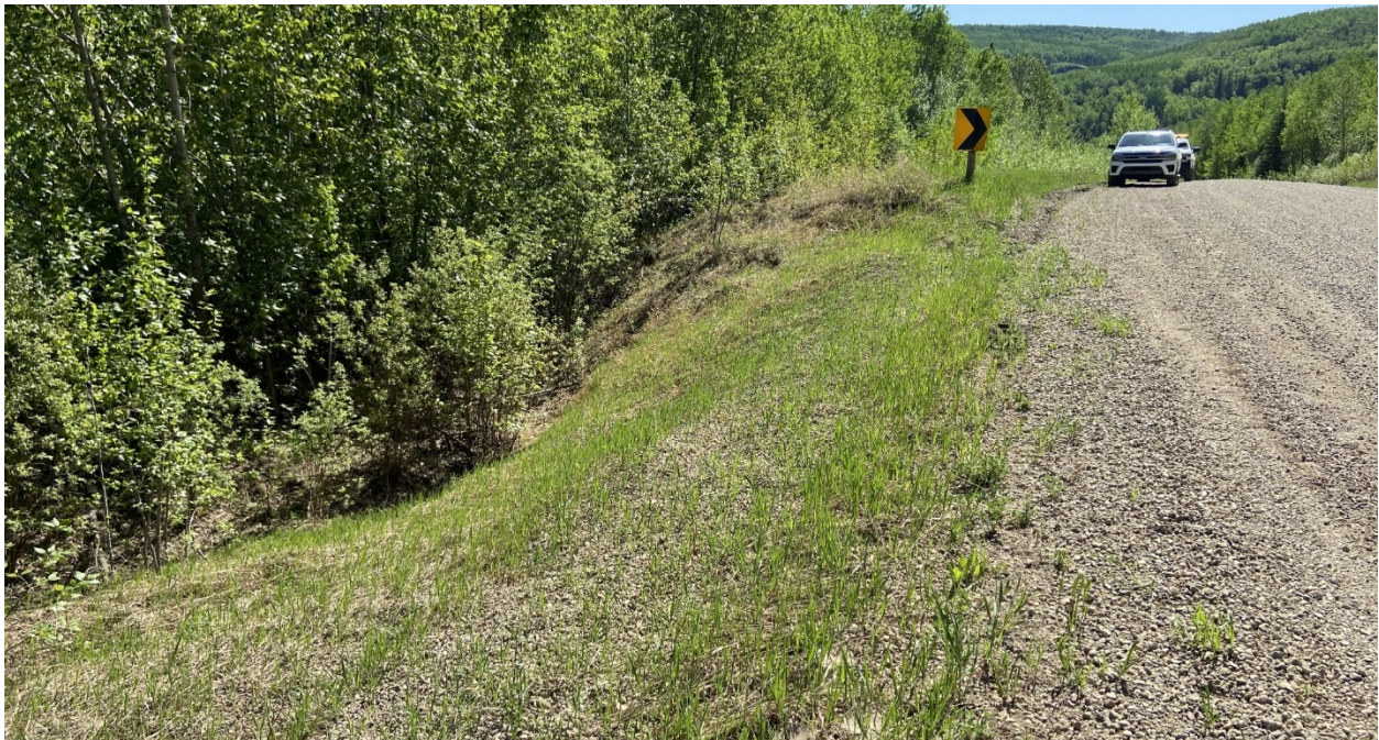
Site 2, Photo 2 – Looking southeast where scarp crack is visible on the east side of the highway.
