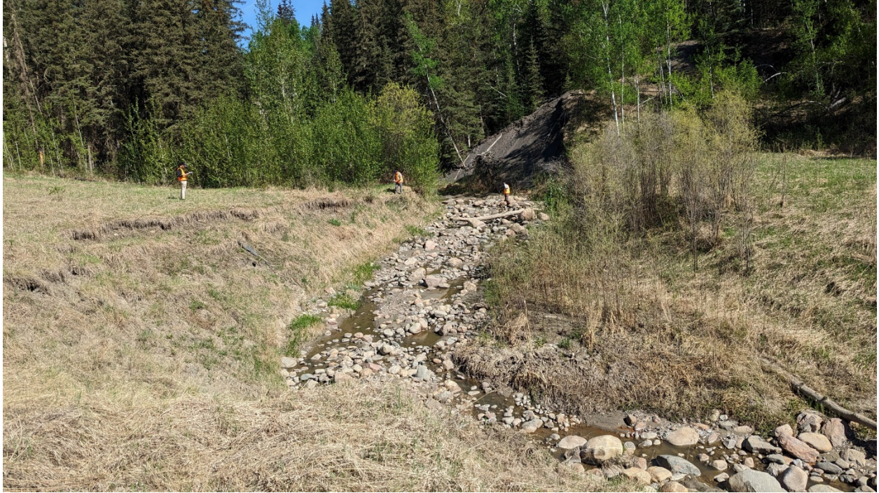
Site 1, Photo 3 – Looking north at creek bank slumping upstream of the culvert inlet.
