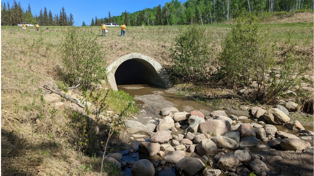
Site 1, Photo 5 – Looking north at culvert outlet. There is significant sediment accumulation.
