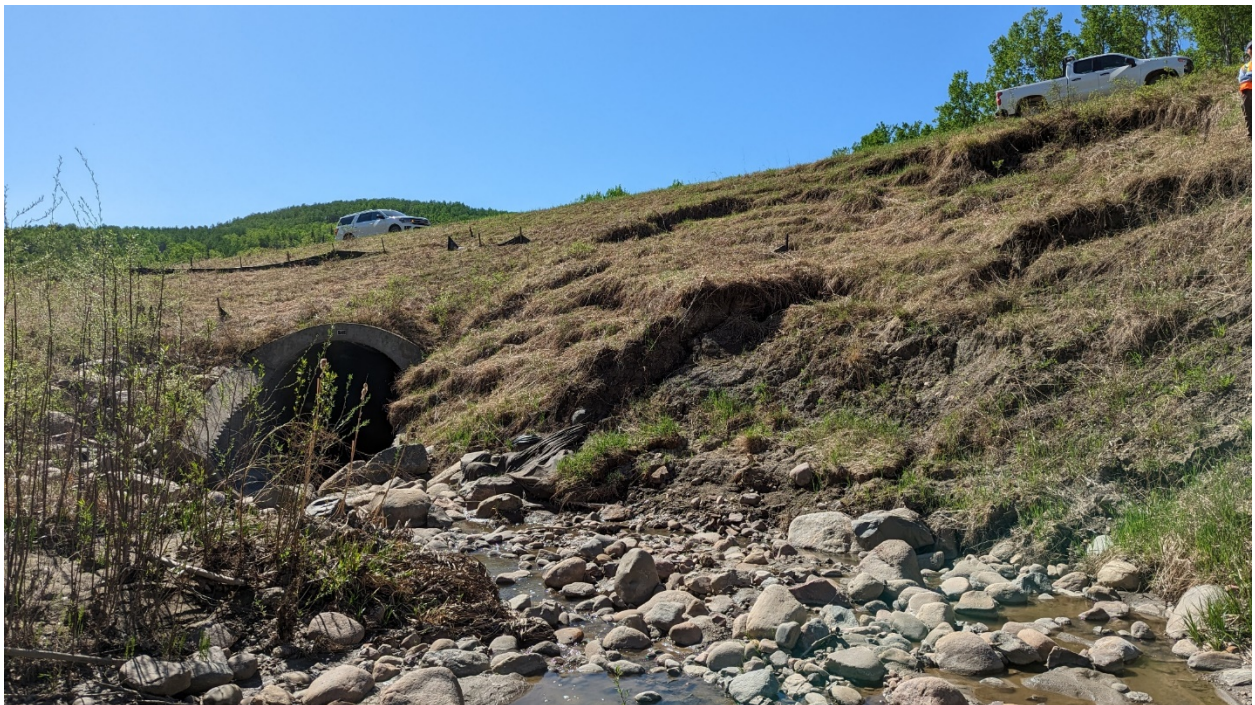
Site 1, Photo 2 – Looking southeast at creek bank slumping upstream of the culvert inlet.
