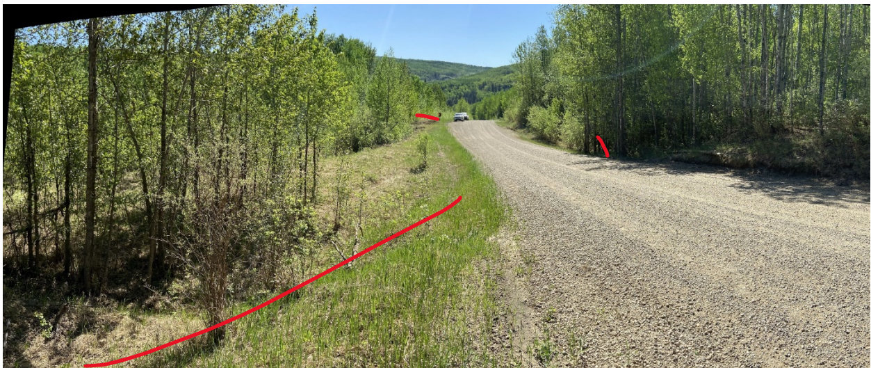
Site 2, Photo 4 (composite) – Looking southeast from north end of the site at the sag in the highway where it crosses the slide mass. The clearly visible scarps are shown with red lines.
