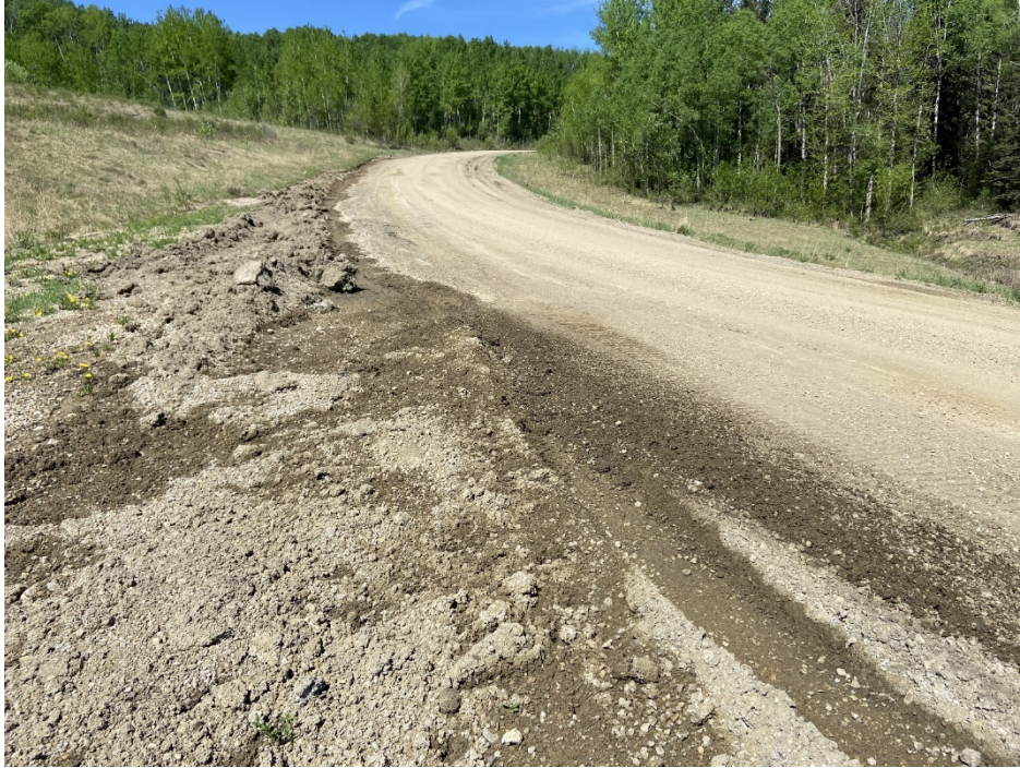
Photo 7 – Looking at seepage along west side of road near the north end of the site.
