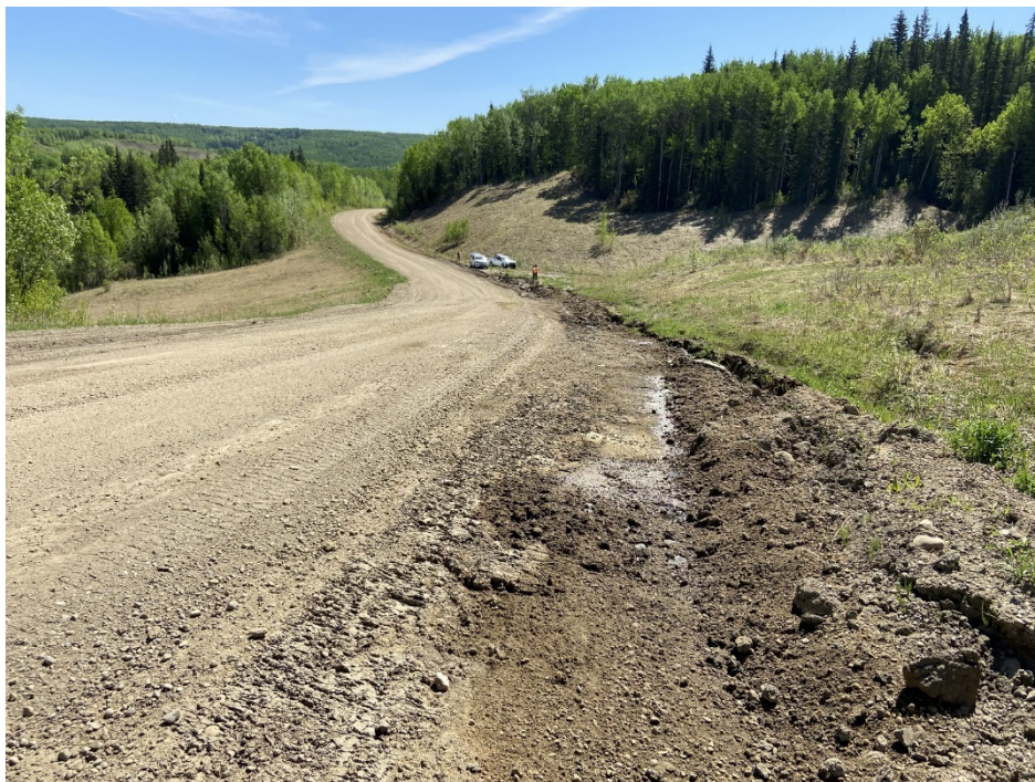
Photo 6 – Looking southwest at road and seepage along west ditch.
