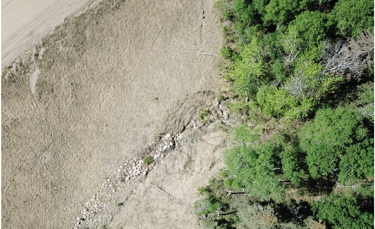
UAV 2023 UAV Image – Slumping at the north end of the of the riprap-lined channel on the east embankment.
