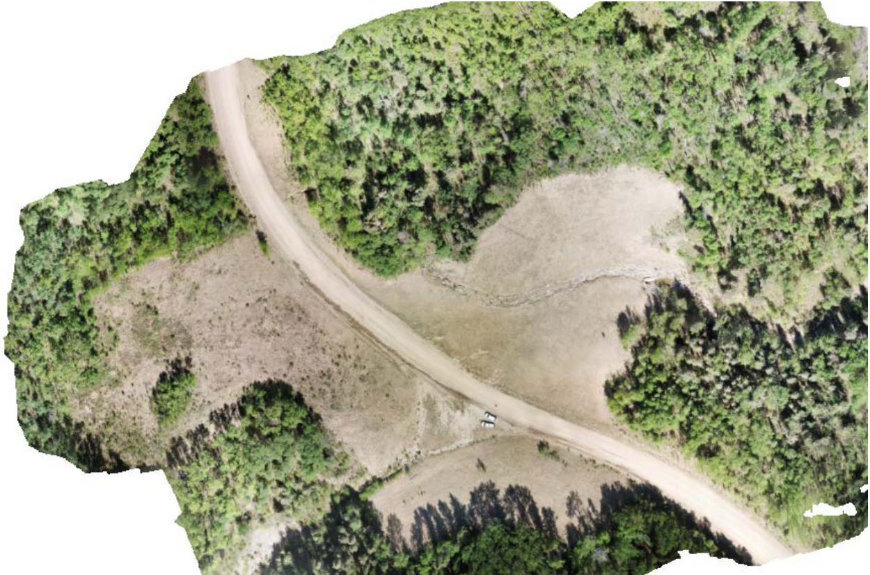
UAV 2023 Orthomosaic: Seepage can be seen along the left side of the highway; the eroding and slumping channel is to the right of the highway.
