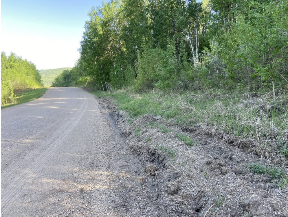
Photo 3 (PH011-3) – Looking north along backscarp crack (in the grass).
