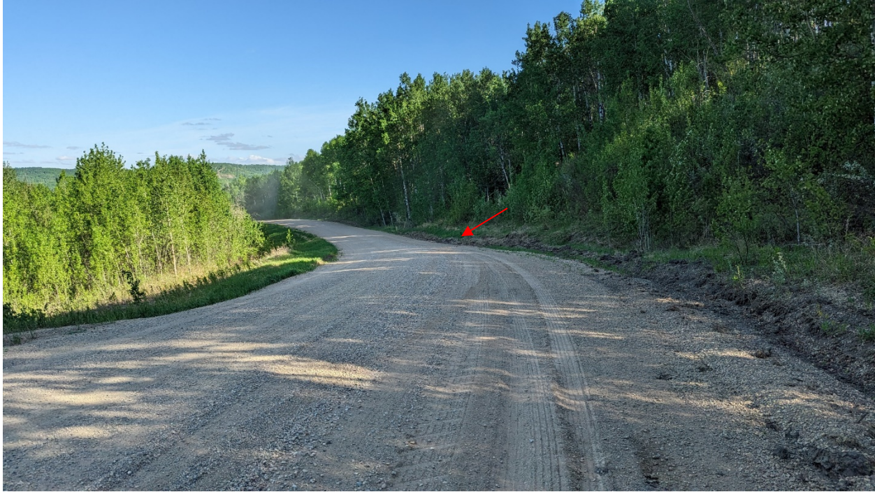
Photo 1 (PH011-3) – Looking north at landslide site identifiable by the dip in the highway surface.
