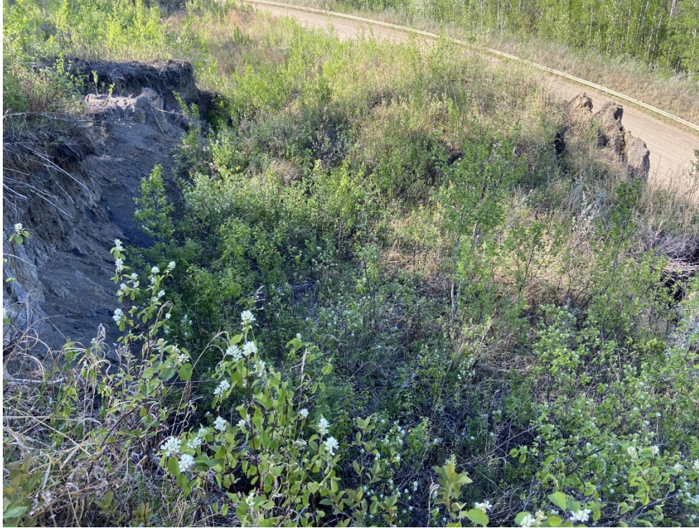
Photo 8 (PH011-2) – There is an evidence of recent scarp cracks opening behind the top of the slope.
