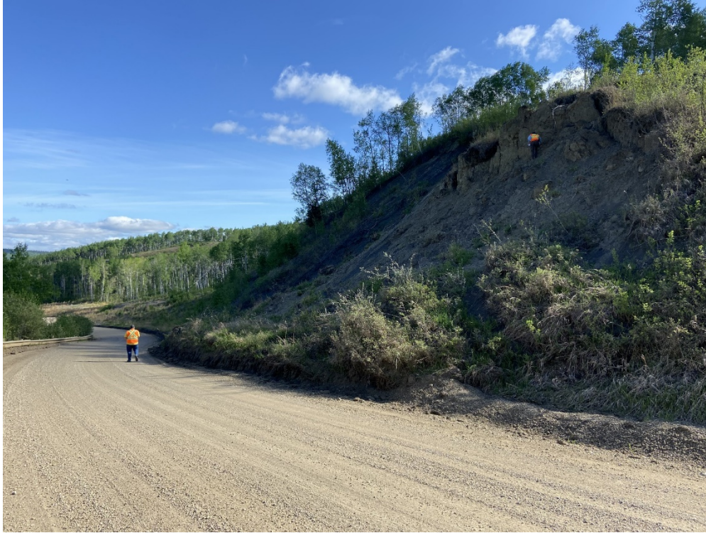
Photo 7 (PH011-2) – There has been a recent movement on this backslope resulting in material accumulating onto the east shoulder of the highway.
