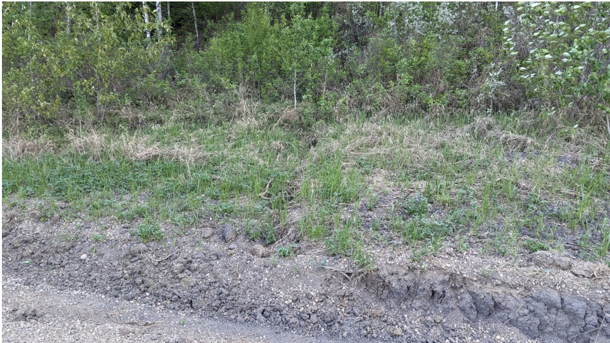
Photo 2 (PH011-3) – Scarp crack beyond the edge of the road.
