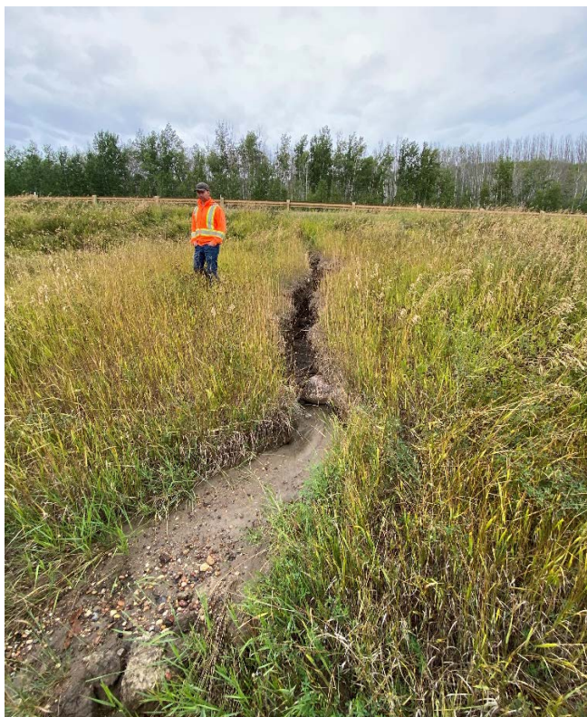
Photo 12. Erosion in sideslope downhill of culvert outlet.
