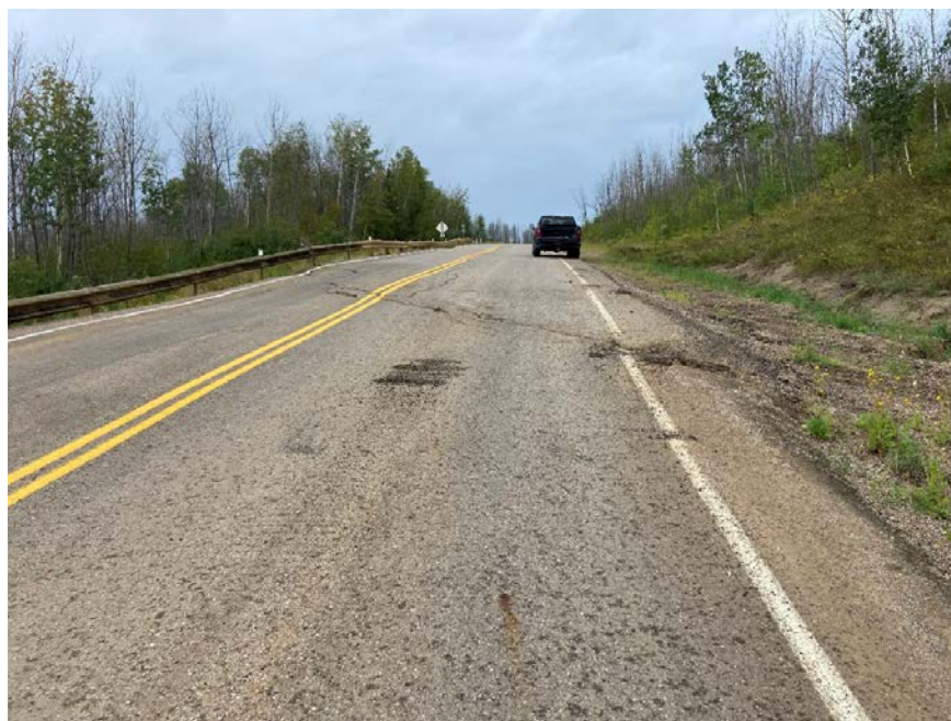
Photo 2. Looking SW at slide crack B.
