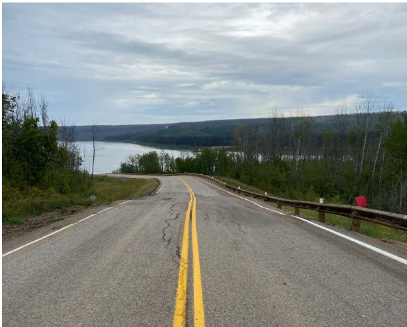
Photo 1. Looking NE at slide Crack B.
