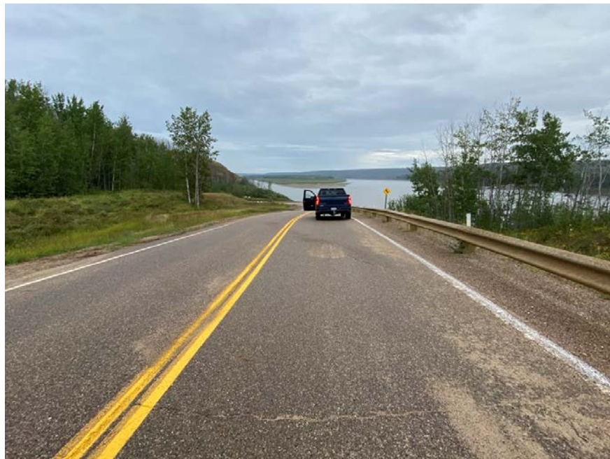
Photo 9. Looking NE at slide crack D.
