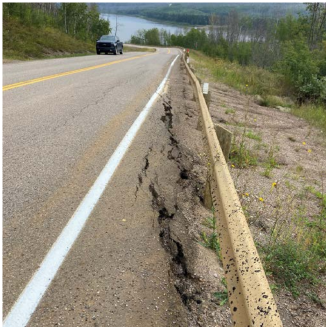
Photo 5. Looking NE at slide crack A.
