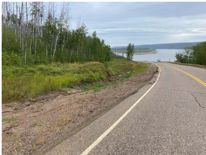
Photo 8. Looking NE at slide crack C with graben in background.
