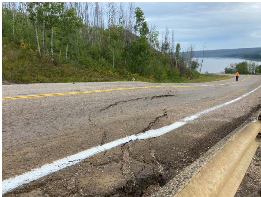
Photo 3. Looking north at Crack B.
