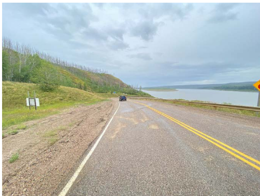
Photo 10. Looking north at slide crack E.
