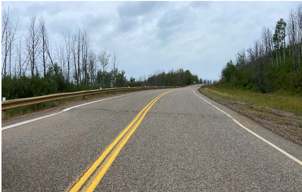
Photo 7. Looking SW at slide crack C.
