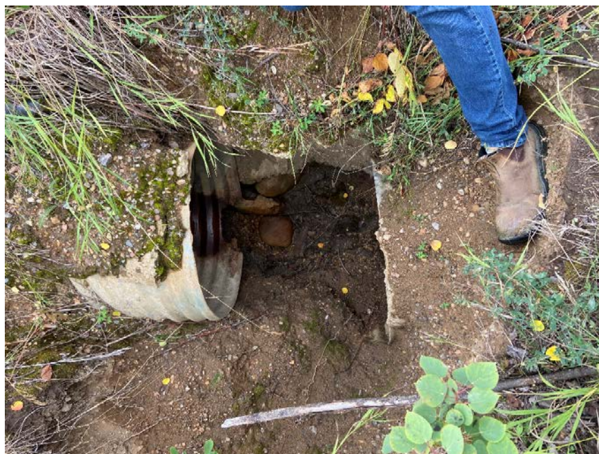
Photo 6. Separation in C.S.P. downpipe at slide crack
