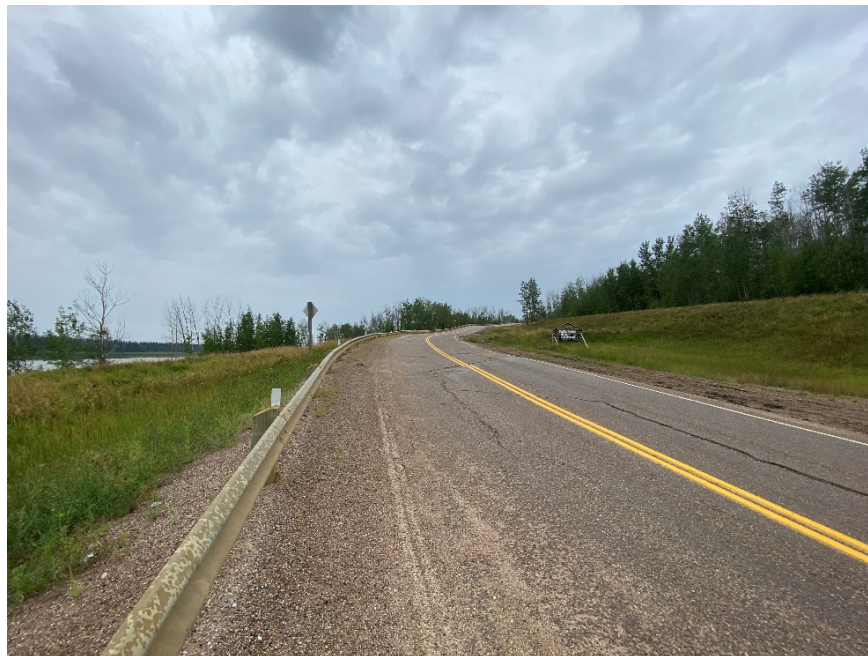
Photo 11. Looking south at slide crack E.
