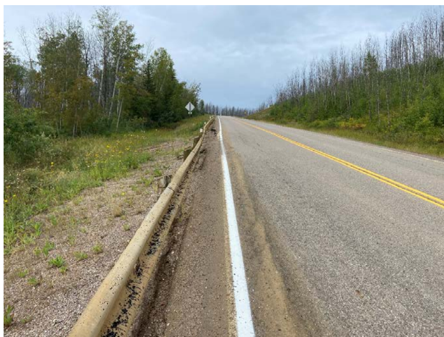
Photo 4. Looking SW at slide Crack A.
