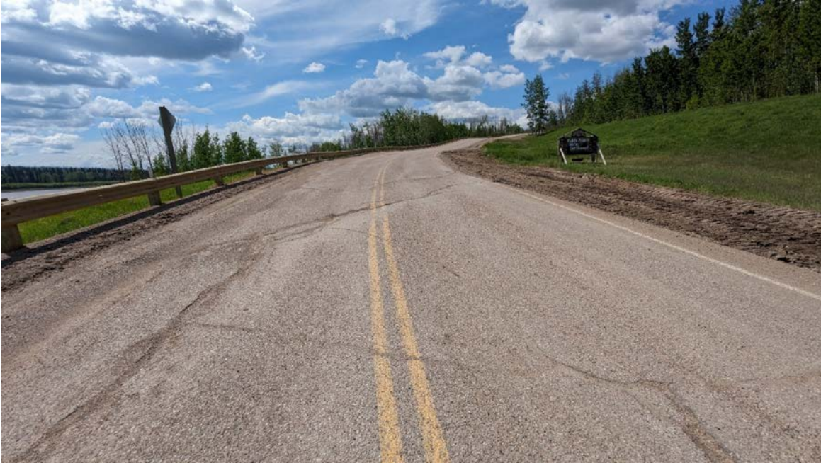
Photo 9 – Cracks on highway near bottom of valley.
