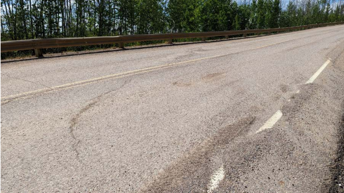
Photo 5 – Diagonal crack across the highway at Sta. 17+240.
