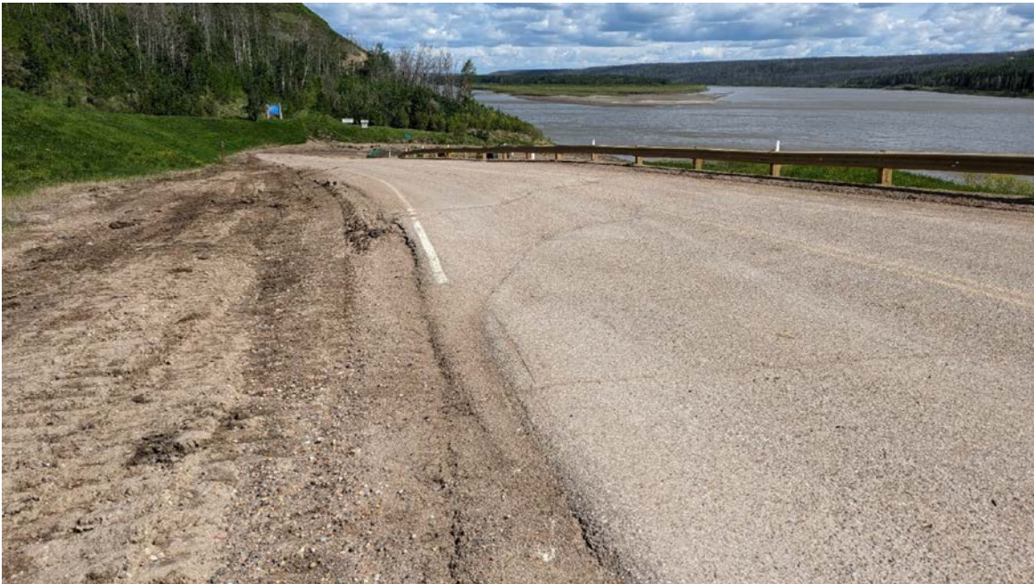
Photo 10 – Looking northeast at cracks on the highway and recent regrading on the upslope side.
