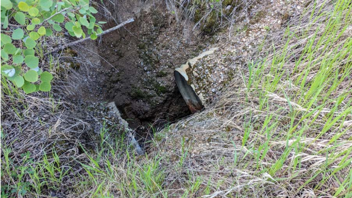
Photo 3 – Sinkhole at separated 800 mm CSP downpipe south of the highway.
