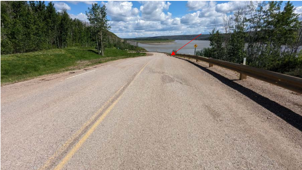
Photo 6 – Looking northeast across the diagonal crack from Photo 5 at another dip in the highway (red arrow).
