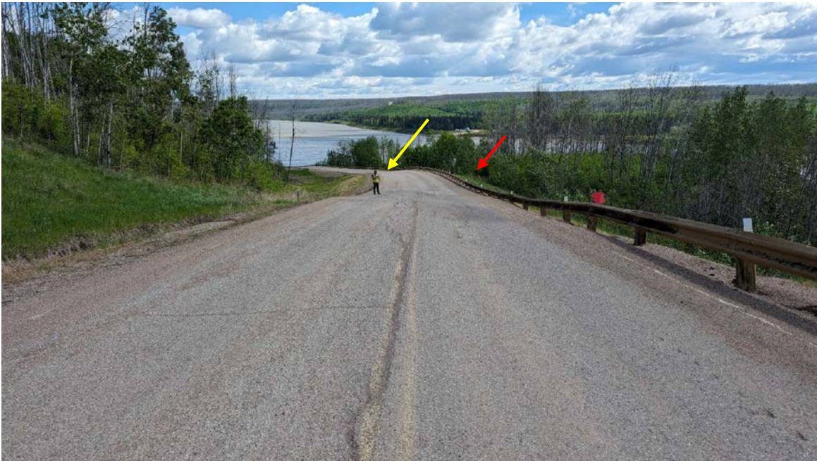
Photo 2 – Looking northeast at dips in the road (yellow arrow and red arrow).
