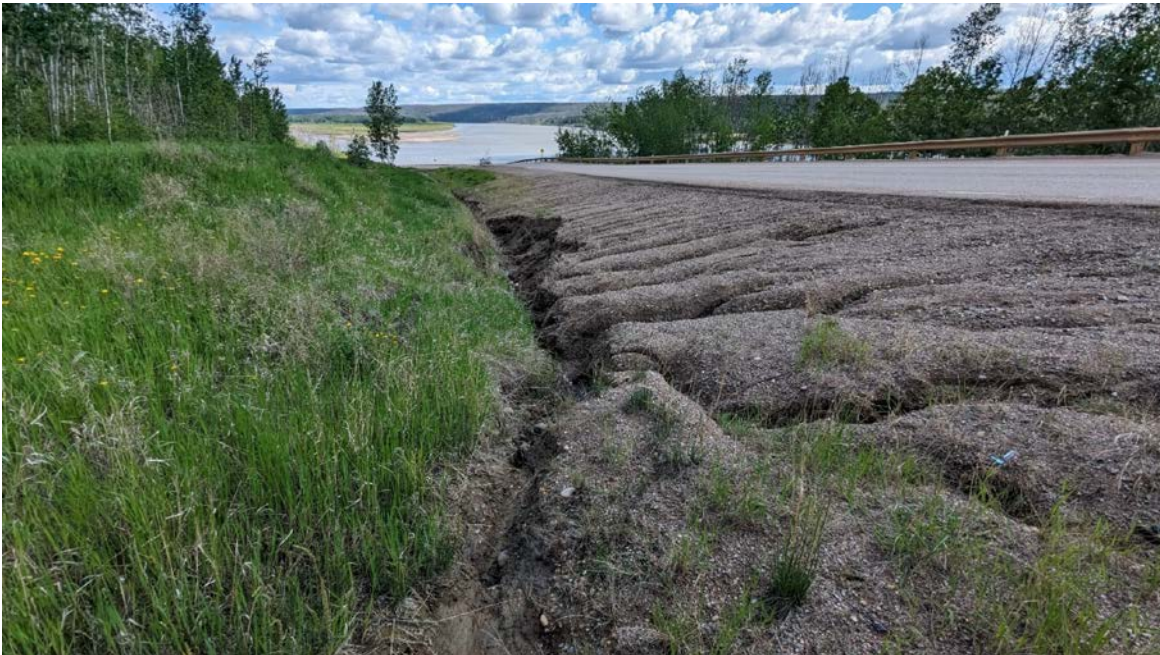
Photo 4 – Looking northeast at deep erosion gully in upslope ditch.
