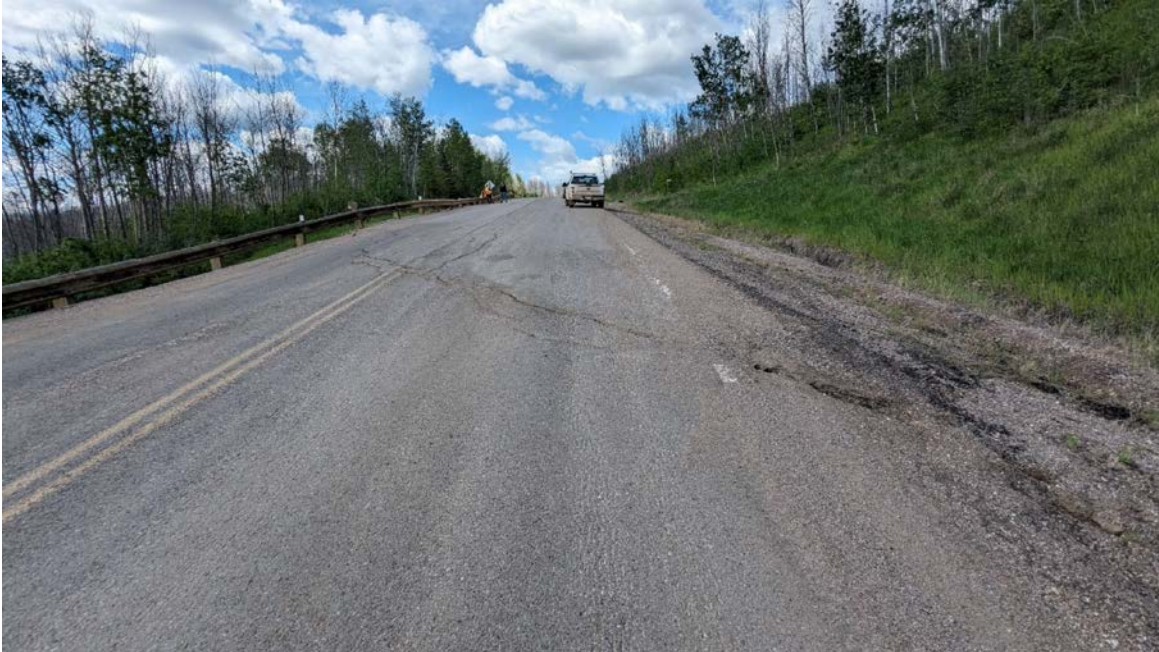
Photo 1 – Looking west at the main scarp crack near the top of the valley at Sta. 17+015.
