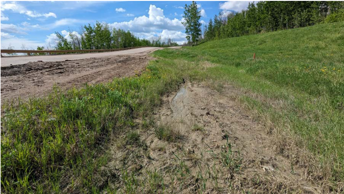
Photo 8 – Looking southwest at accumulating sediment at bottom of valley.
