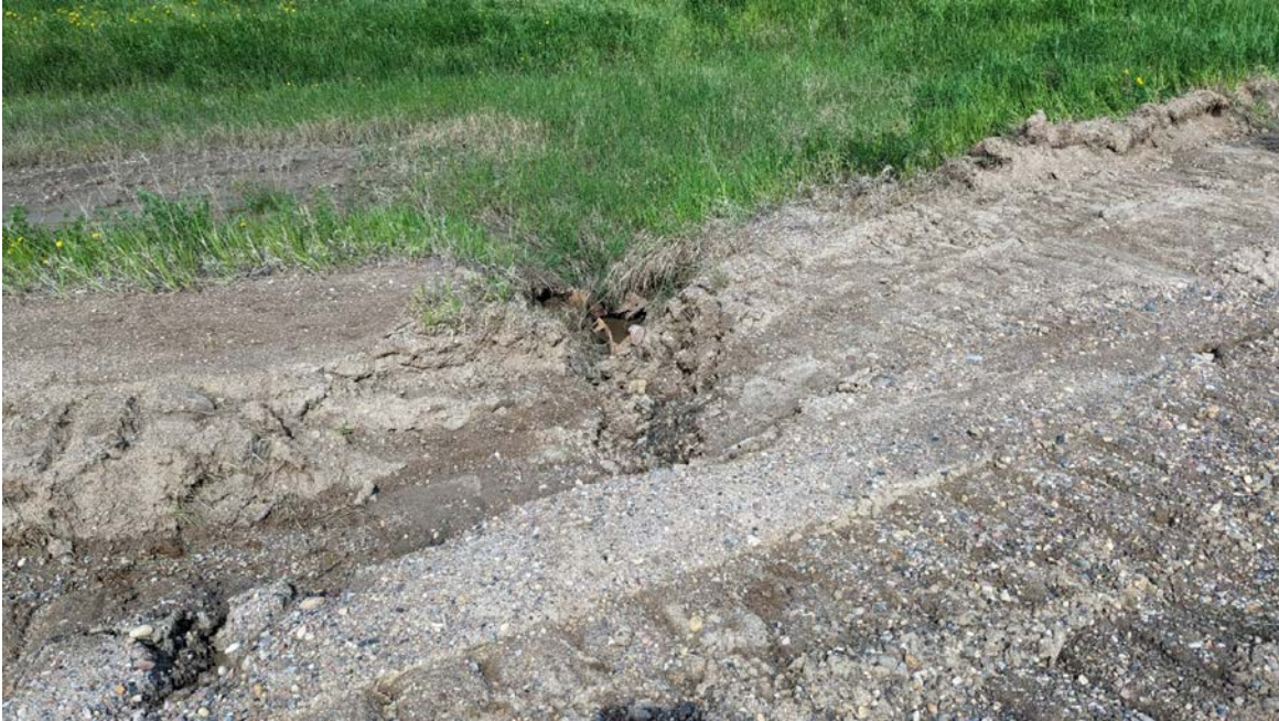
Photo 7 – Looking northwest at the partially visible inlet of only one of the twin culverts.
