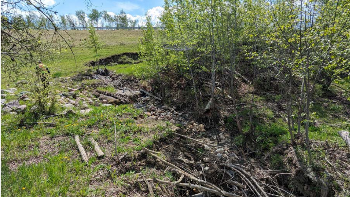
Photo 7 – Looking south where the erosion gully discharges into Gravina Creek.
