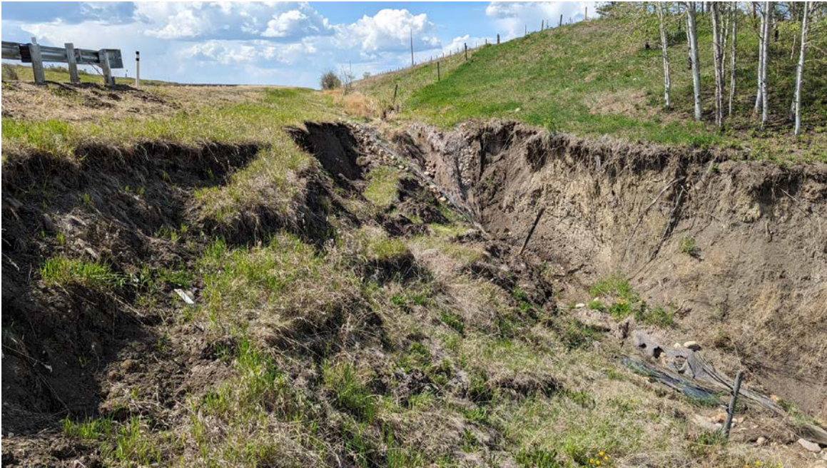
Photo 5 – Looking west at the nick point at the top of the erosion gully where the damaged gabion mattress and underlying nonwoven geotextile is exposed.
