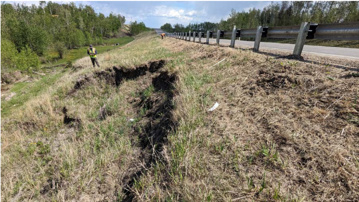
Photo 4 – Looking east where erosion gully slumping is closest to the highway.
