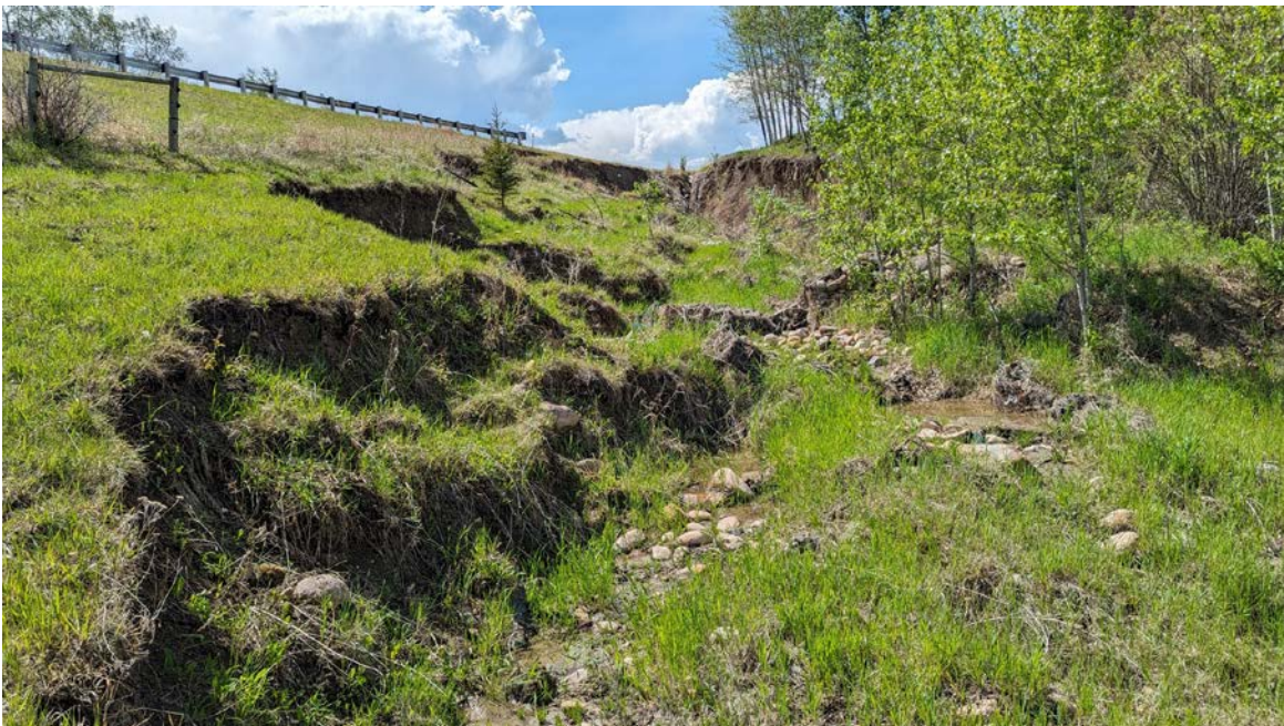
Photo 6 – Looking west near the bottom of the fill where remnants of a gabion basket check dam are visible on the right-hand side of the photo.
