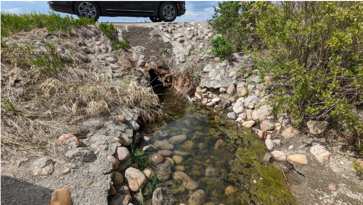
Photo 2 – Standing water at outlet of culvert at km 2.845 approach.
