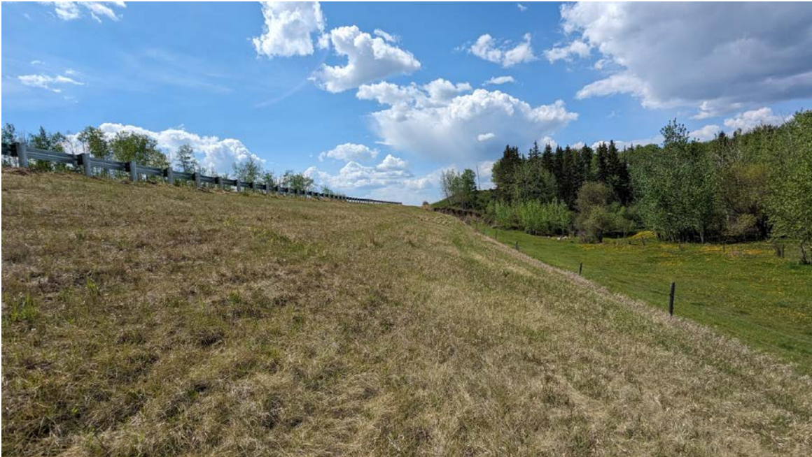
Photo 9 – Looking west along the north slope of the highway embankment fill which shows no evidence of slumping.
