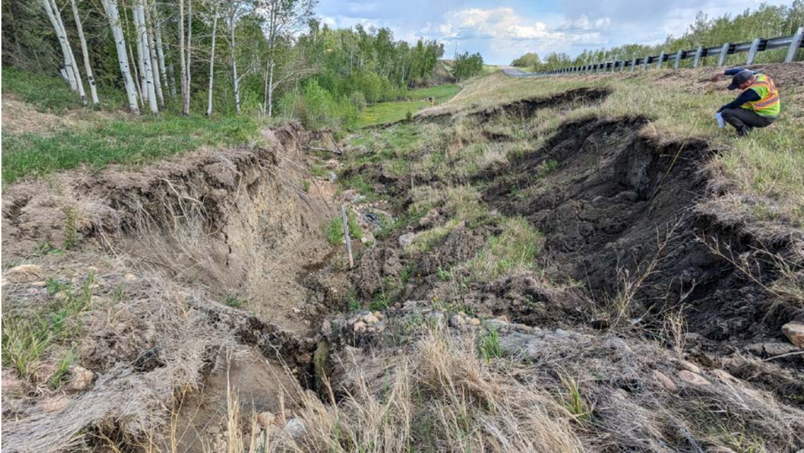
Photo 3 – Looking east at start of erosion gully in northwest corner of the highway embankment.
