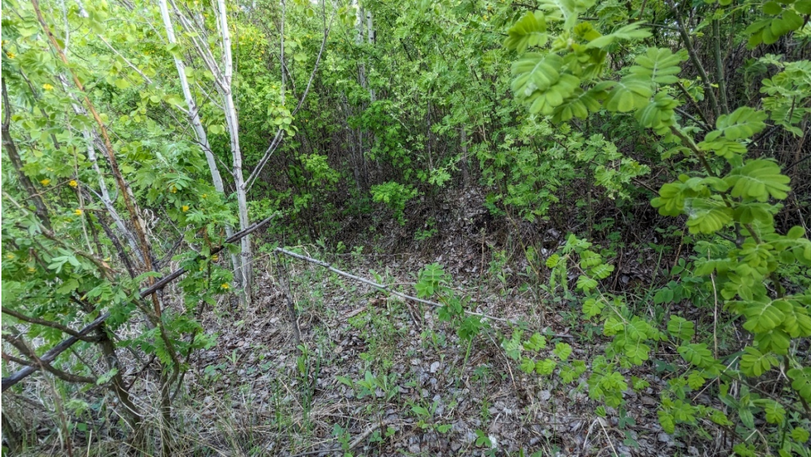
Photo 5 – Observed toe roll below the area of distress.
