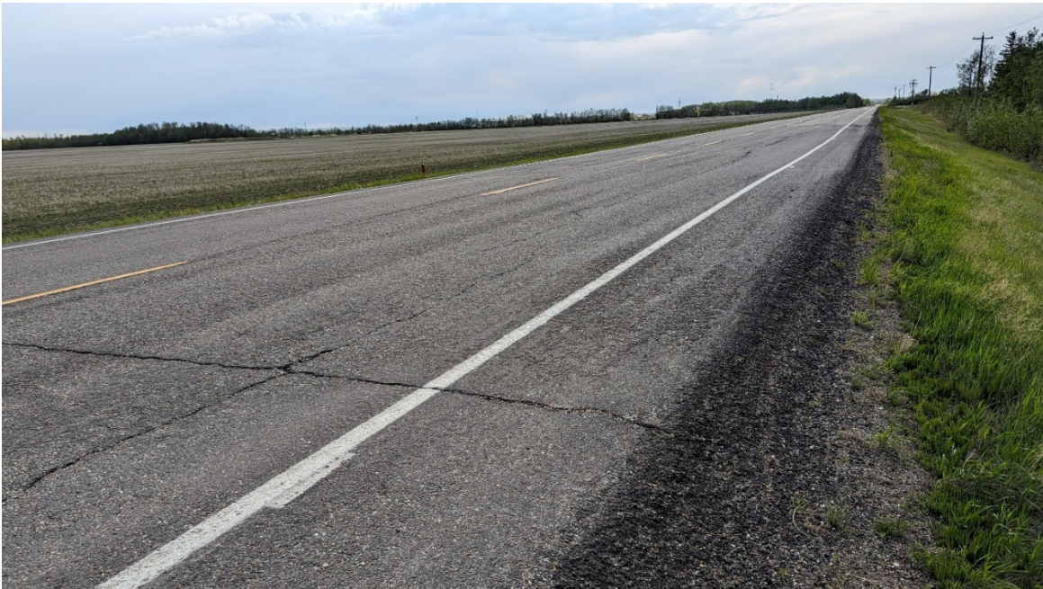
Photo 2 – Looking west at distressed area.
