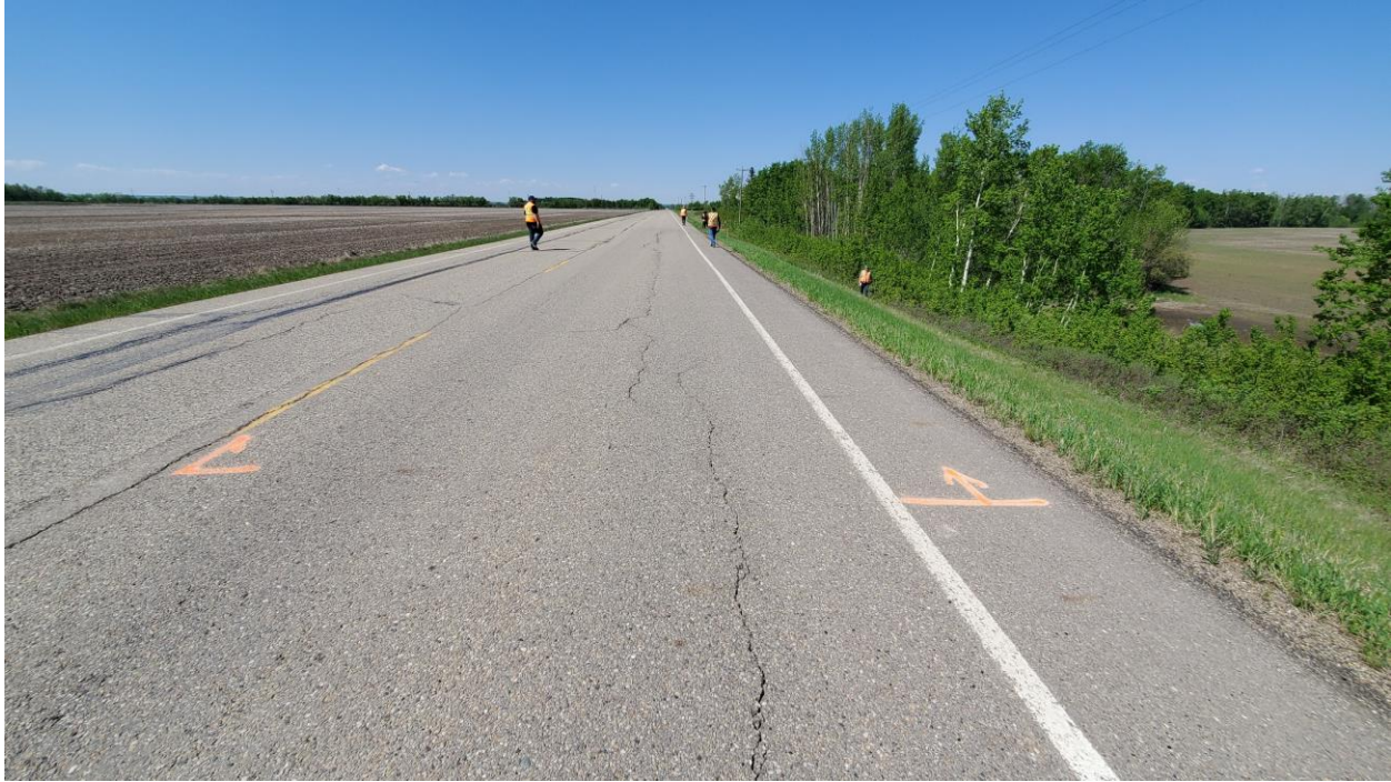
Photo 3 – Looking west at east of the proposed patch over the distressed area.
