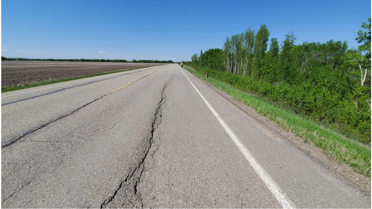
Photo 5 – Looking west at the main crack (taken west of Photo 4).
