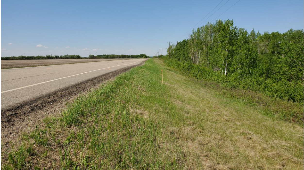
Photo 1 – Looking west over distressed area where dip is visible in the roadway surface and the stakes mark the planned patch.
