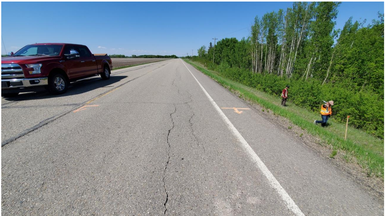
Photo 6 – Looking west at end of proposed patched and beyond the area of distress.
