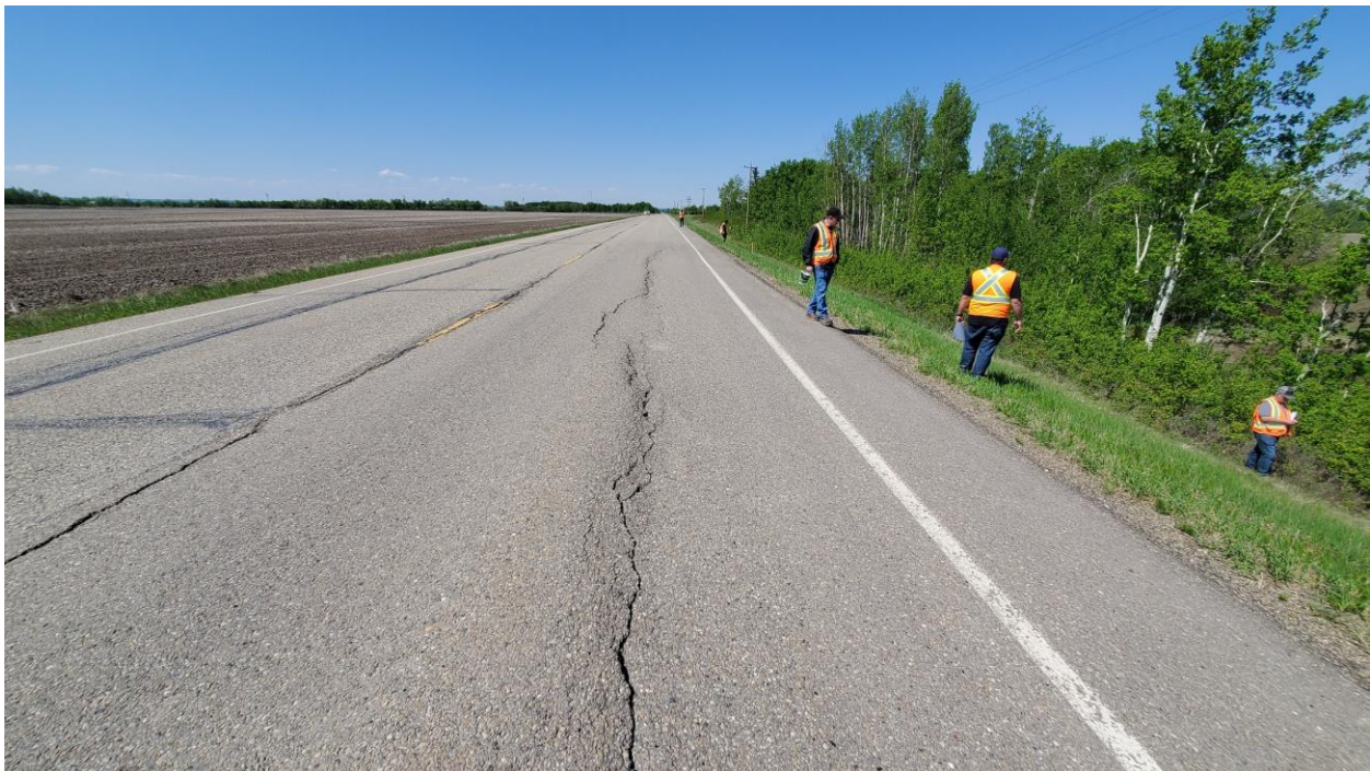
Photo 4 – Looking west at the central portion of the crack forming in the area of distress.
