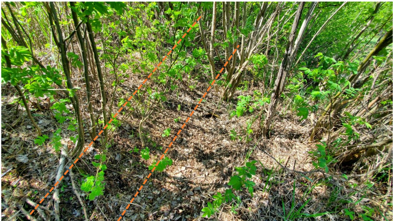
Photo 8 – Possible toe roll below the area of distress.
