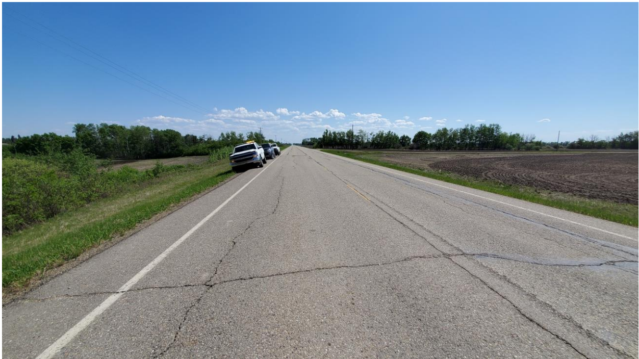
Photo 2 – Looking east beyond the area of distress.
