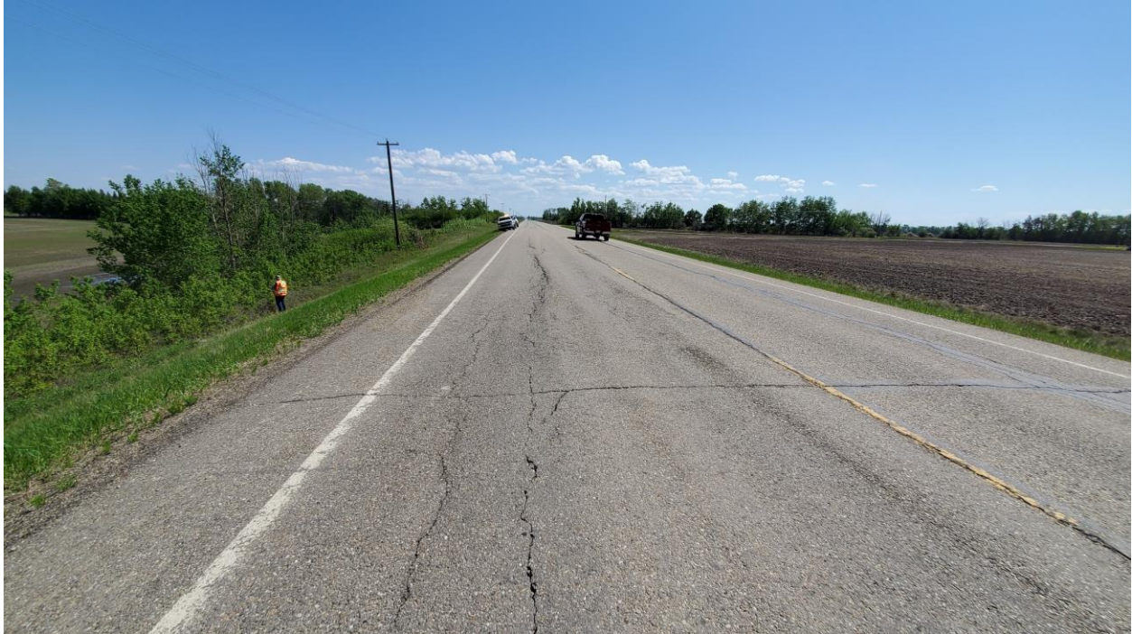
Photo 7 – Looking east from near the west end of the area of distress.
