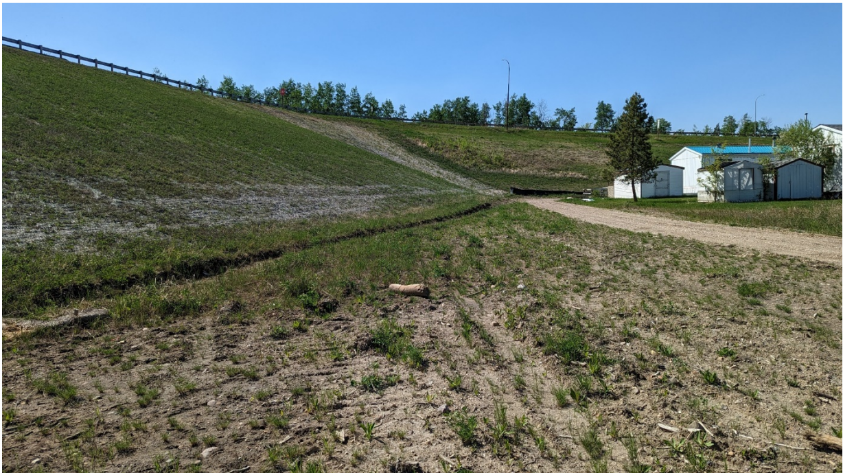
Photo 8 – Looking west along the toe of the Hwy 691 embankment where the Town cut a drainage channel which ties into the culvert outlet.
