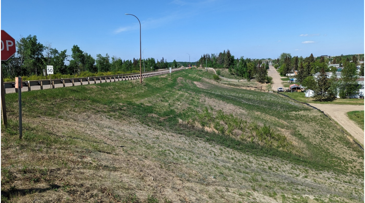
Photo 1 – Looking north toward the slide repaired on the east side of Hwy 35.
