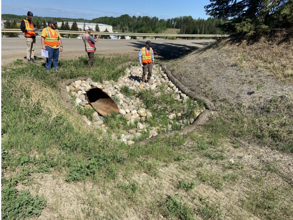
Photo 5 – New SWSP inlet in the east ditch of Hwy 35 on the south side of Hwy 691.
