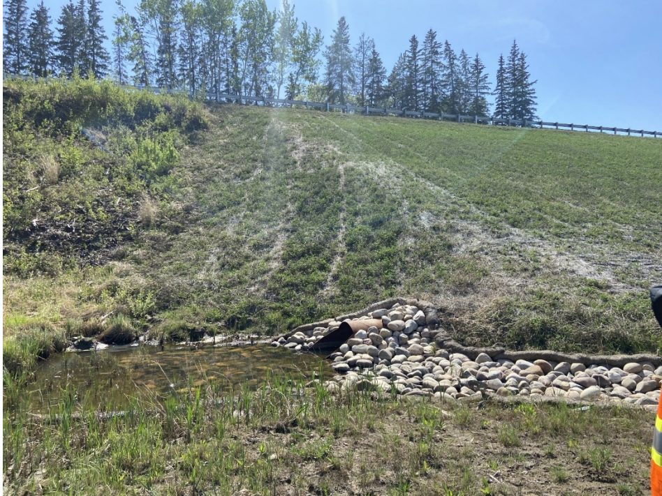
Photo 7 – Looking south at the outlet of the 750 mm SWSP with the wetland to the left.
