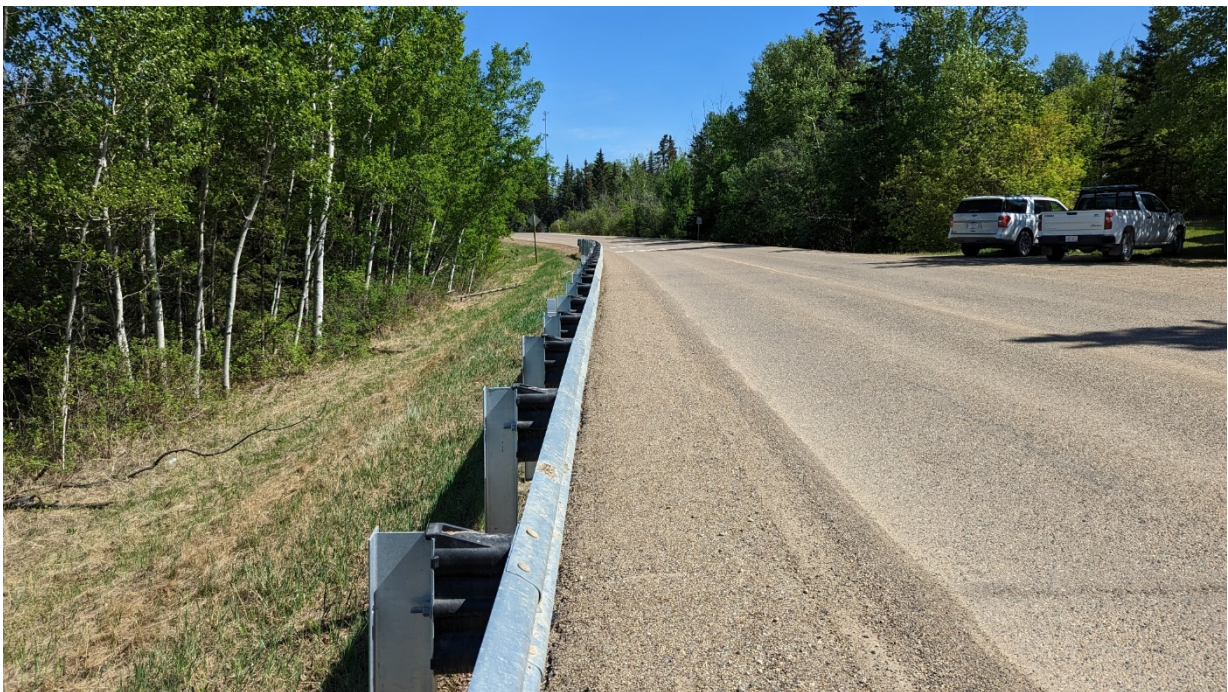
Photo 4 – Looking east along Hwy 691 at the east end of the site where the guardrail was extended by the Maintenance Contractor.
