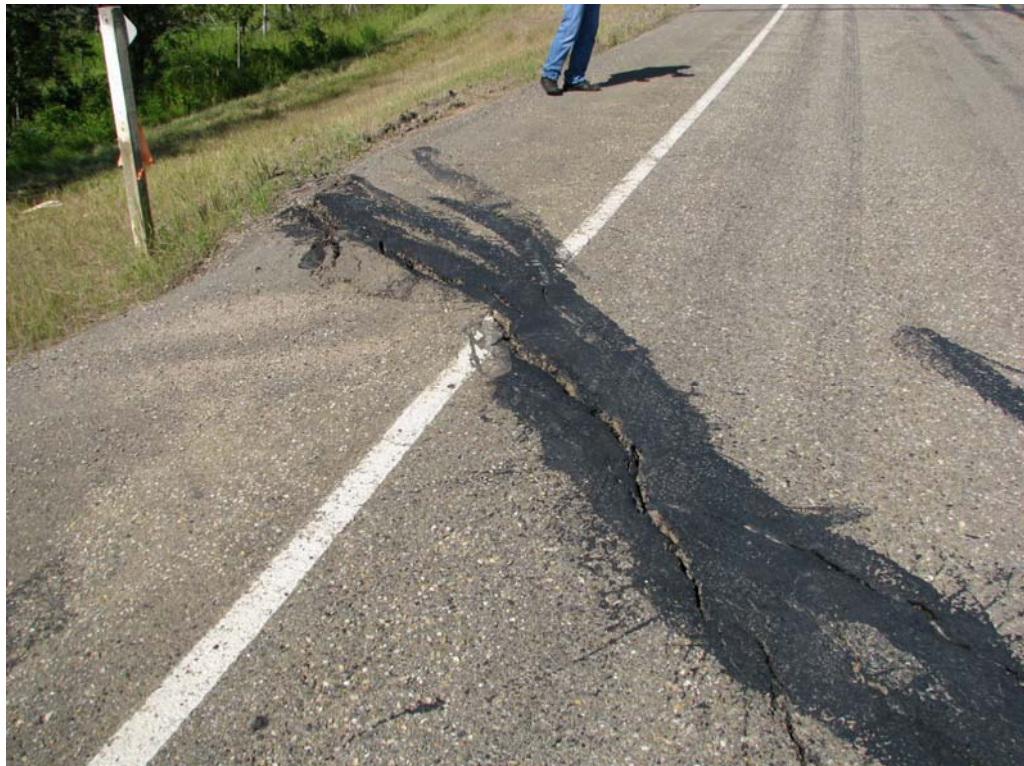
Photo 4 – View of asphalt crack and dip
