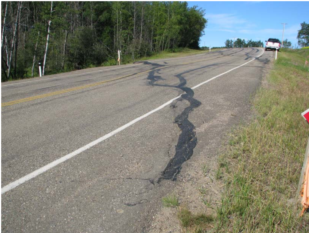
Photo 2 – View of the crack on the highway and asphalt thickness, looking southwest.
