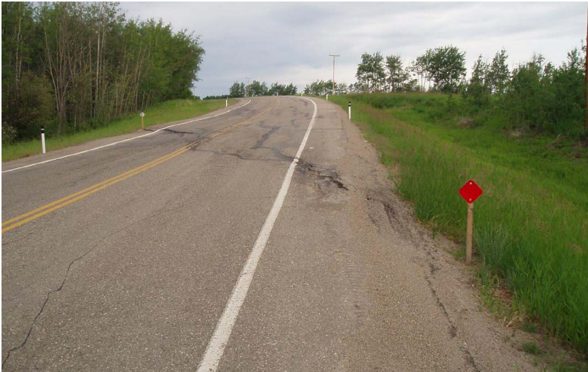
PHOTO 1: Looking west along Hwy 690:02 at the active backscarp location
