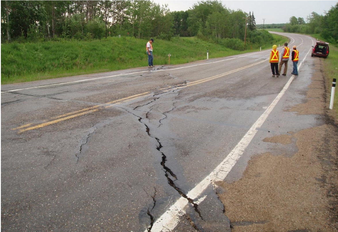
PHOTO 2: Looking east along Hwy 690:02 at the active backscarp location
