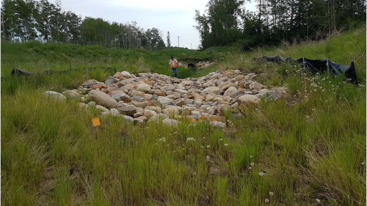
Photo 5 – Looking east from lined swale at bare spot between the swale and riprap apron where vegetation growth has been slowly improving.
