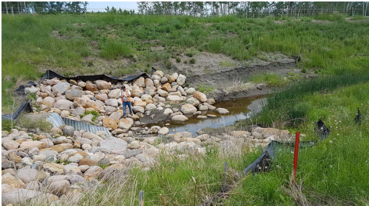
Photo 4 – Looking west at bare area at culvert outlet where possible tension cracks may be forming. Subdrain outlet is just on the far side of the culvert outlet. Note the eroded bare spot just beyond the riprap.
