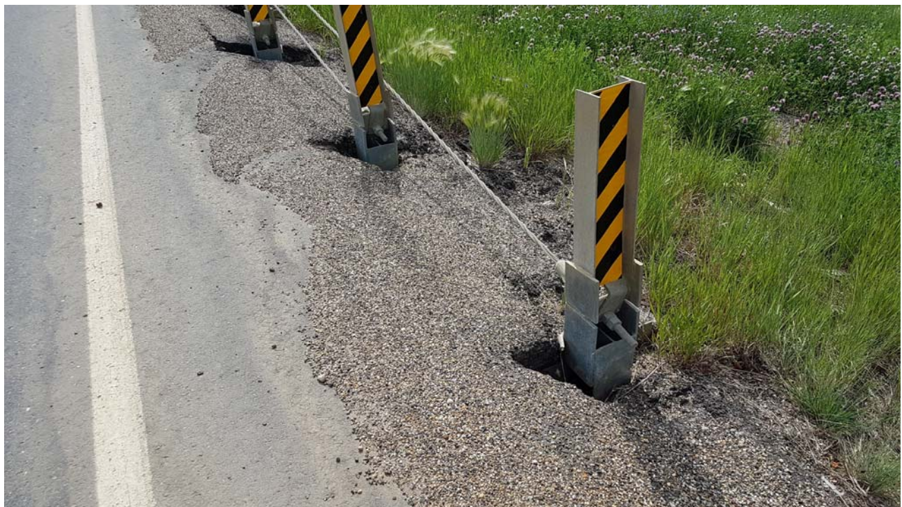
Photo 2 – Looking at voids around HTSCB on south side of highway at the west end.
