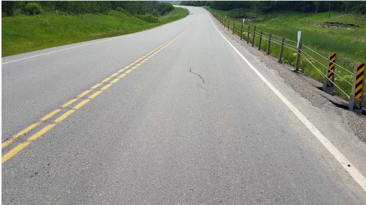
Photo 3 – Looking east at small crack at west end of slide area near the end of the HTSCB.
