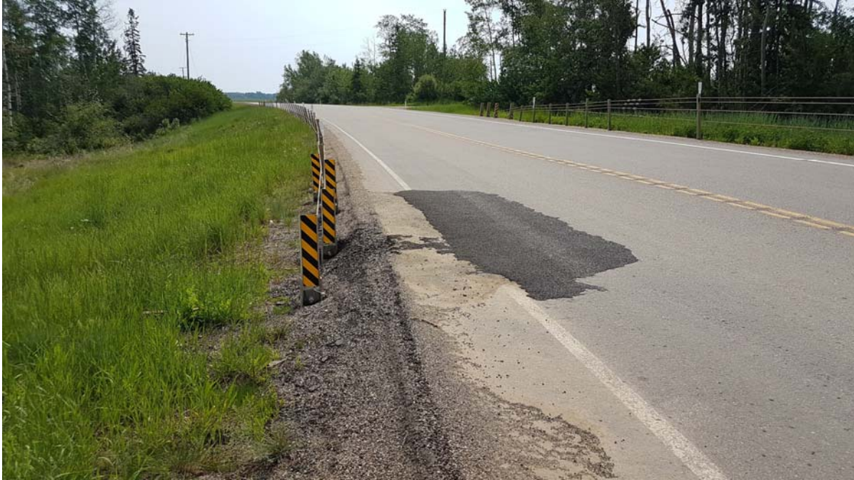
Photo 7 – Looking east at voids around HTSCB posts and settlement cracking of the pavement at west end of the north barrier located by the outlet of BF72371 culvert. Note that two patches have been required in this area.
