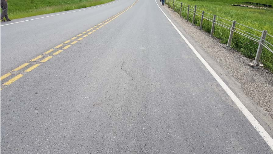
Photo 3 – Looking east at small crack at west end of slide area near the end of the HTSCB.
