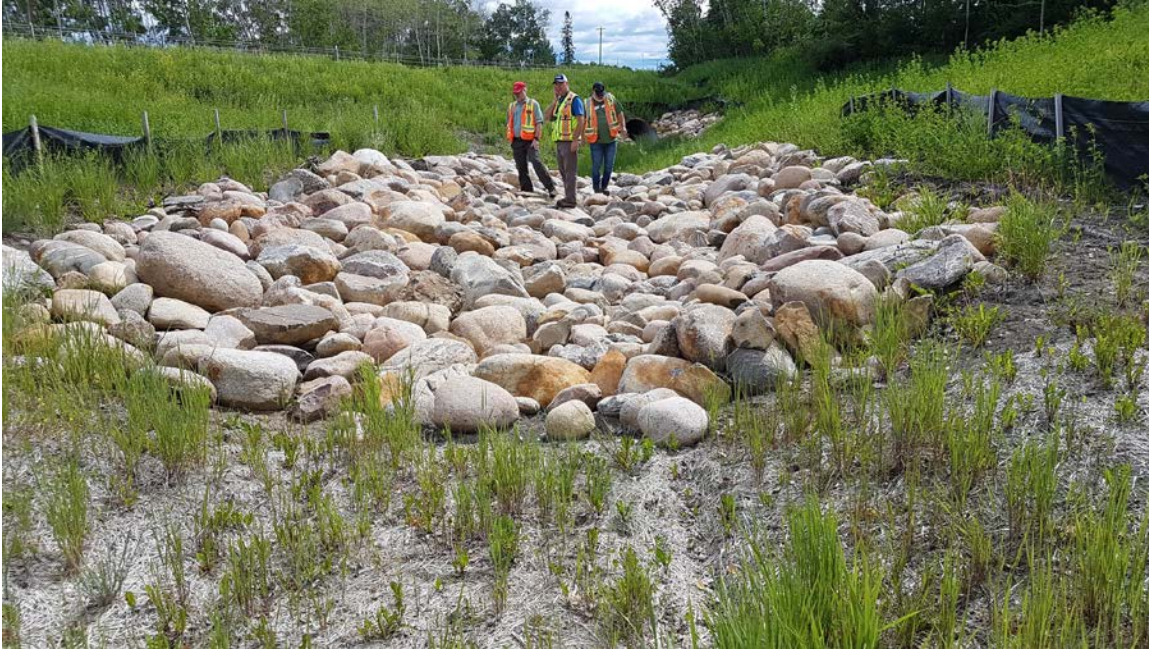
Photo 5 – Looking east from lined swale at bare spot between the swale and riprap apron.
