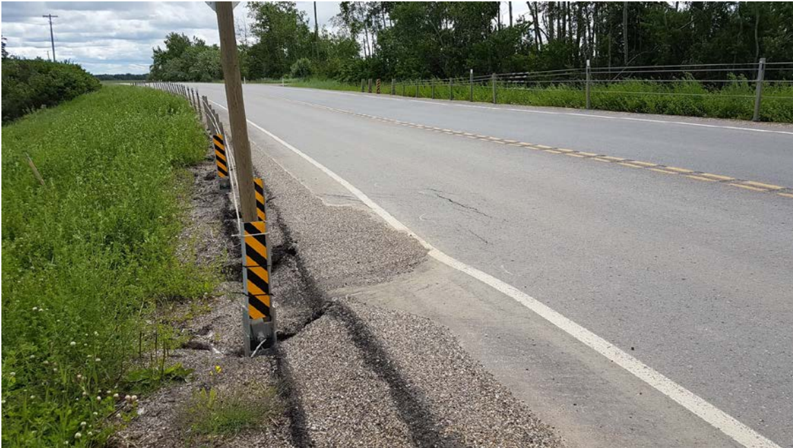
Photo 7 – Looking east at voids around HTSCB posts and settlement cracking of the pavement at west end of the north barrier located by the outlet of BF72371 culvert.
