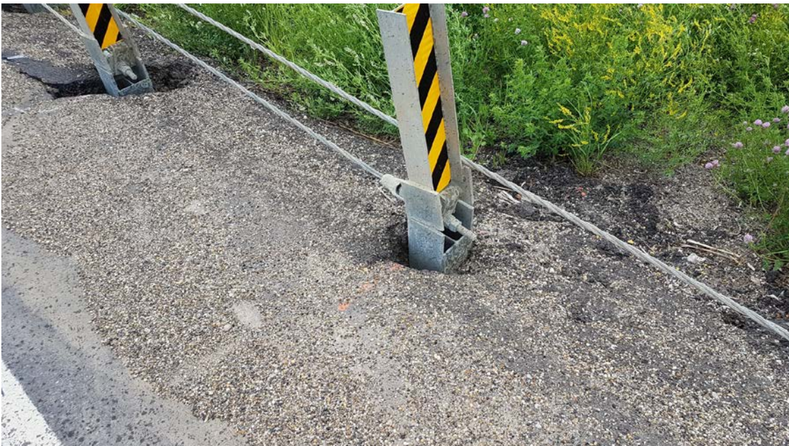
Photo 2 – Looking at voids around HTSCB on south side of highway at the west end.
