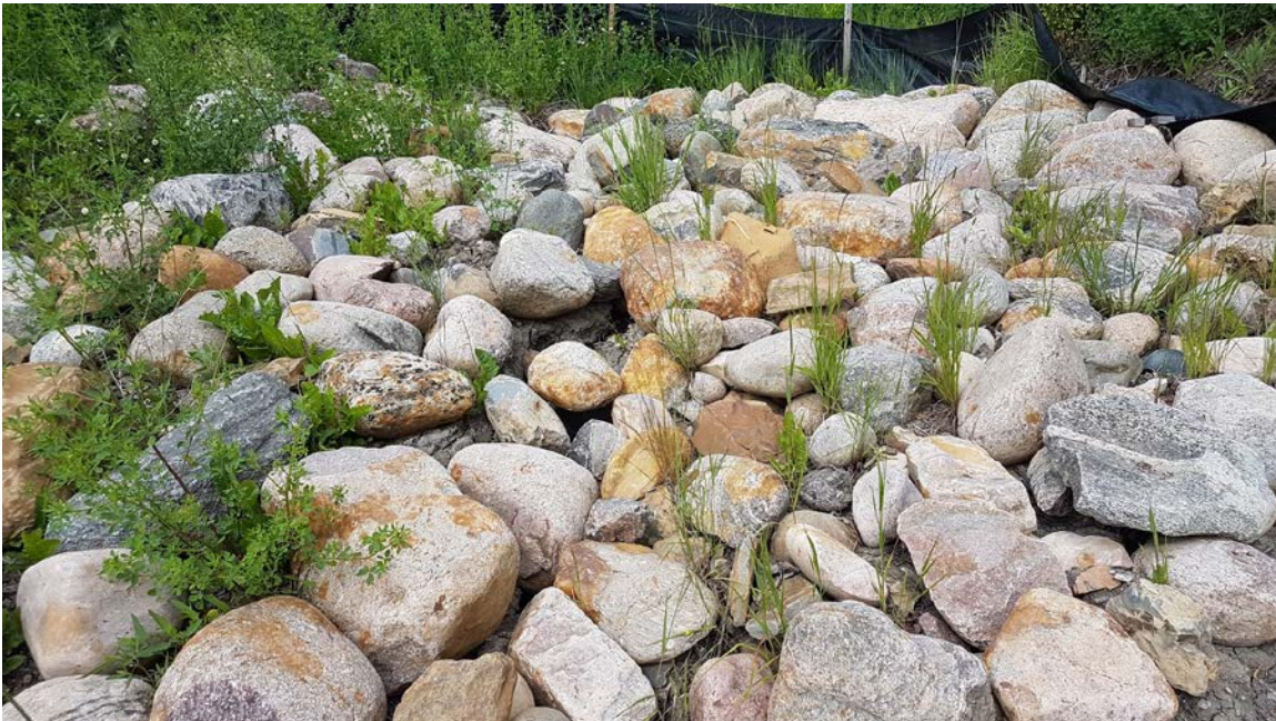
Photo 8 – Looking at riprap placed over bare ground (no nonwoven fabric below) at east end of north ditch the outlet of BF72371.
