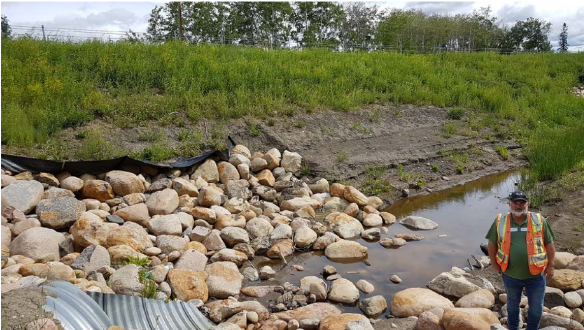
Photo 4 – Looking west at bare area at culvert outlet where possible tension cracks may be forming. Subdrain outlet is just on the far side of the culvert outlet.
