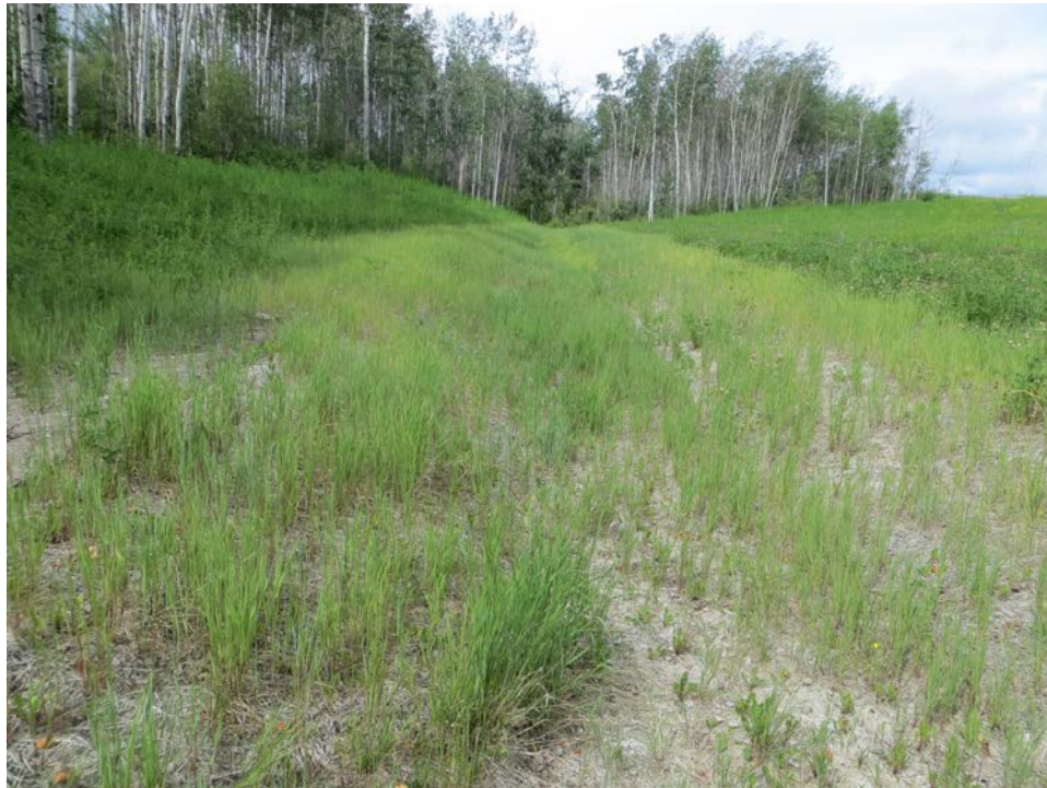
Photo 6 – Looking west along lined swale located at the south end of the toe berm.
