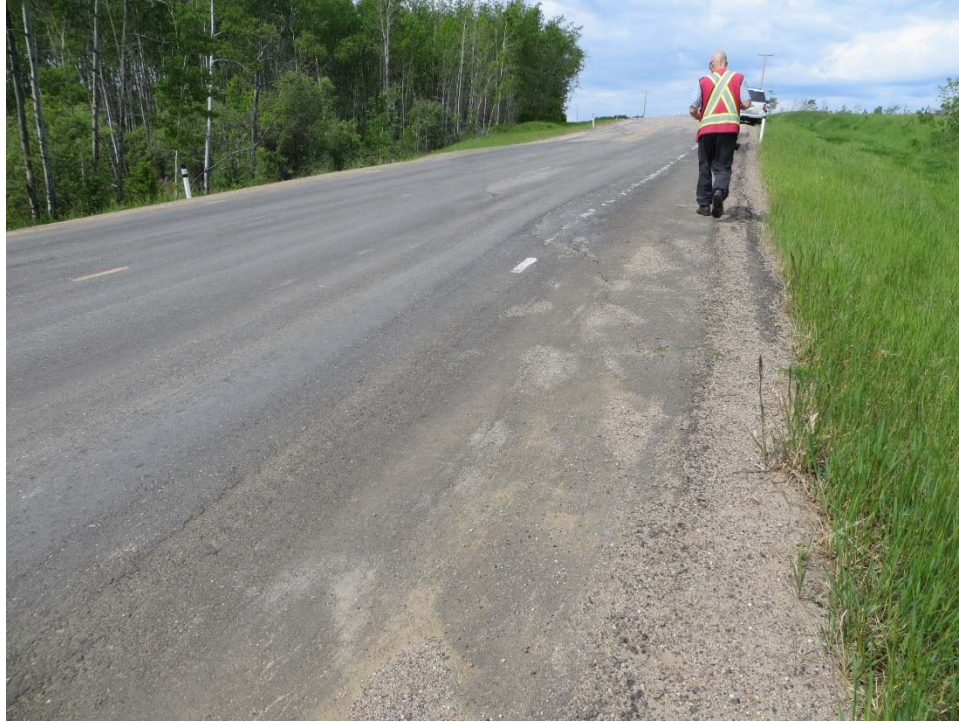
Photo 3 – Looking west at west portion of crack and recent patch.
