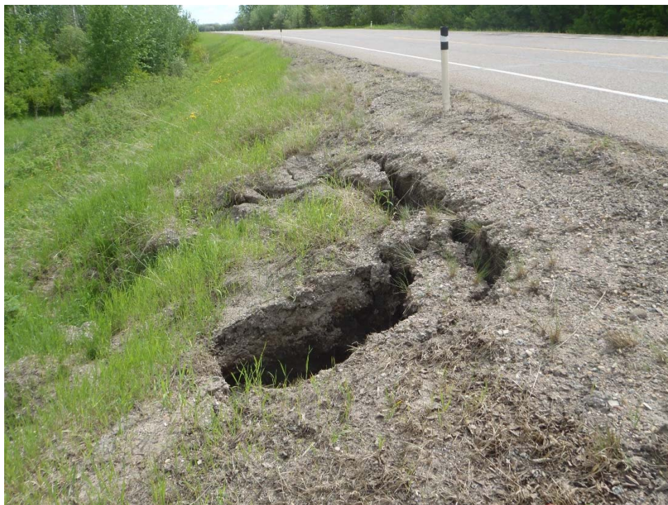
Photo 4 – Slumping at the culvert outlet on the north side of the highway.
