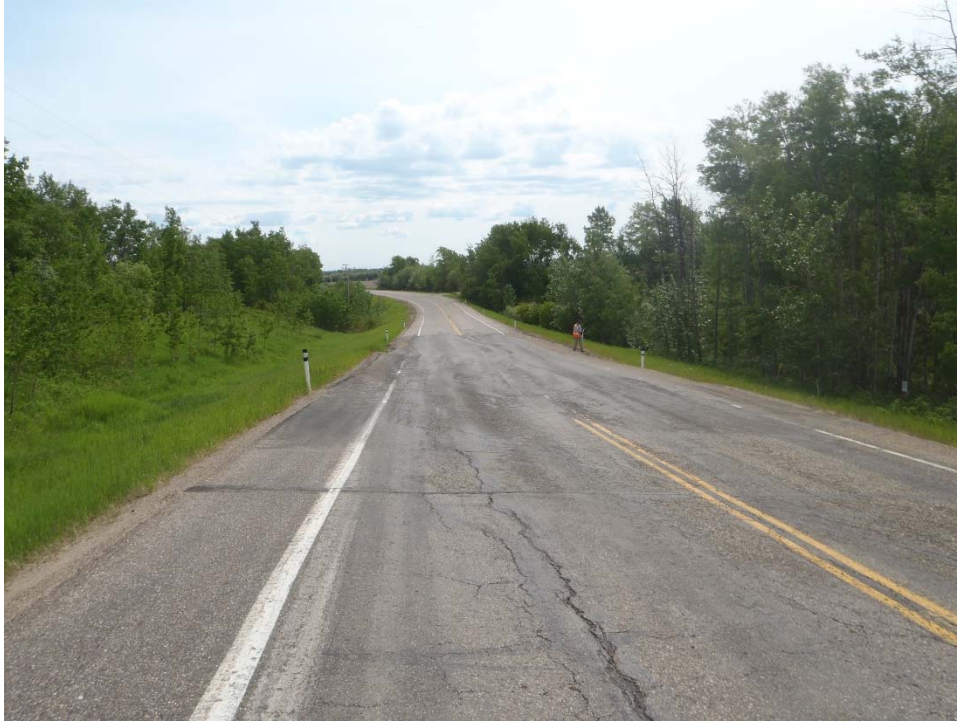
Photo 1 - View of Highway 690 showing the 2011 ACP patch, looking east.
