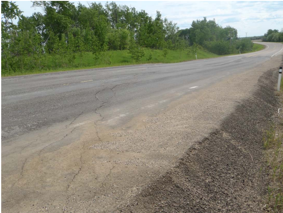
Photo 2 – View of the crack and asphalt thickness, looking northeast. The dip in the highway surface can be seen in the centre of the patch
