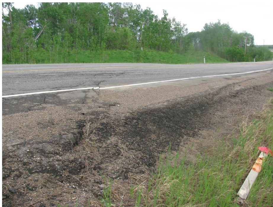
Photo 4 – View of asphalt thickness and crack
