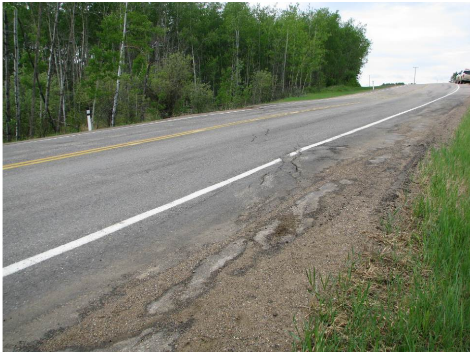
Photo 2 – View of the crack on the highway and asphalt thickness, looking southwest.
