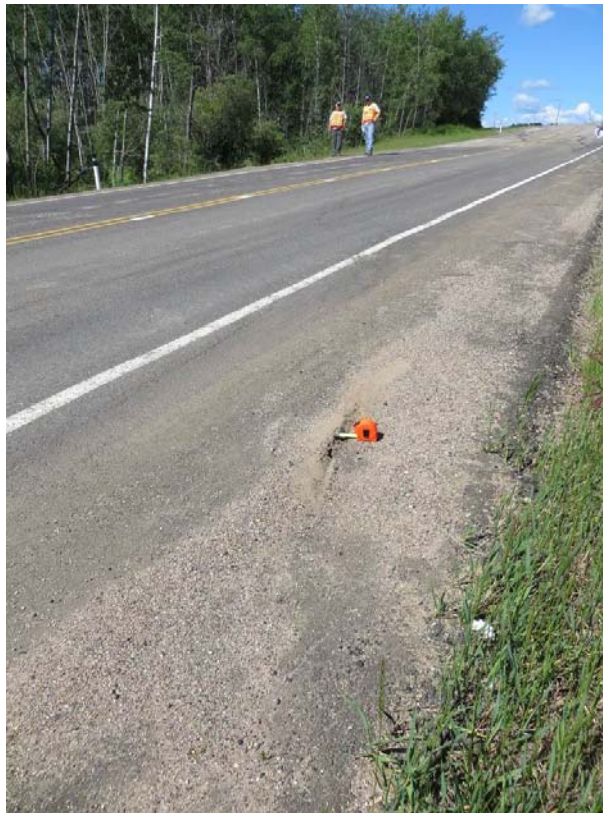
Photo 2 – View of the crack on the highway and asphalt thickness, looking southwest.
