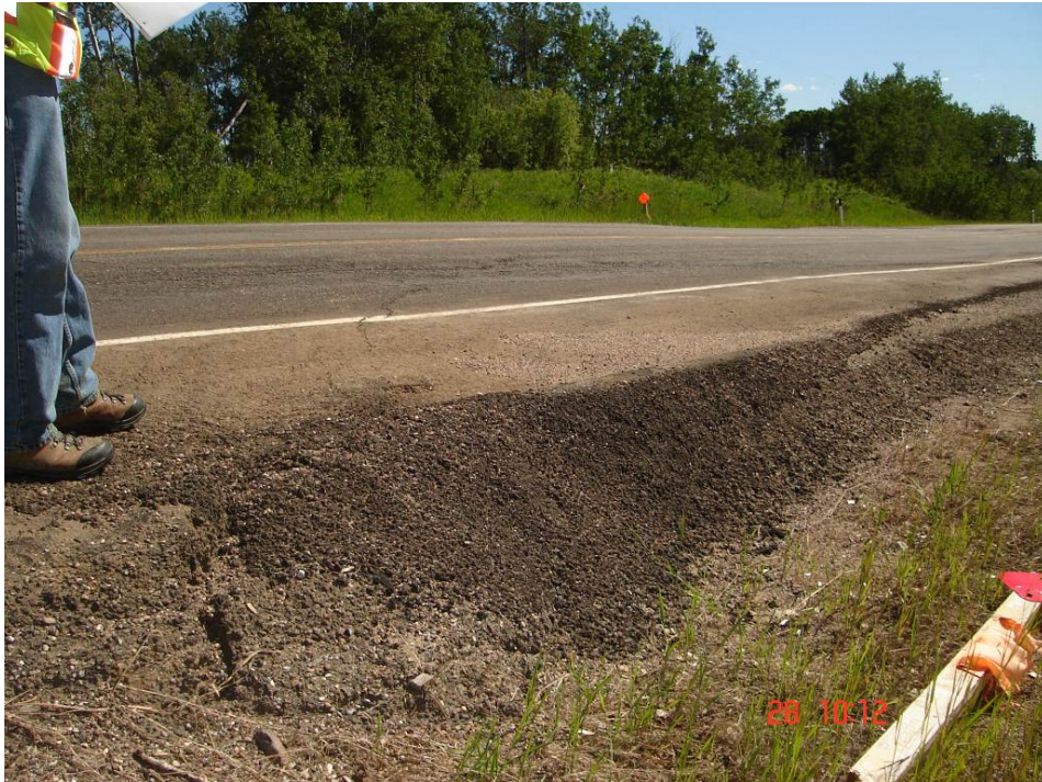
Photo 4 – View of asphalt thickness and crack
