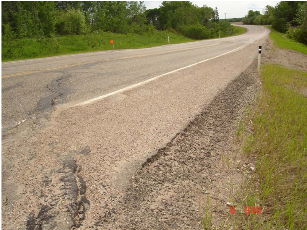
Photo 2 – Increased cracking on pavement looking southwest.
