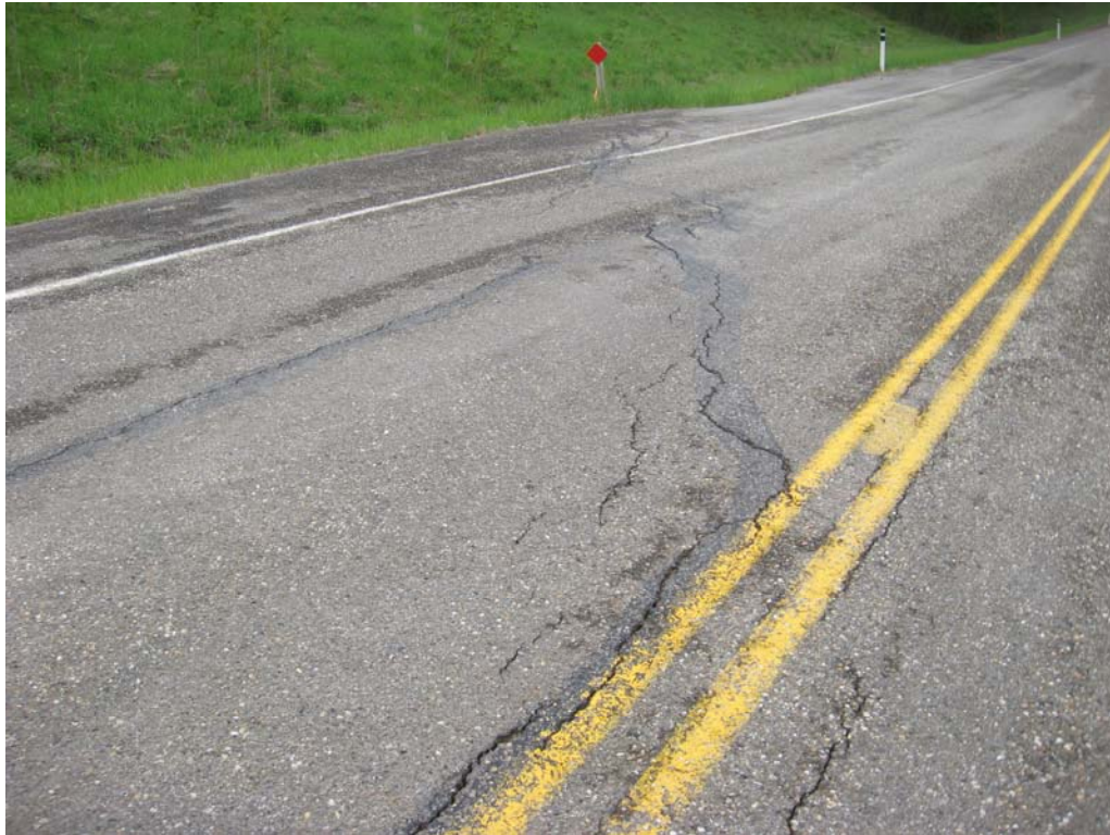
Photo 3 – Increased cracking on pavement looking southwest.
