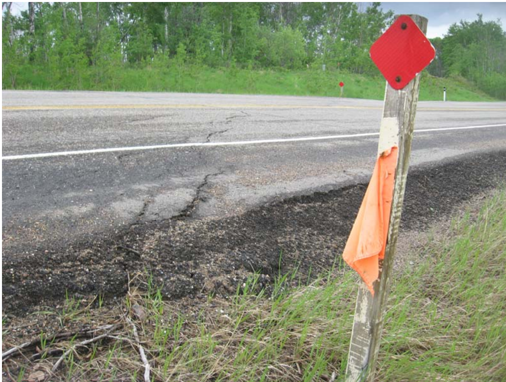
Photo 2 – View of the crack on the highway and asphalt thickness, looking northeast.
