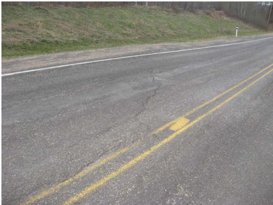
Photo 2 - View of crack reflecting through 2008 ACP patch, looking northeast.
