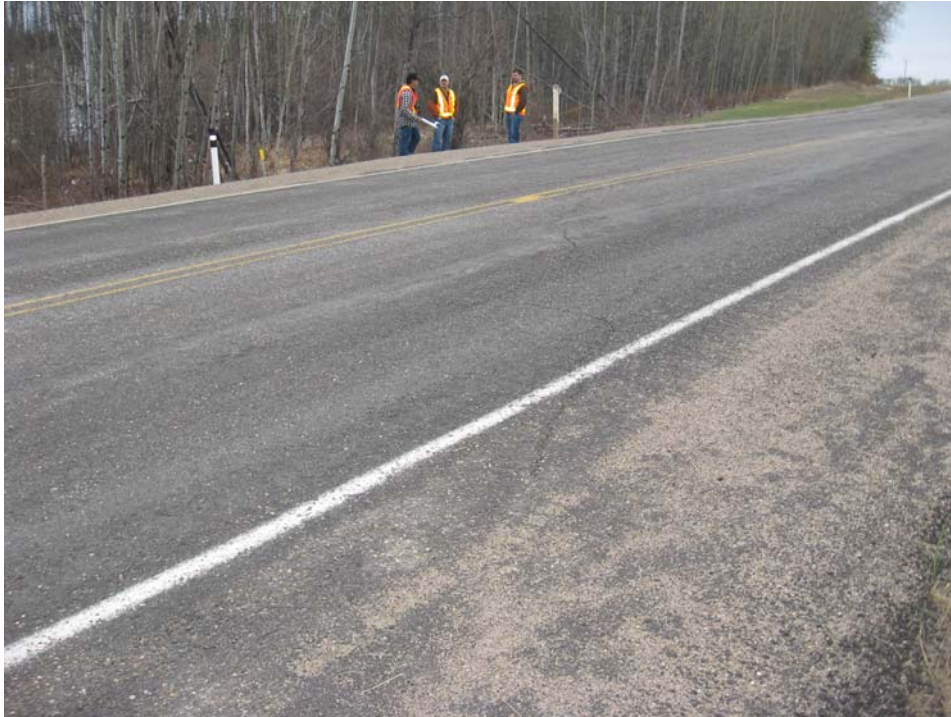
Photo 3 - View of crack reflecting through 2008 ACP patch, looking southwest.
