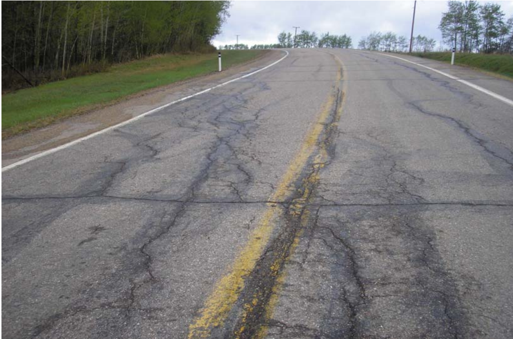
PHOTO 5 - View of extended and widened cracks facing west.
