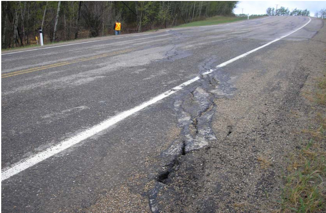
PHOTO 3 - View of active slide scarp across the roadway surface, facing west.
