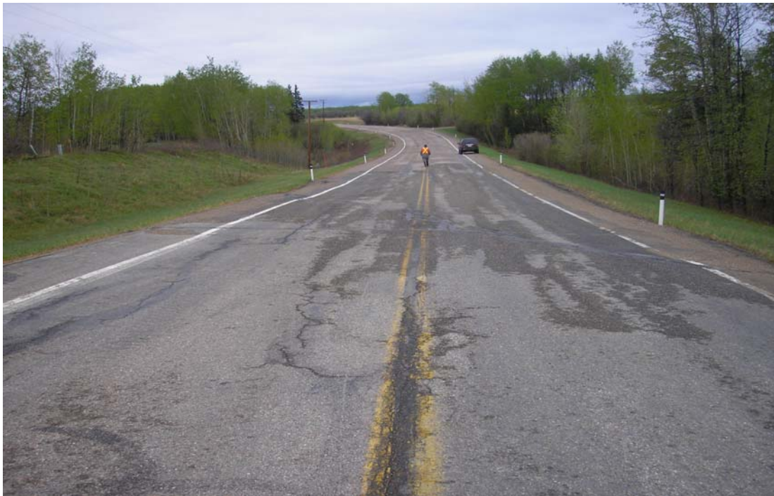
PHOTO 6 - View of Highway 690 facing east, showing a dip in the pavement.
