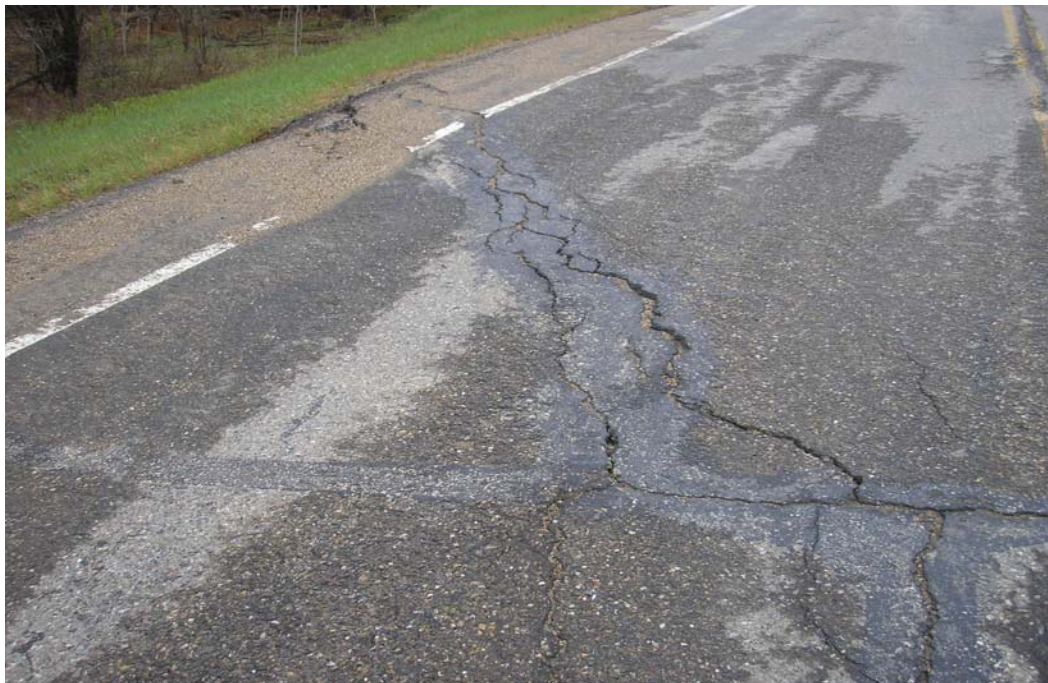
PHOTO 4 - View of active slide scarp across the roadway surface, reaching the south shoulder, facing southwest.
