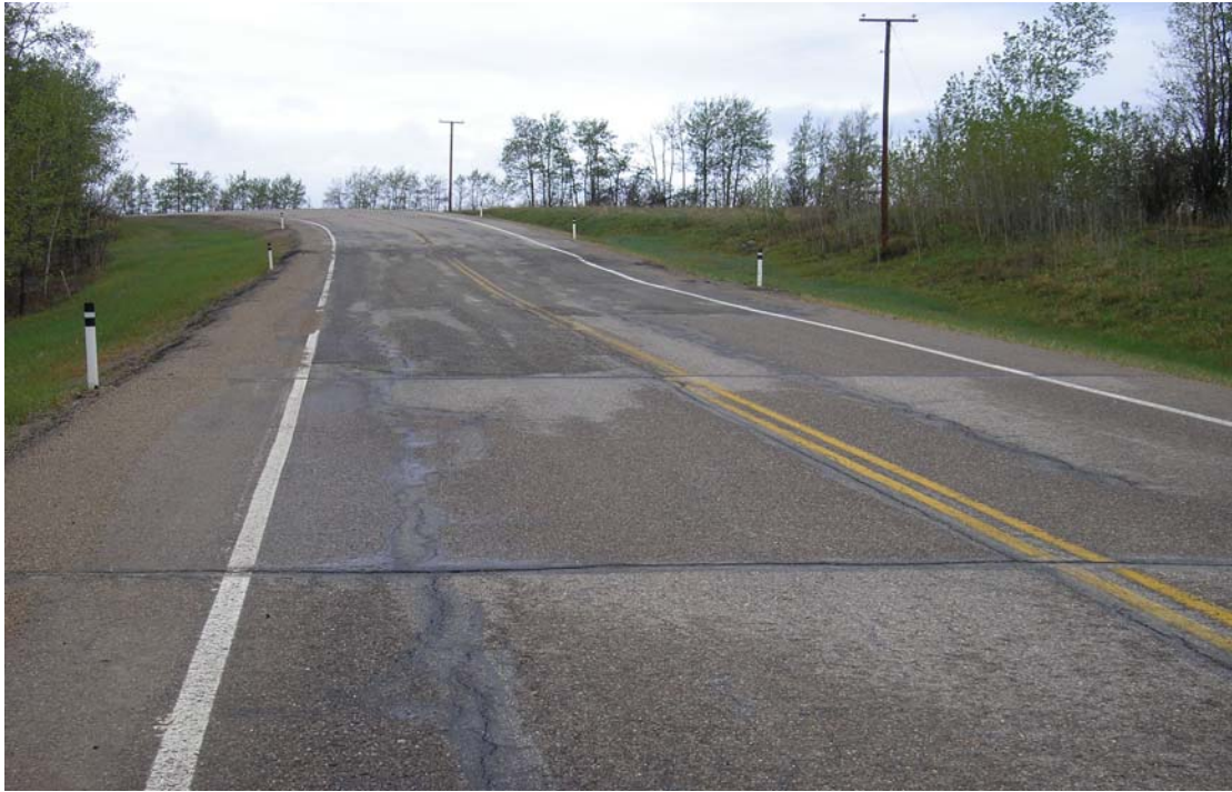
PHOTO 1 - View of Highway 690 facing west, showing a dip in the pavement.
