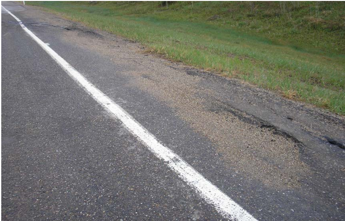
PHOTO 2 - View of slide scarp reaching the north shoulder and turning towards the east, penetrating again into the westbound lane.
