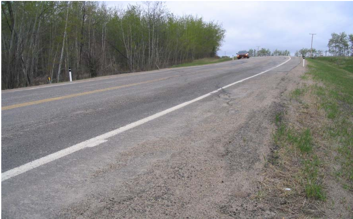
Photo 1 - View of active slide scarp across the roadway surface, facing west.
