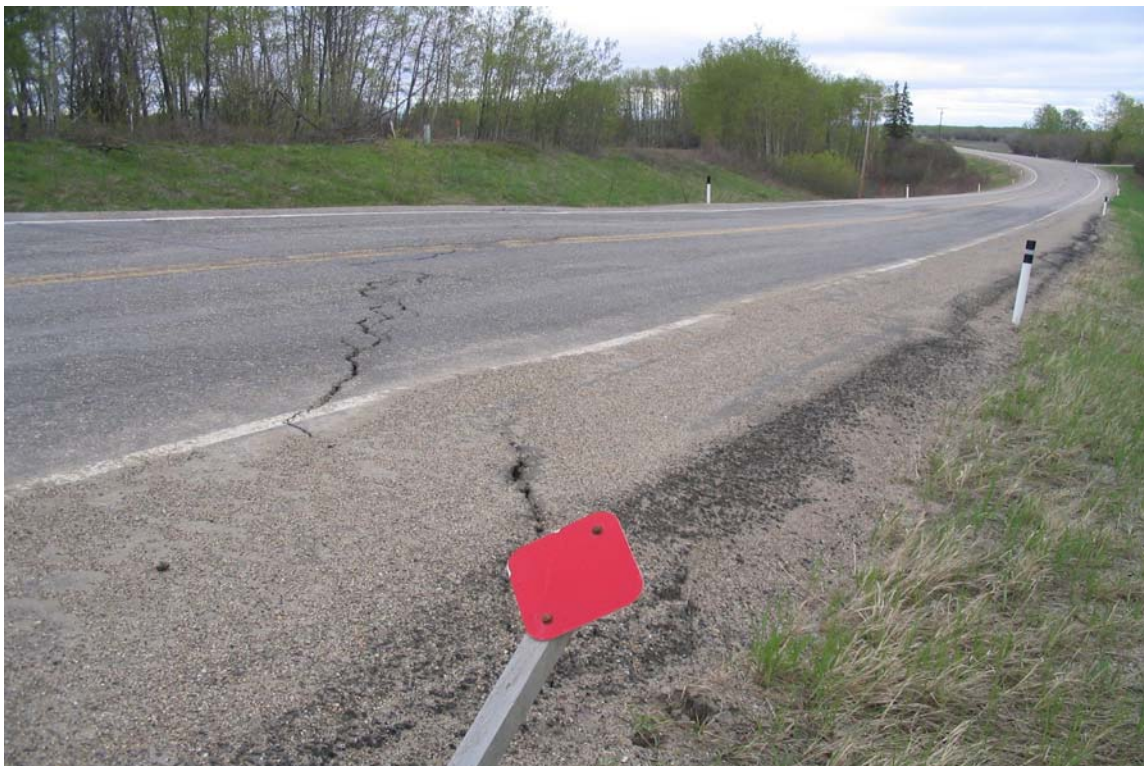
Photo 2 - Cracks reopening through Fall 2005 ACP patch.
