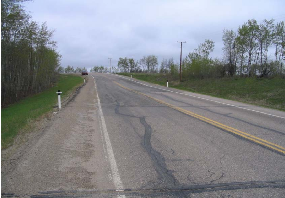
Photo 3 - View of Highway 690 facing west, showing a dip in the pavement.
