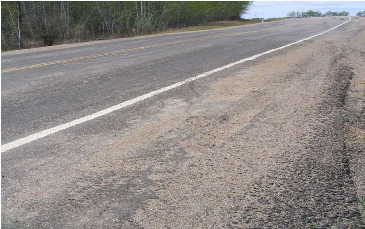
PHOTO 1: Cracks re-opening through Fall 2005 ACP patch.
