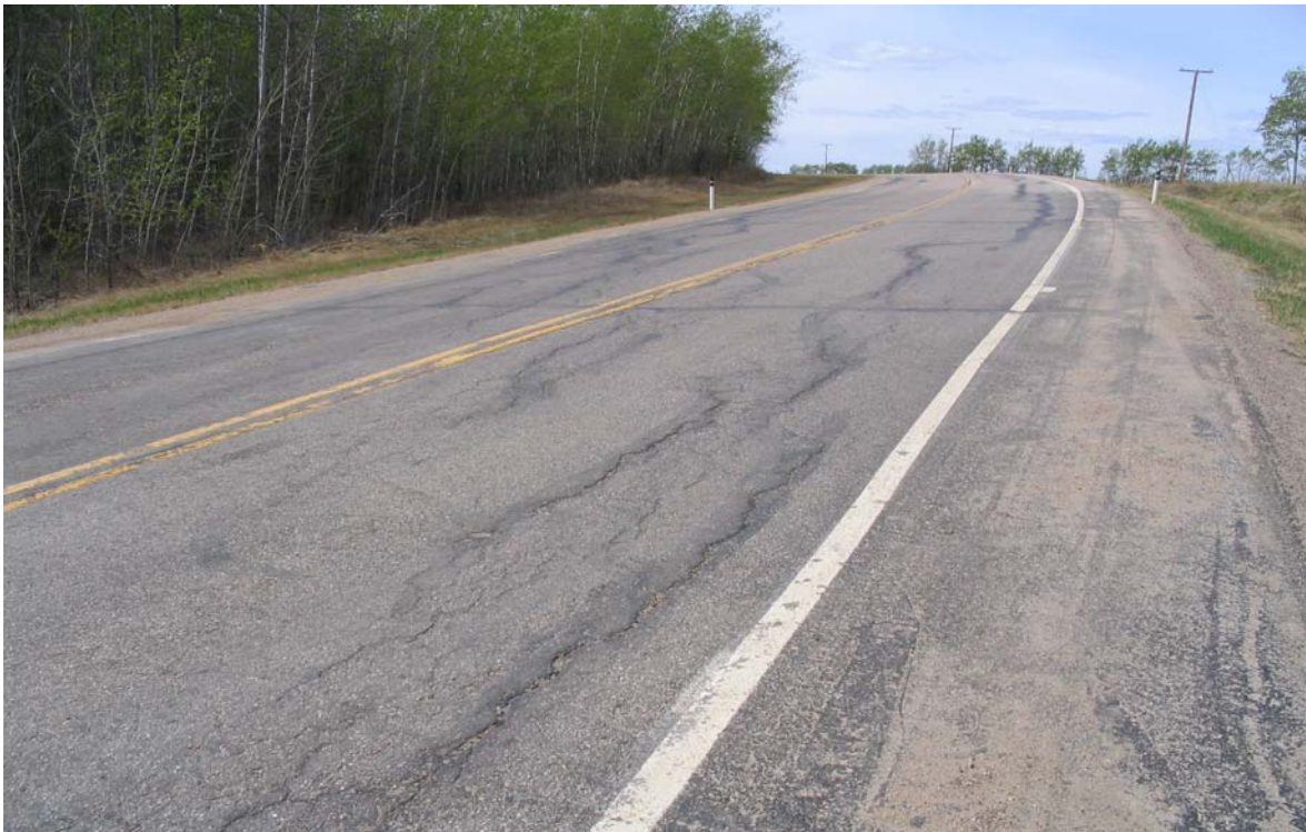
PHOTO 2: Stretch cracks at west end of slide.
