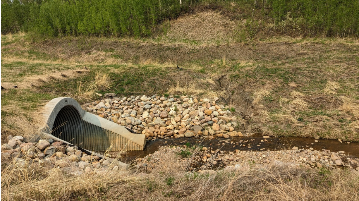
Photo 6 – Looking north at erosion gully on the north side of the culvert inlet.
