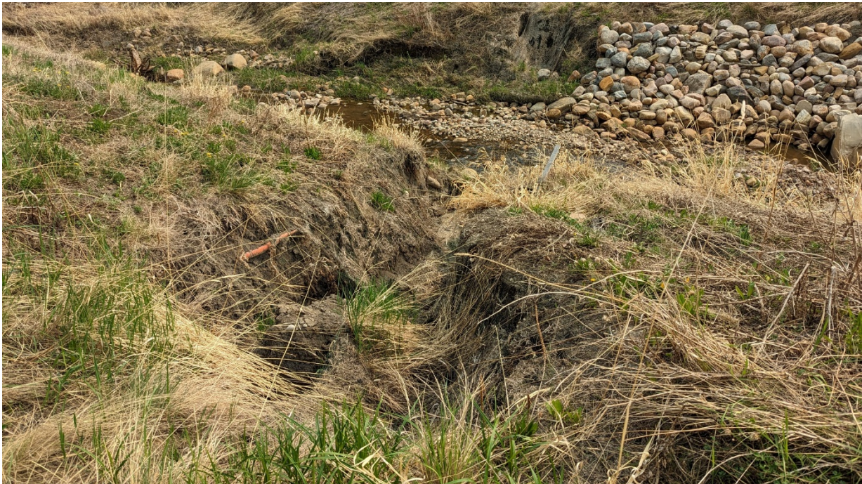
Photo 7 – Looking south at the north erosion gully (far side of Photo 6) and south erosion gully (far side of this photo) at the culvert inlet.
