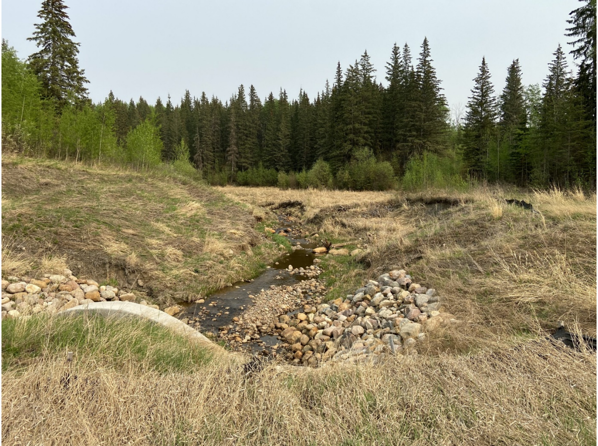
Photo 8 – Looking east at slumping forming upstream of the culvert inlet.
