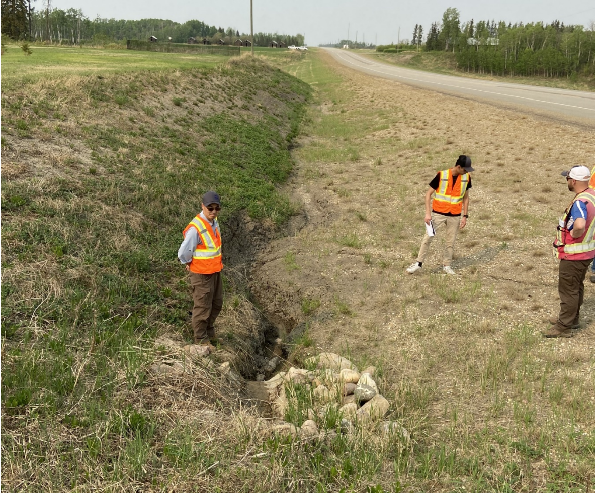
Photo 5 – Looking north at erosion gully forming below the outlet of an approach culvert in the west ditch south of the bridge culvert.
