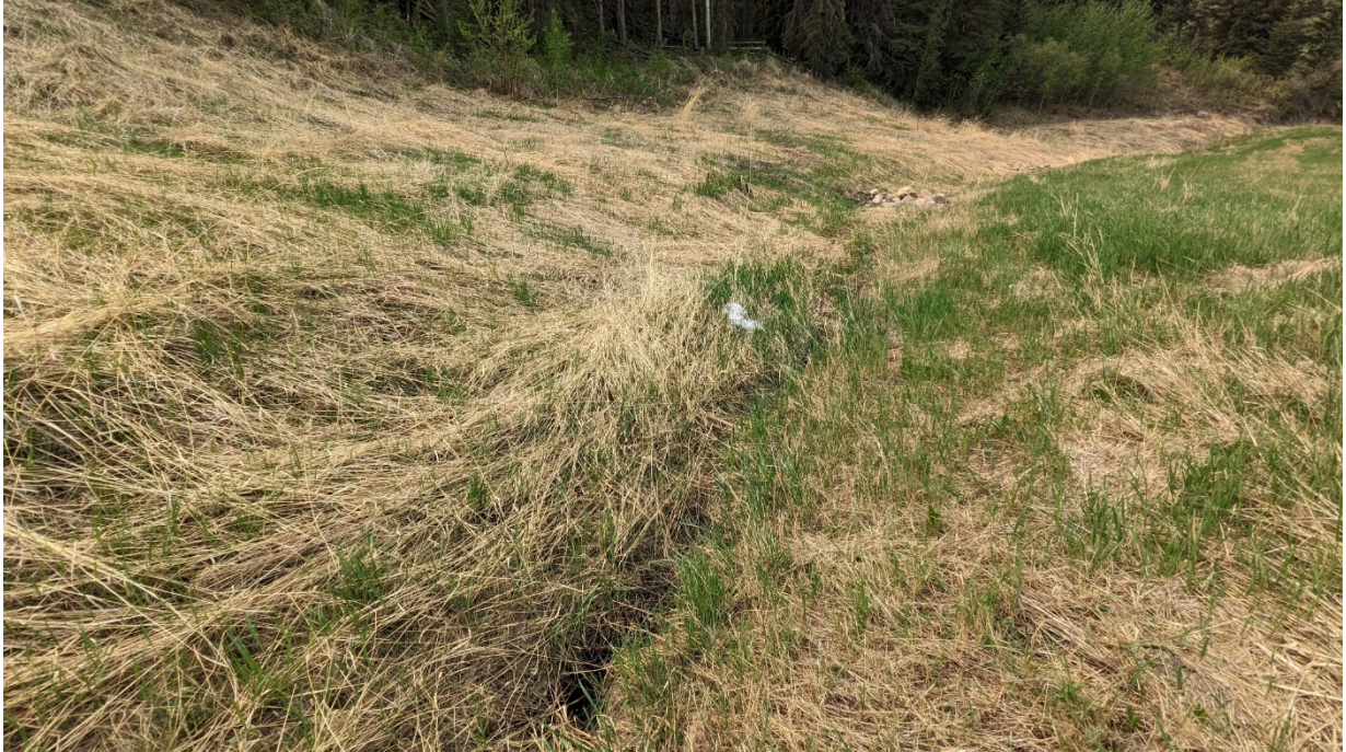
Photo 3 – Looking west at erosion gully forming in SW quadrant ditch.
