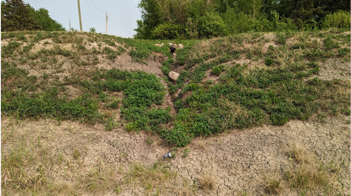
Photo 9 – Looking east at erosion gully forming below private landowner culvert on the east side of the ditch north of bridge culvert.
