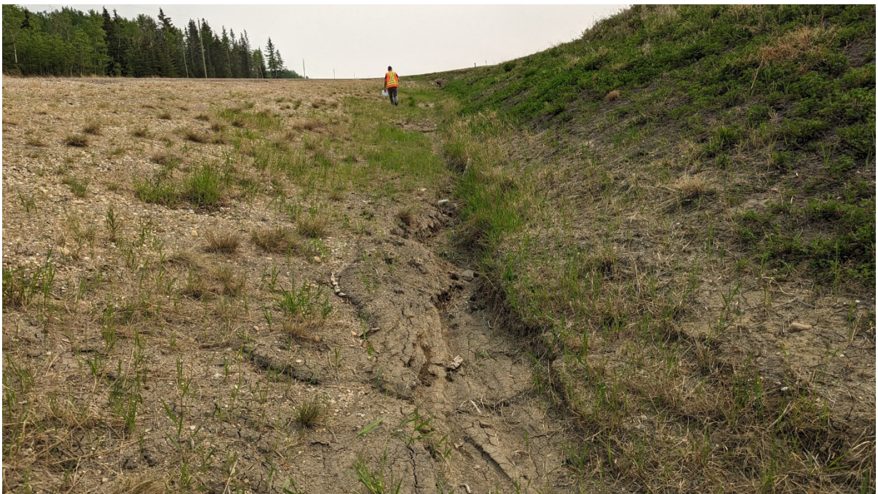
Photo 4 – Looking south at eroding west ditch.
