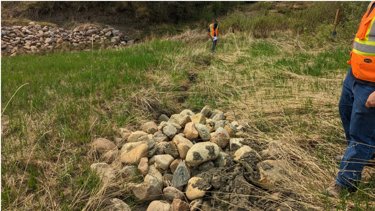
Photo 2 – Looking west at a riprap cluster and erosion gully in lower half of NW quadrant ditch.
