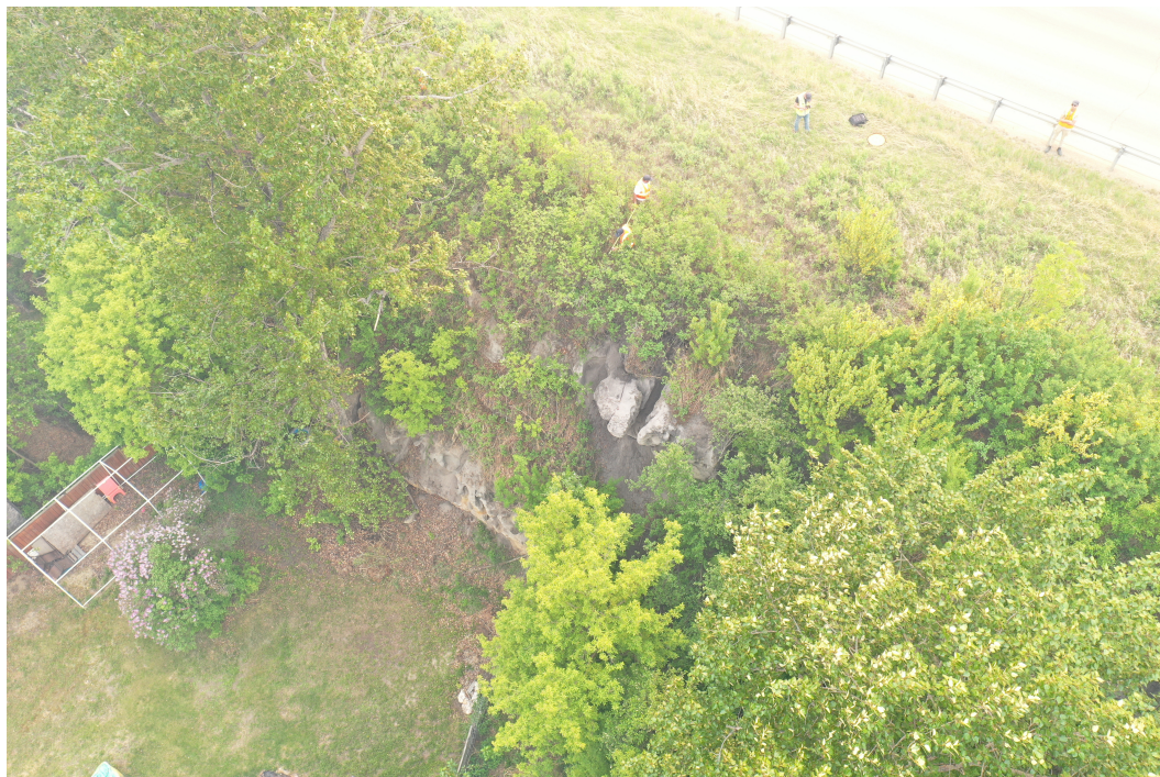
Photo 54-2. Closer view of steep eroded slope.
