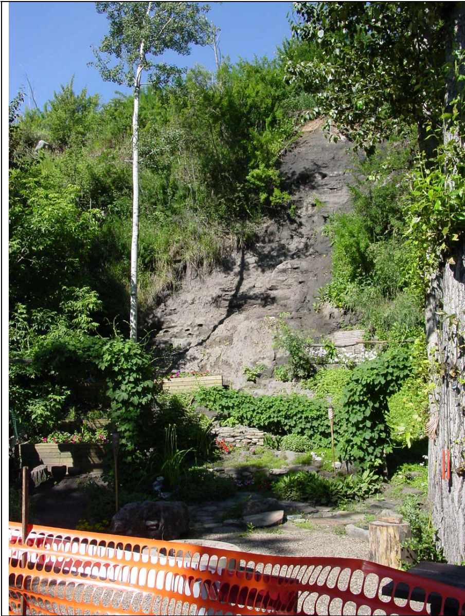
Photo 2. Slide to the south of the Cartier residence.
