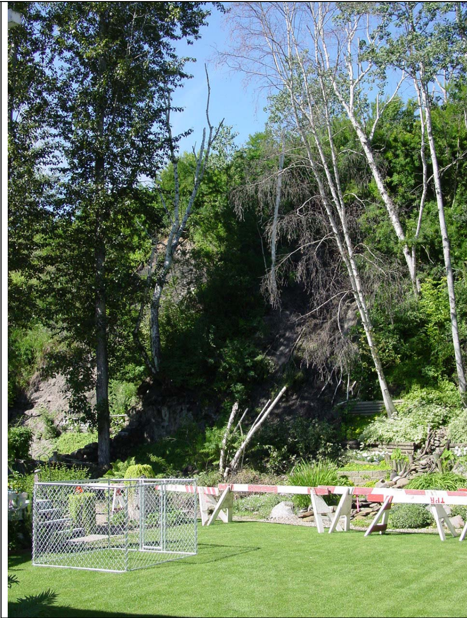
Photo 1. Cartier residence slide. Debris from the slope has entered the developed area below. Note some apparently dead trees on the slope.
