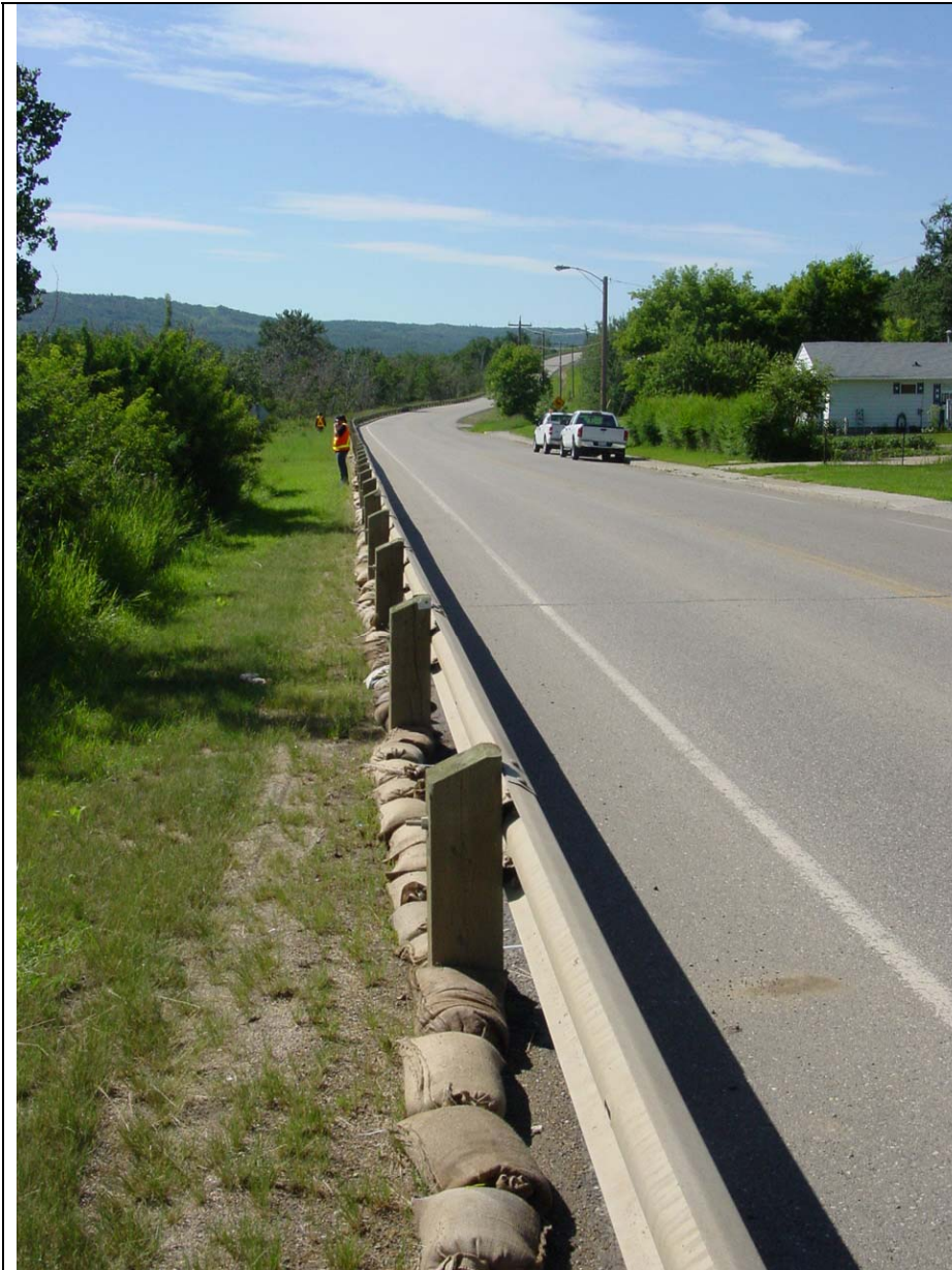
Photo 4. Highway upslope of the failure area. The edge of pavement is roughly 10 m away from the crest of the slope.
