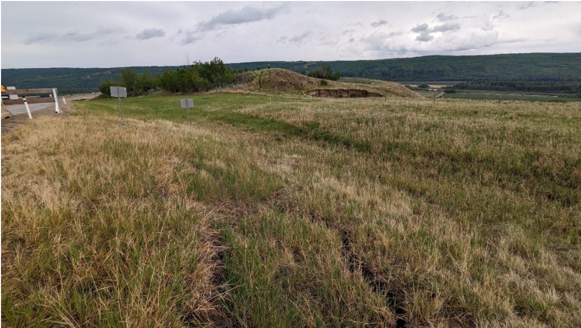
Photo 3: Looking southeast along the rest of the main tension crack at the highway sideslope.
