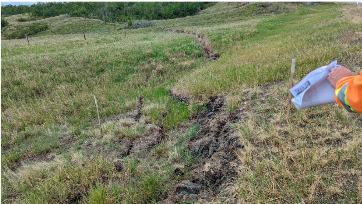
Photo 2: Looking southwest along main tension crack at the highway sideslope with measuring transect stakes in foreground.
