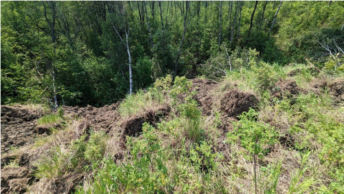
Photo 16: Crest of the toe of the slide.
