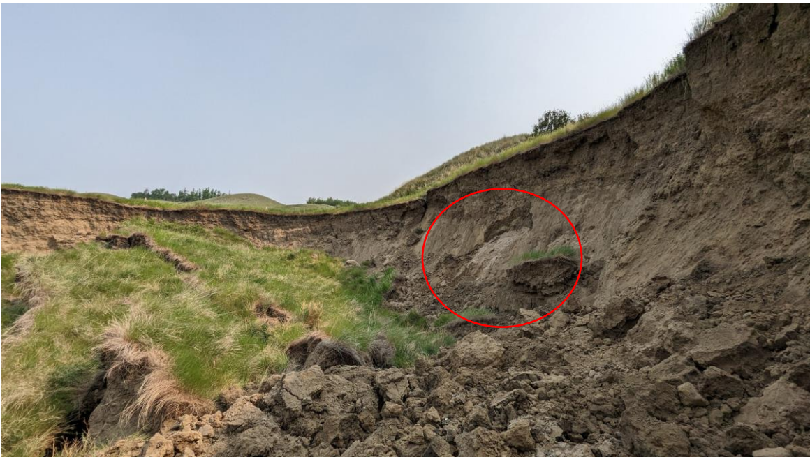
Photo 8: Looking north at the east flank of the main headscarp. Note large pocket (circled) of fine sand ravelling out of the face.
