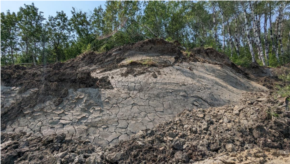
Photo 24: Looking southwest at a large portion of exposed, desiccated slip surface where drainage channel had been.
