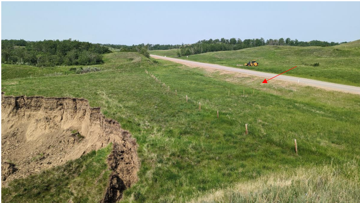
Photo 11: Looking west at the main crack forming in the highway sideslope.
