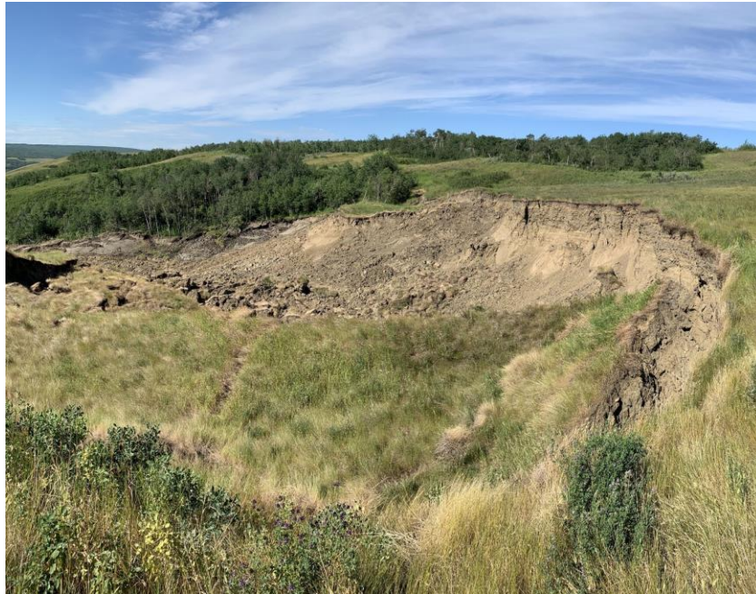
MCI Photo, June 29, 2023: Looking west at main headscarp which is mostly unchanged from the condition observed on June 9, 2023 (see Photo 10).
