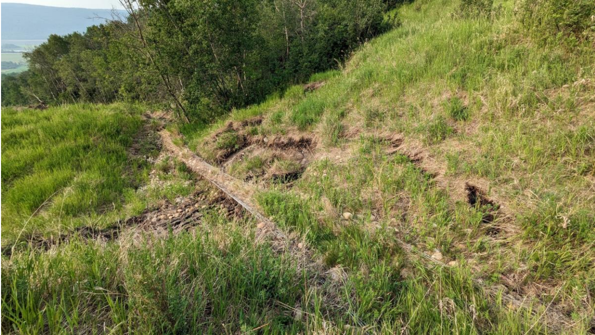
Photo 3: Looking south at stretched gabion mattress with west flank visible on the right side going into the trees.
