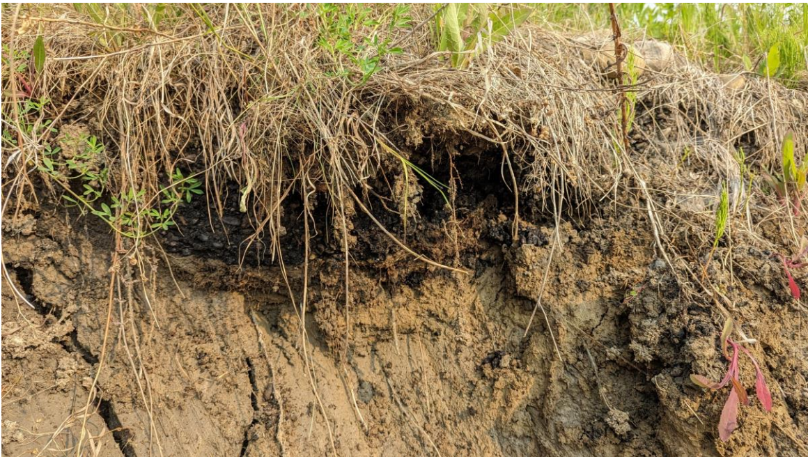
Photo 4: Seepage and asphalt exposed below drainage channel.
