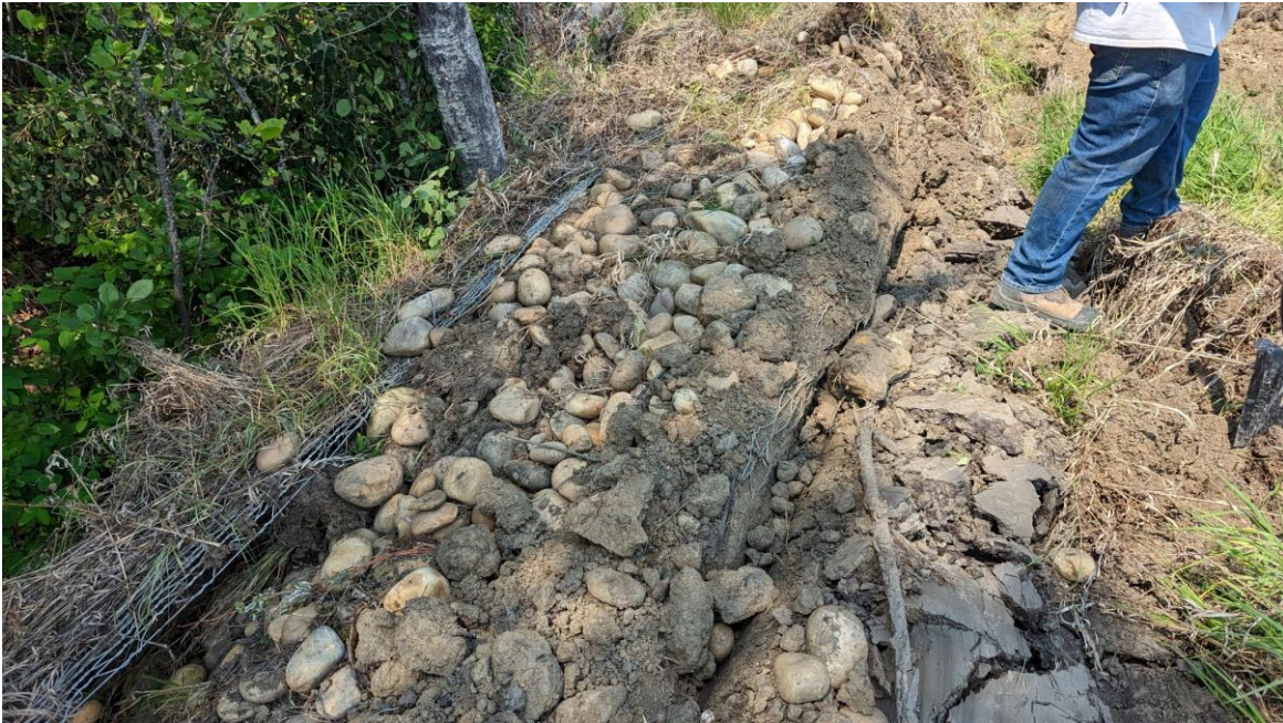
Photo 22: Distorted gabion mattress in the drainage channel. This suggests both that the drainage channel extended all the way to the bottom of the fill and that the lineal feature in Photo 21 could also have been gabion mattress being dragged.
