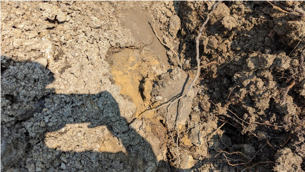
Photo 18: Wetter material down at the bottom of the toe.
