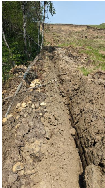
Photo 21: Looking north at possible secondary slip surface that cut through debris from an earlier phase of this slide. This groove ran for about 60 m on the west flank of the slide.
