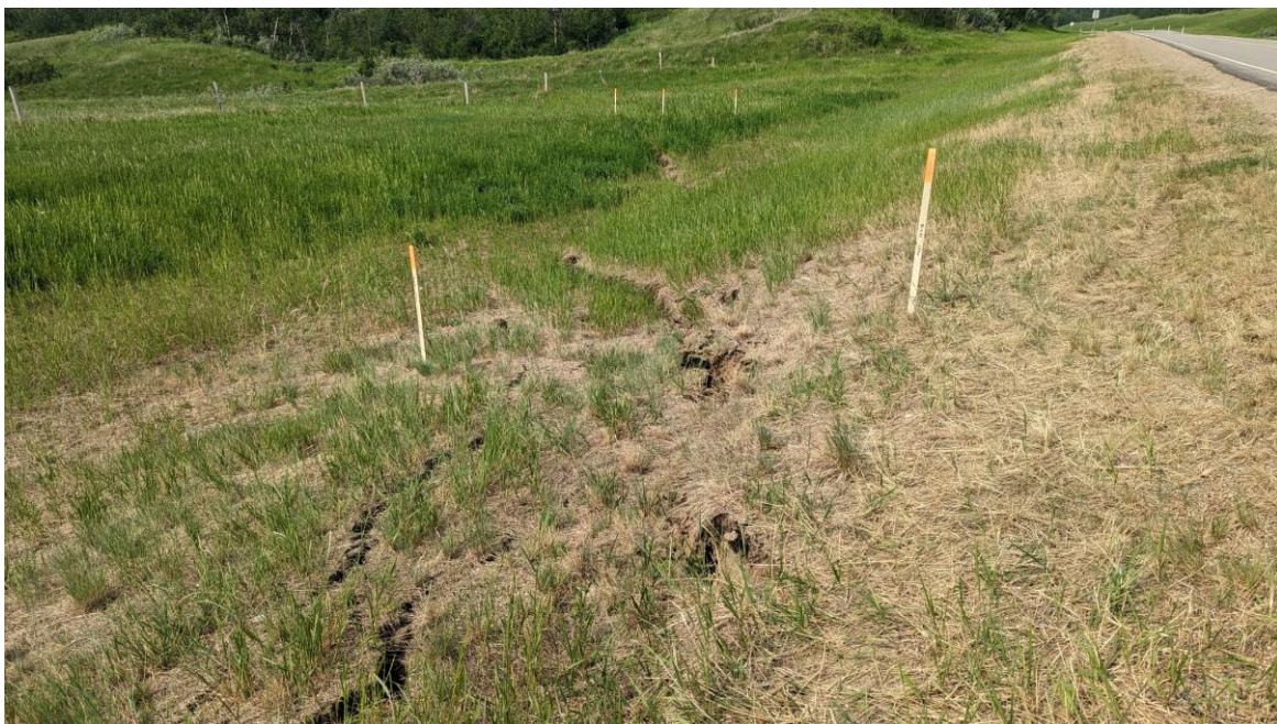
Photo 12: Looking southwest along the main crack in the highway sideslope. Line B stakes are in the foreground and Line A in the background. Measurements are made between the stakes.
