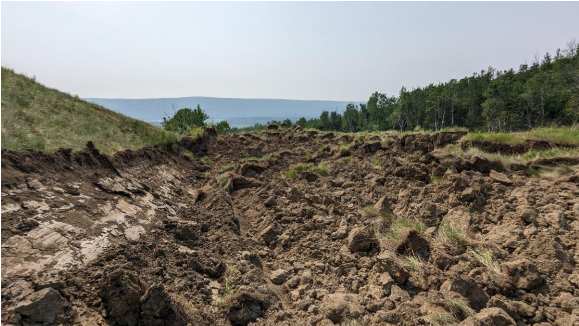
Photo 13: Looking south along east edge of the landslide body. The exposed slip surface on the left-hand side was desiccated.
