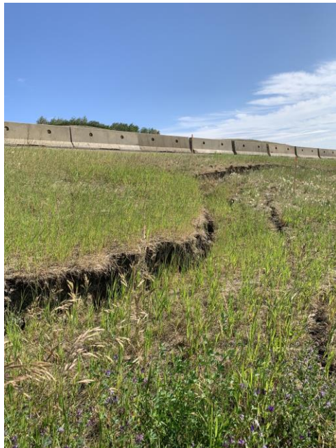
MCI Photo, June 29, 2023: Looking northeast at graben forming below tension crack in the highway sideslope.
