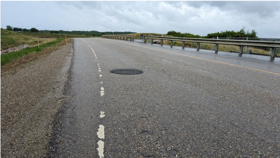
Photo 4 – Looking northwest at patched sinkhole in Hwy 2 off-ramp surface northwest of 99 Avenue intersection.
