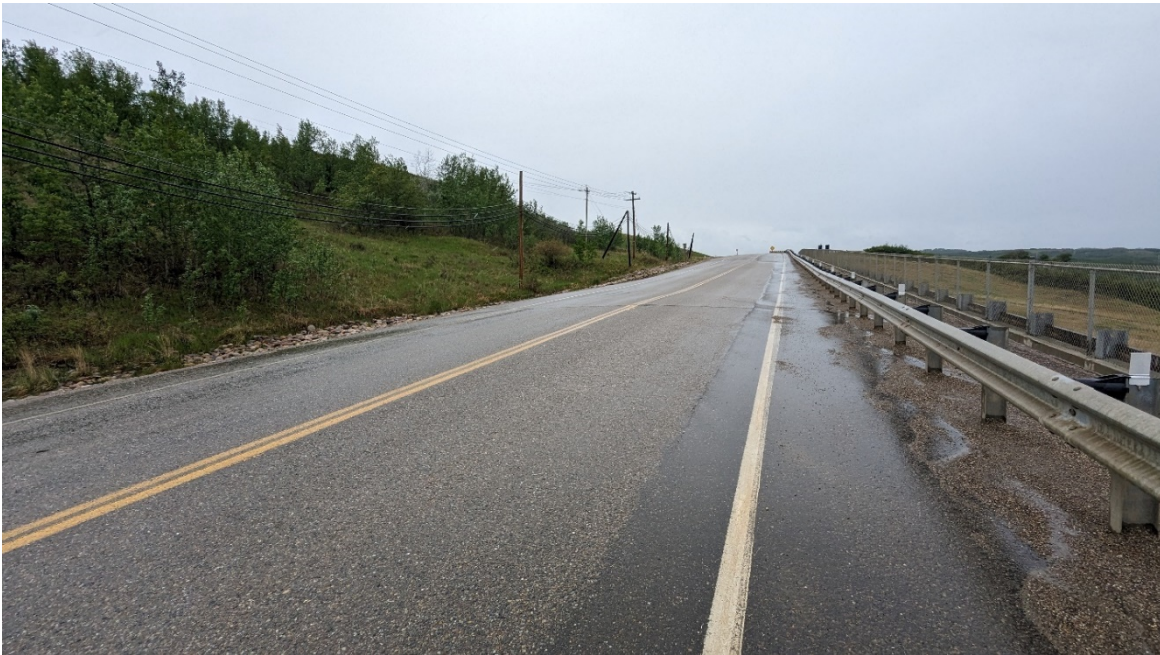
Photo 16: Looking northwest the dips in the roadway surface.
