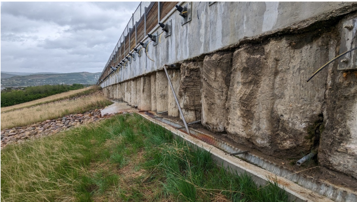
Photo 6: Accumulating rusty sediment from the existing subdrain flow. The pipe was flipped to flow the other way and some sediment blockage manually removed during the inspection.
