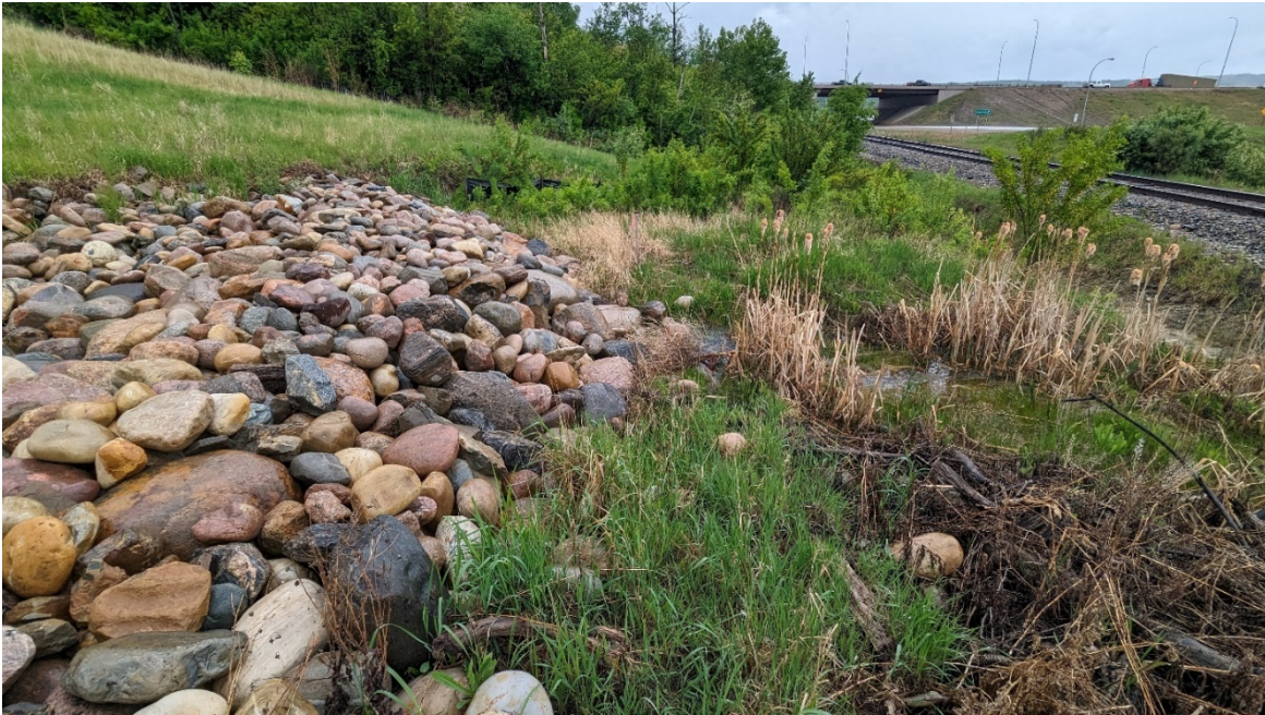
Photo 7: Looking north at bottom of the main riprap channel at the edge of the CN ROW.
