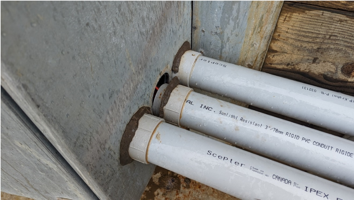
Photo 9: Thermal expansion/contraction may have detached this conduit from the side of the data enclosure.
