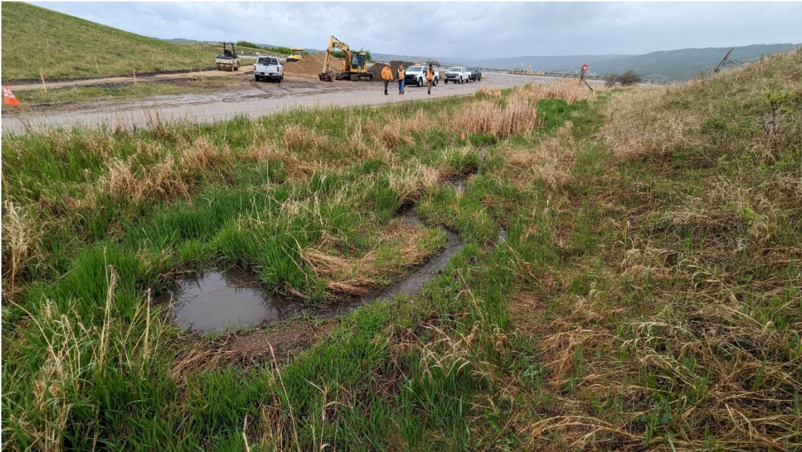
Photo 1: Looking north at spring along 99 Avenue and Town building new pedestrian pathway.
