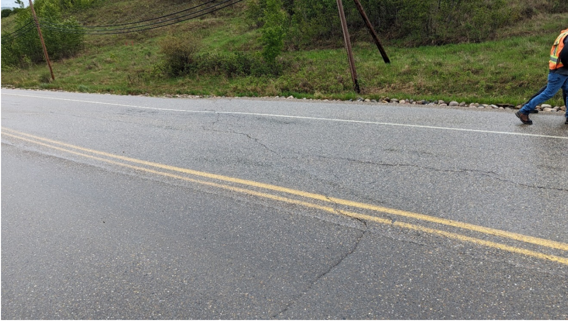
Photo 17: Looking south at the cracks coincident with the northwest flank of the deep-seated landslide.
