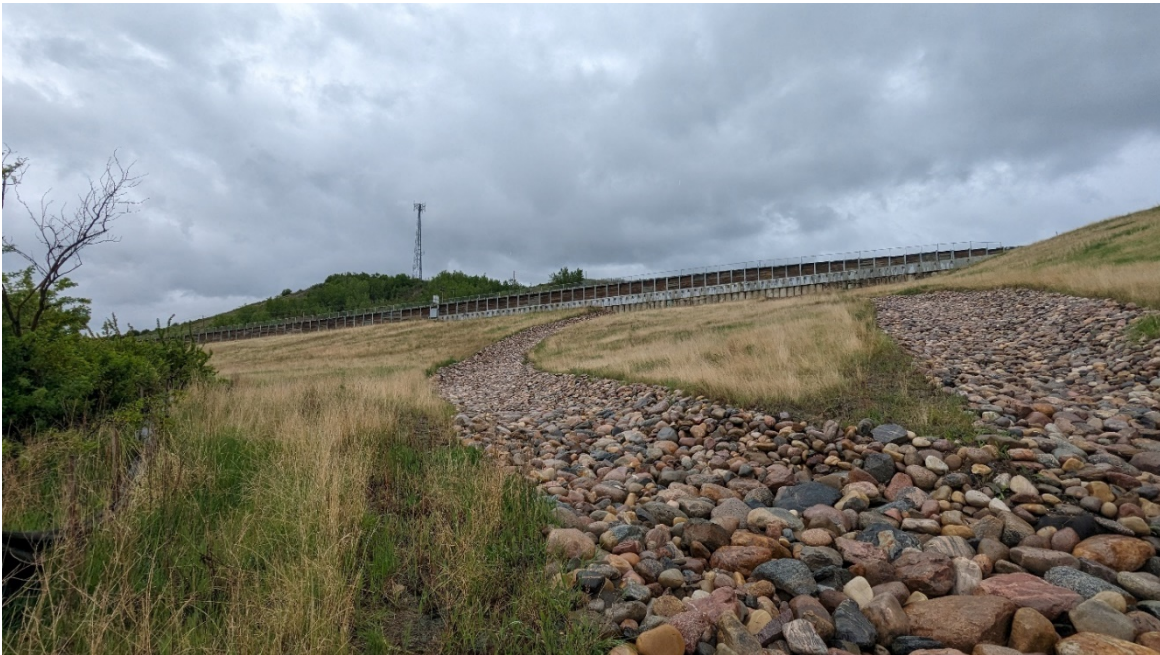
Photo 8: Looking southwest back up at the wall along the regraded slope and riprap drainage channels.
