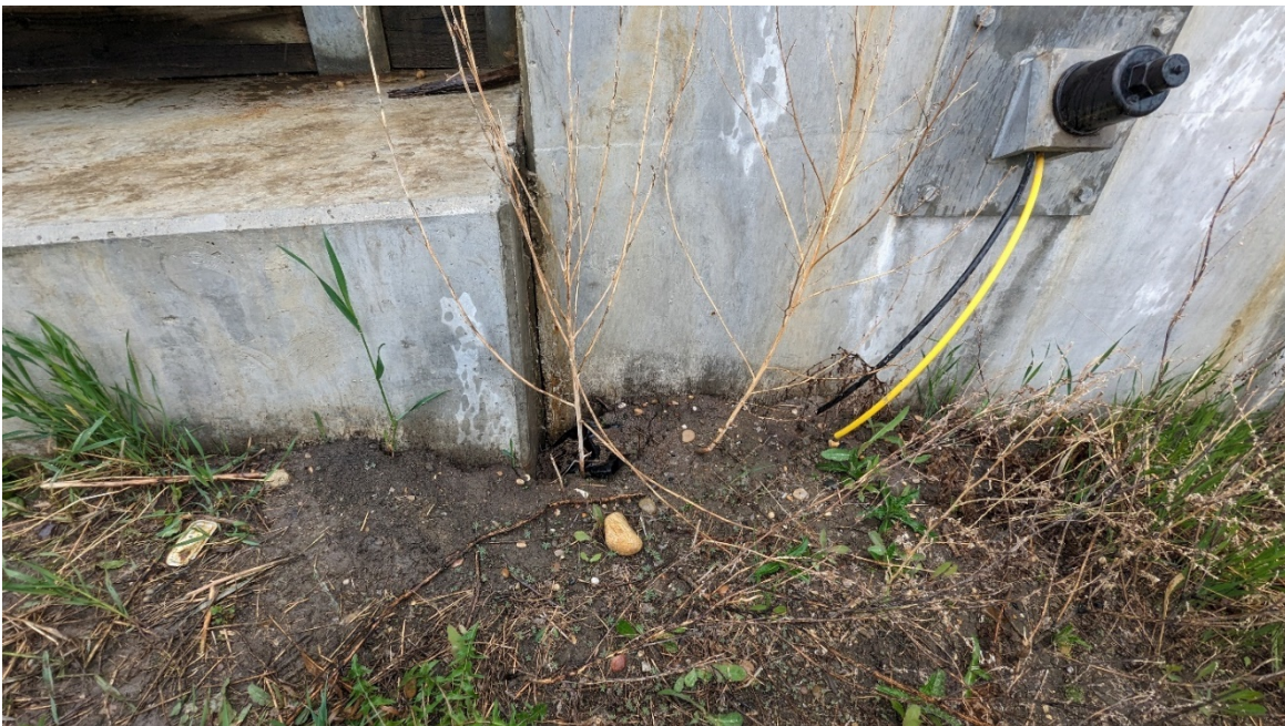
Photo 10: Small void or settlement at the junction between Wall Types 2 and 3.
