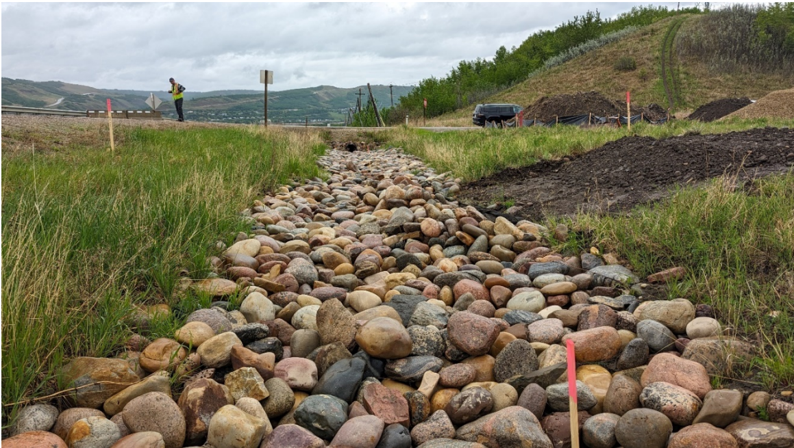
Photo 2: Looking southeast along grouted riprap in Hwy 2 off-ramp ditch at 99 Avenue culvert inlet
