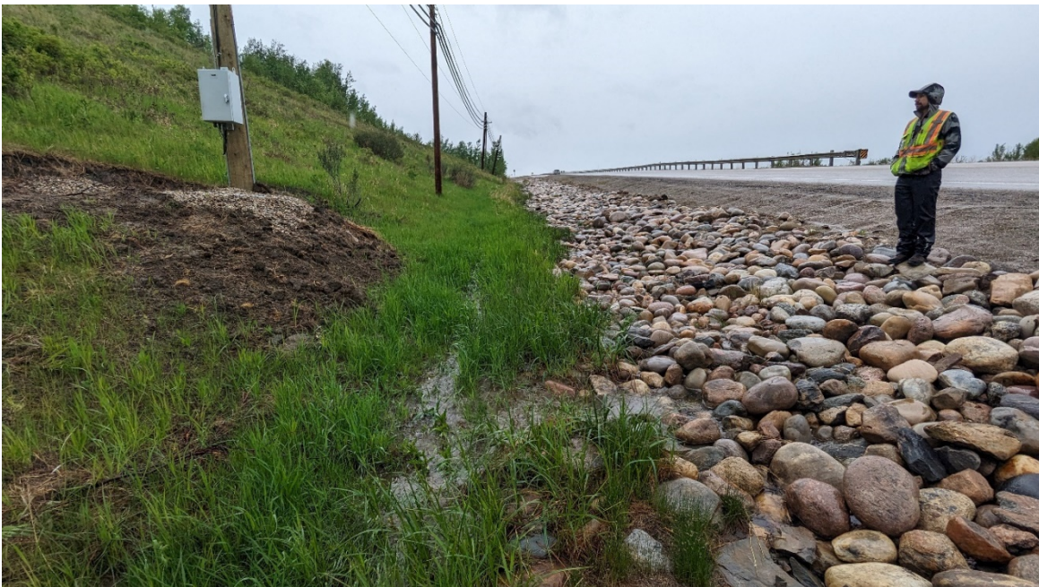
Photo 14: Looking northwest along the re-lined upslope ditch where recent construction activity disturbed the riprap diverting flow out of the channel.
