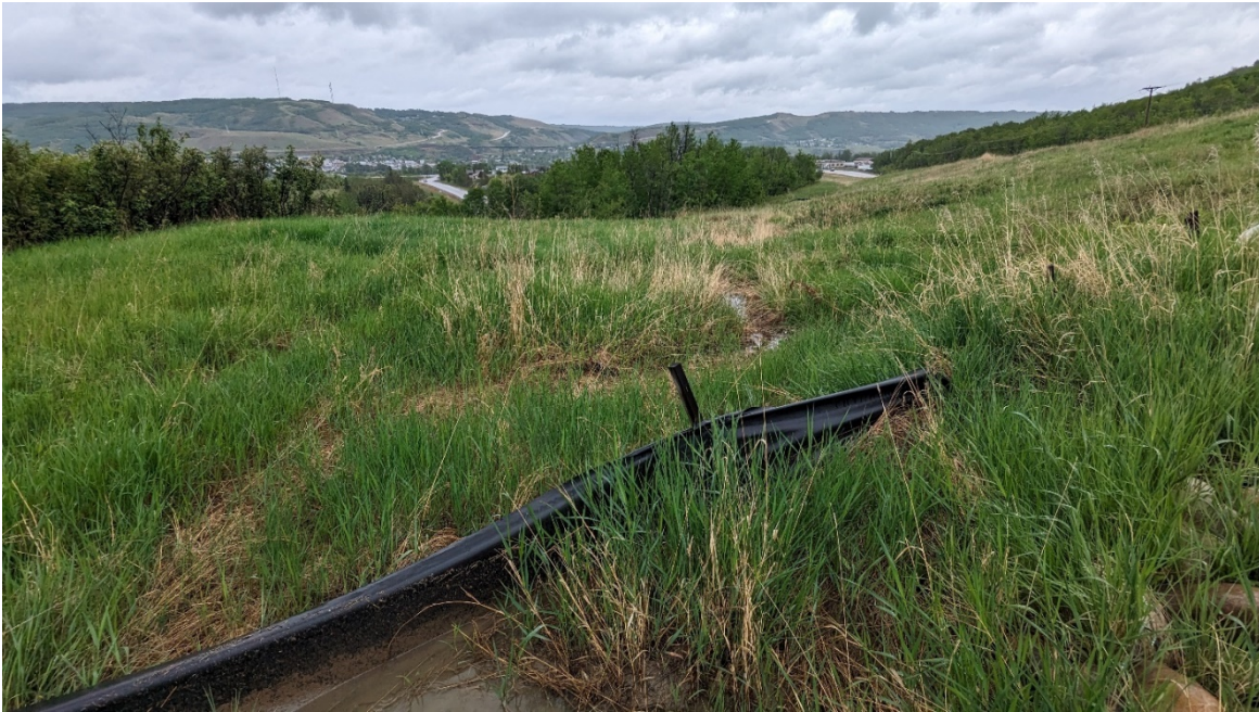
Photo 11: Looking southeast at the shallow gully forming beyond the silt fence at the end of the riprap dissipation bowl.
