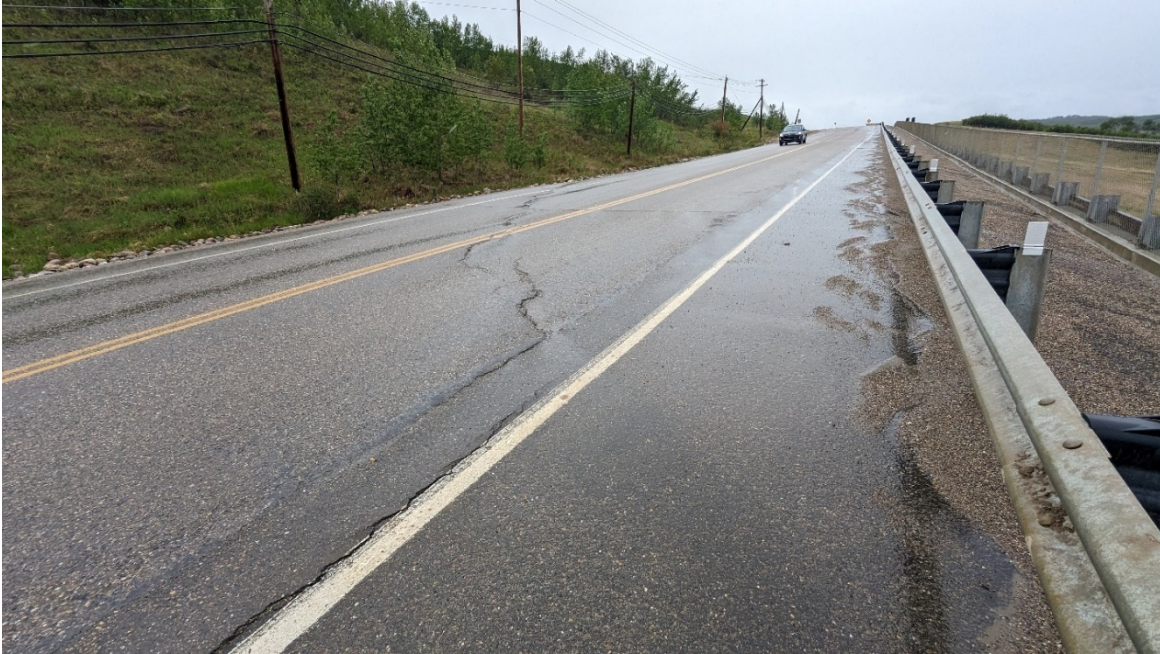
Photo 15: Looking west at the historical deep-seated crack location at the SE end of the pile wall.
